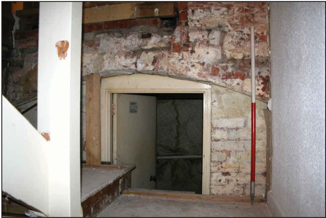
Photo. 1 The arched cellar opening in the rear wall of the basement, looking northwest. 1m scale.
