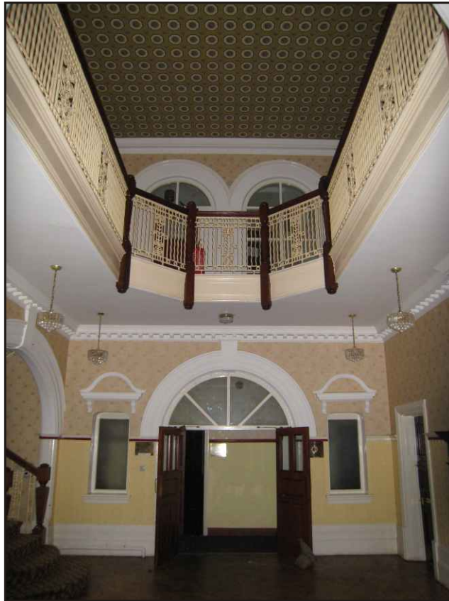
Photo. 3 The hall showing cornice with the gallery above photographed in 2007, looking east (Kathy Metcalfe, Exeter City Council).
