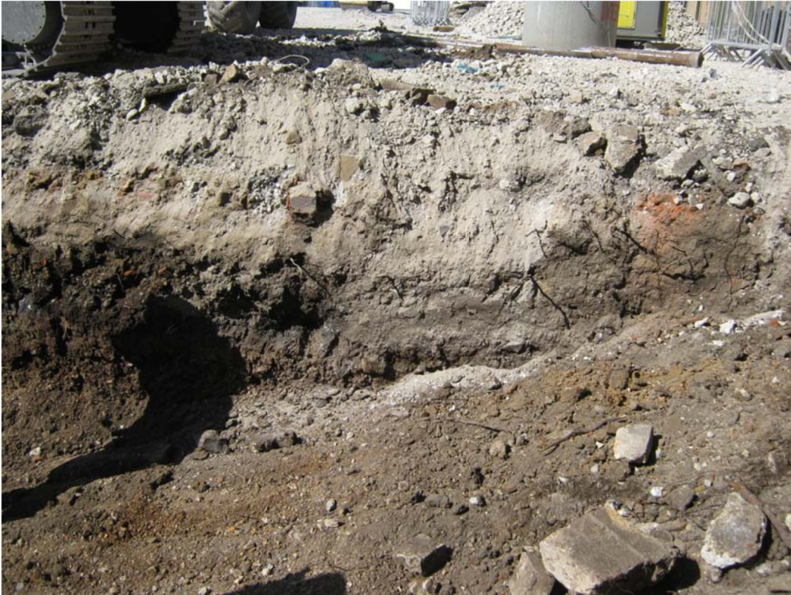
Plate 2: North-east facing section of western side of excavated area illustrating area of made ground (001)
