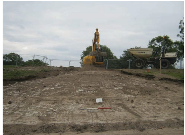
Machine reduction of package plant footprint
