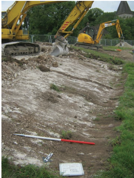
Machine reduction of package plant footprint
