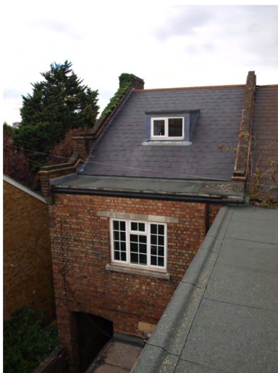
Plate 50: Block 3 – detail of the south elevation with entrance to through passage on the ground floor
