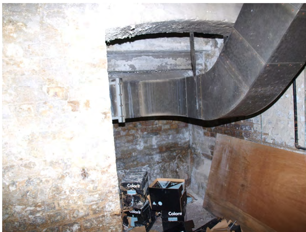
Plate 10: Phase 1 – Block 1 cellar, detail of archway in north-east room, supporting the stairs to the east front door of the block
