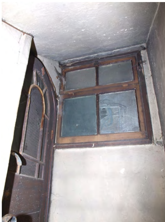
Plate 35: Phase 2 – Block 2a cellar (B3) with door and window detail. The window opened into the foyer for borrowed light
