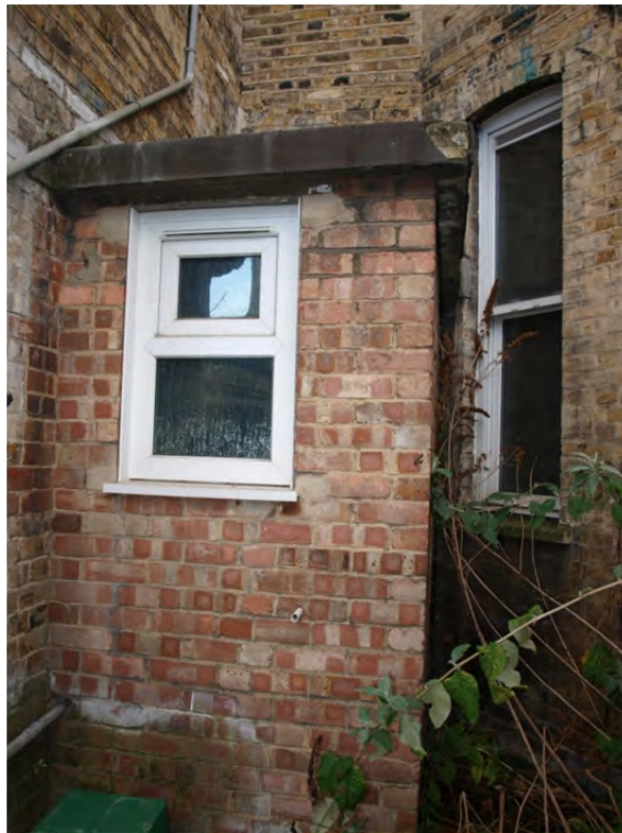
Plate 55: Phase 3 – Block 11, added WC facilities added to the exterior of Block 1e
