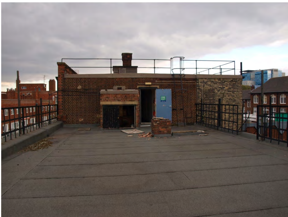
Plate 31: Block 2a – east end of the roof, shows contrasting brick detail of the hidden parts of the building in contrast to the principal elevation. Also shows blocked fire escape doorway
