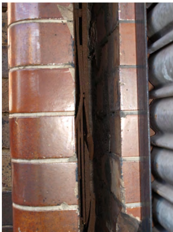
Plate 23: Phase 2 – Block 2a, the recess in the brickwork of the door jamb for the gate
