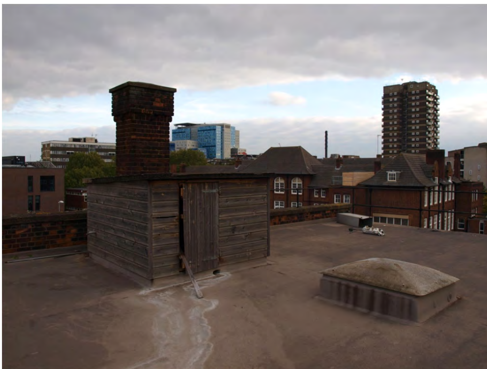
Plate 33: Phase 2 – Block 2a roof over the east tower with later shed built to house a water tank
