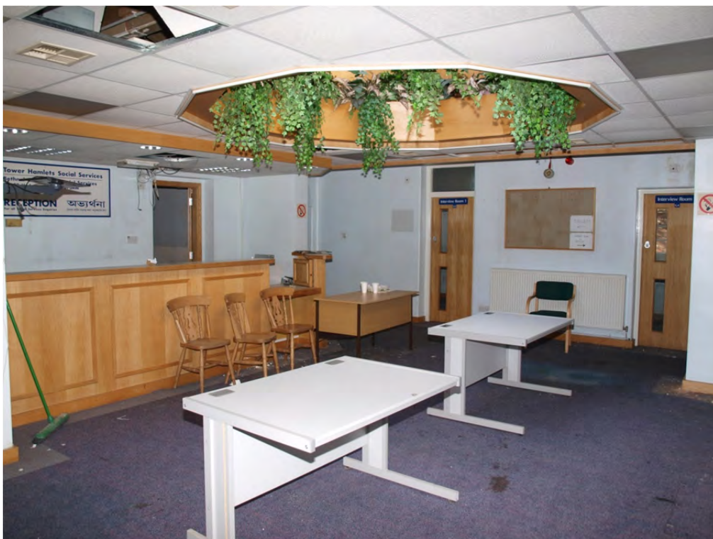
Plate 52: Phase 4 - Block 6, the interior of the large modern added single storey room with domed roof lantern
