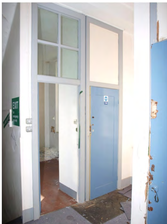
Plate 45: Phase 2 – Block 2b, the door to room F35 on the first floor. The cupboard and room doors share an architrave, the blank space at the top was a former upper cupboard
