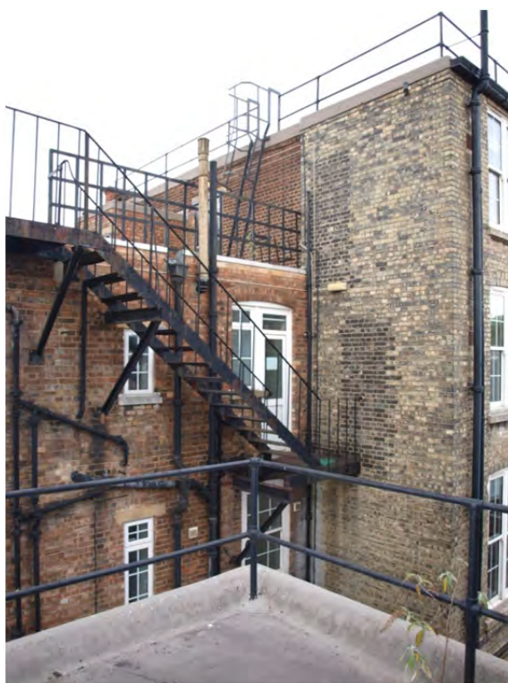
Plate 43: Phase 2 - Block 2a, the south side of main range and west side of east tower. Shows the blocked doors of the former fire-escape location next to the replacement.
