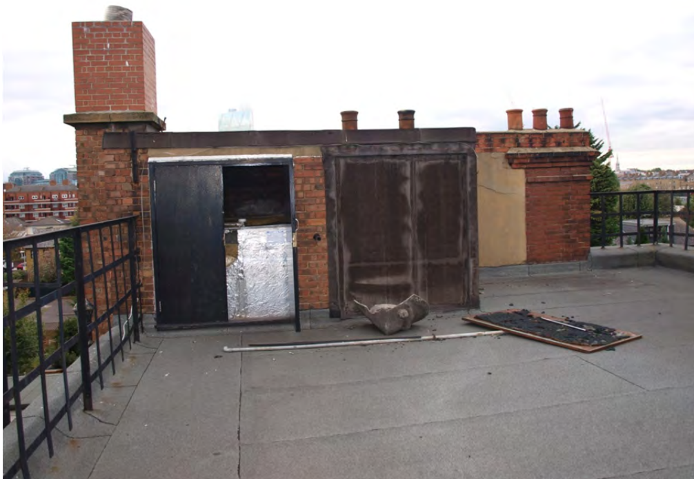
Plate 29: Block 2a, the small west end structure built to house a water tank on the Block 2a roof
