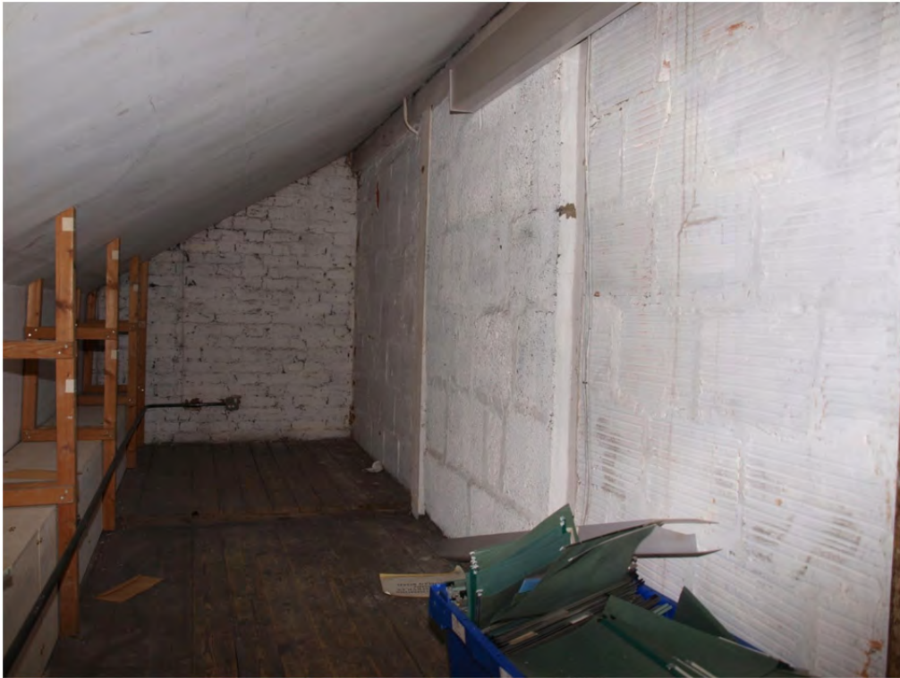
Plate 15: Phase 1 – Block 1a attics, south room, detail of breeze-block construction in north wall
