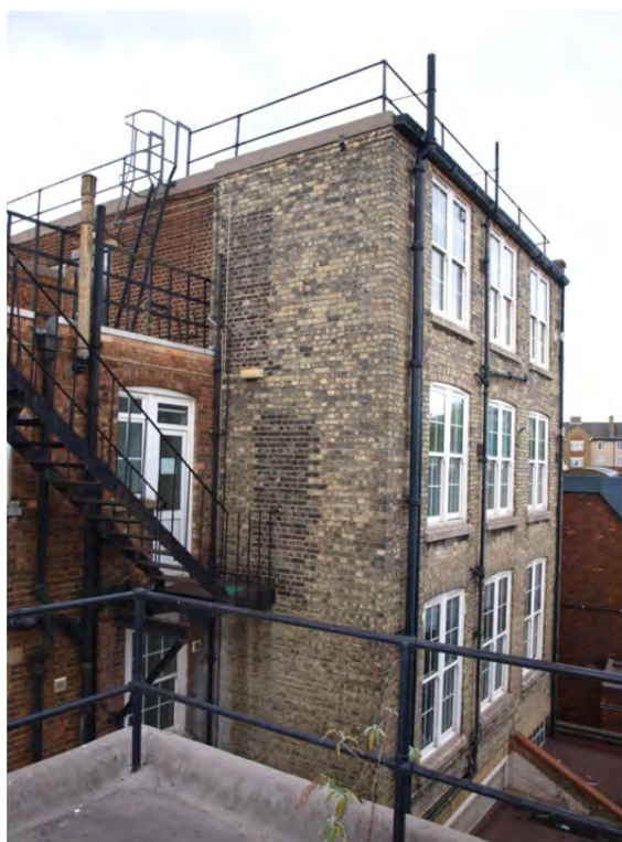
Plate 32: Phase 2 – Block 2a, the east tower with the single storey south structure just visible, showing white painted sloped side of former light well
