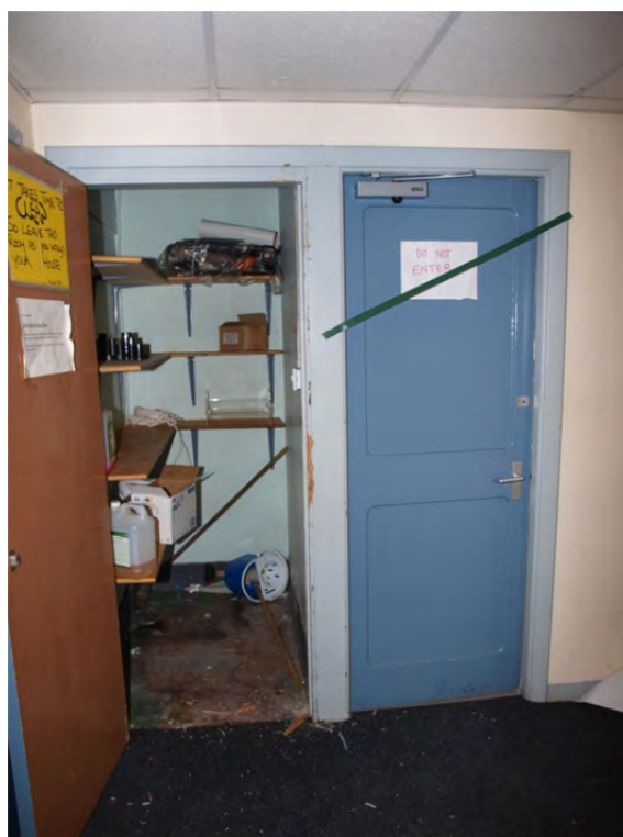
Plate 14: Phase 1 – Block 1a first floor, WC and cupboard detail to east of F13
