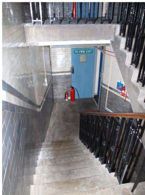
Plate 38: Phase 2 – Block 2a, detail of the tiled interior of the stair tower with principal staircase
