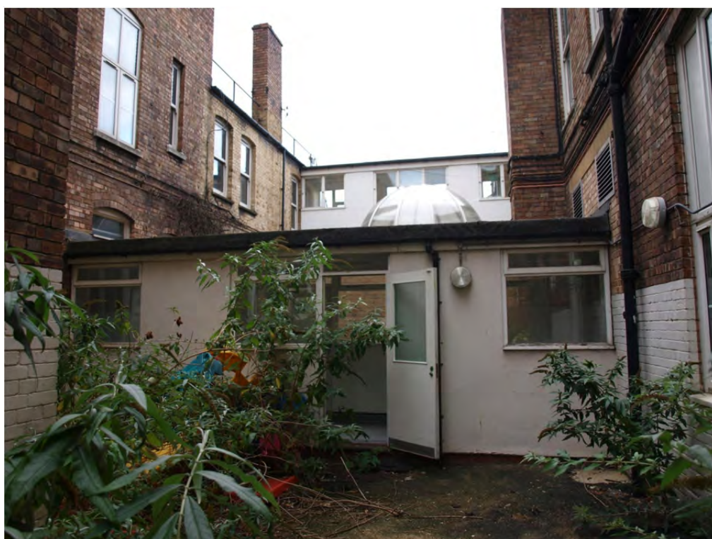
Plate 53: External view from open area 3, looking west: Block 7 link, domed roof lantern of Block 6, modern first floor extension to corridor 1b and the inner elevations of Blocks 2a, 2b, 1a and 1e
