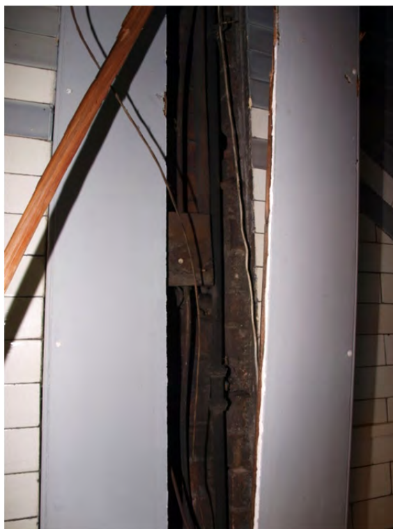
Plate 39: Phase 2 – Block 2a, detail of the integral recess to house pipe-work within the tiled walls of the stair tower
