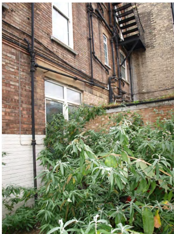
Plate 27: Phase 2 with modifications, part of the south side of Block 2a, with the late 20th century link addition (Block 8)
