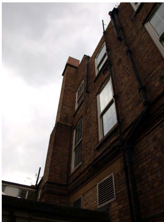
Plate 28: Phase 2 – Block 2a, the south elevation with externally projecting stack, rebuilt at the top
