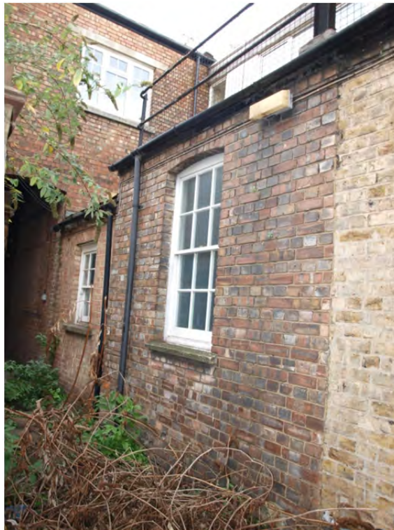
Plate 51: Phases 1, 3 and 4, the west elevations showing the different fabric of the phased construction
