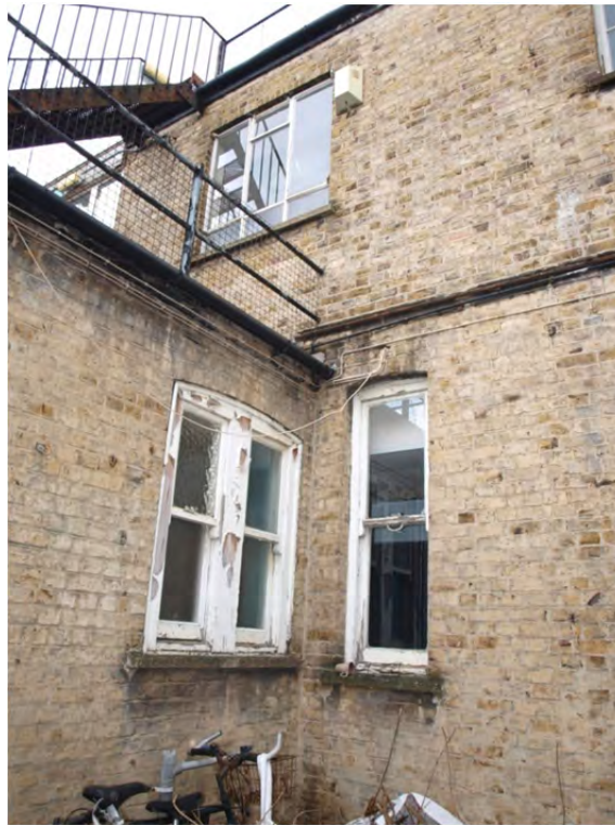
Plate 21: Phase 1 - Junction of Blocks 1c and 1d with straight joint between them
