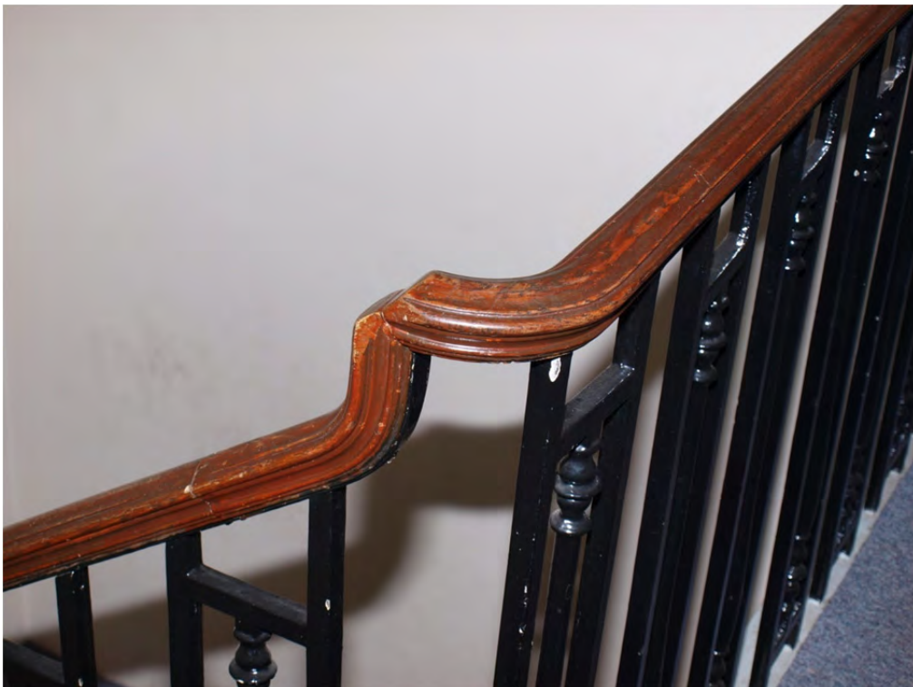
Plate 16: Phase 1 – Block 1a staircase with awkward ramp junction on the handrail
