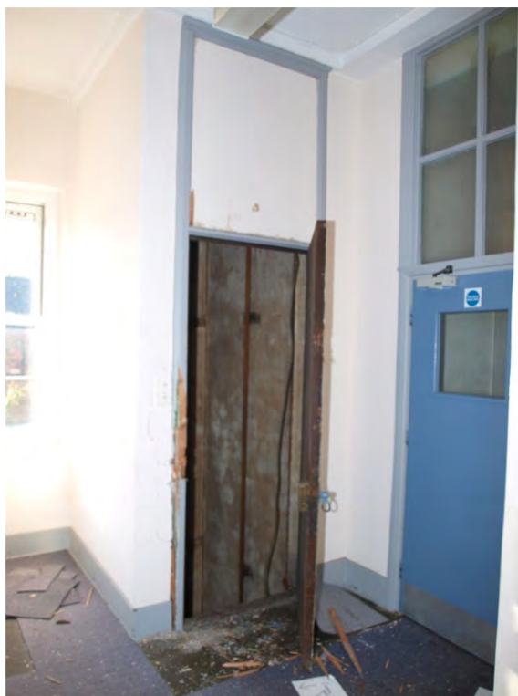
Plate 44: Phase 2 – Block 2b – the remains of the lift shaft within the east arm of the block
