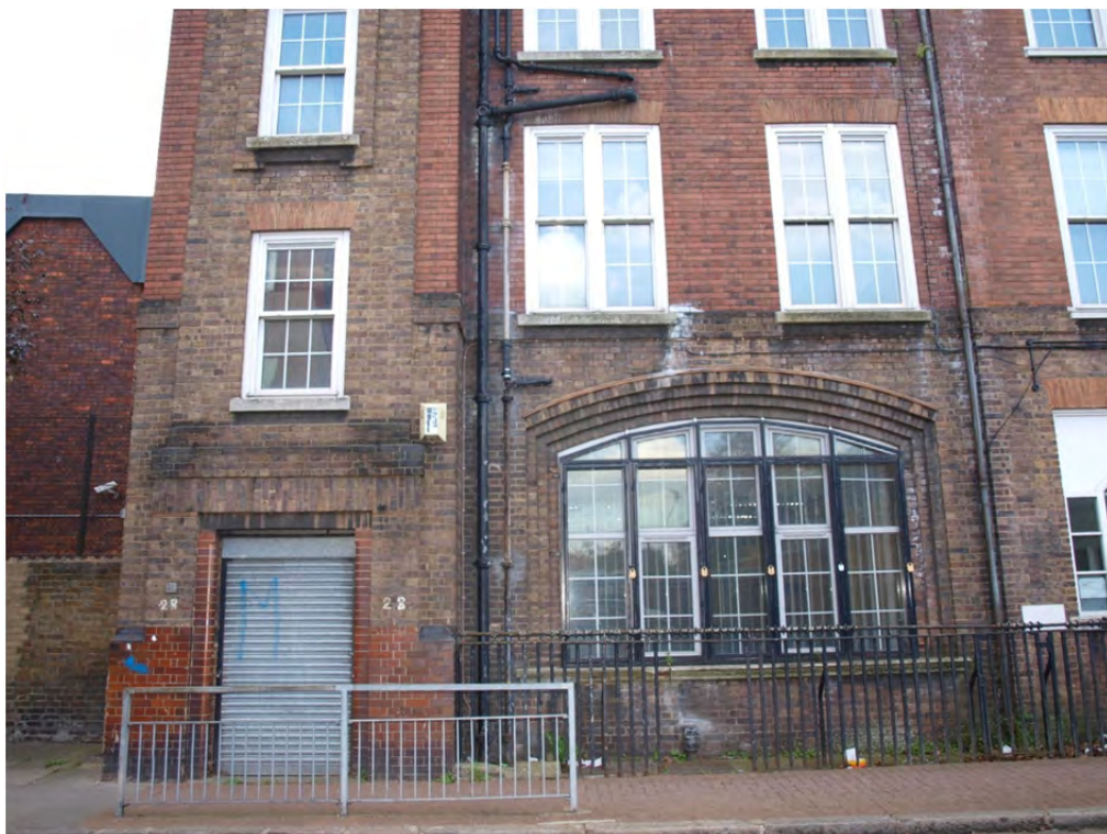
Plate 22: Phase 1 – Block 2a, the east end with stair tower, windows at half-storey intervals on the north elevation
