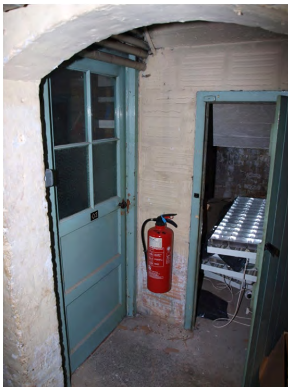
Plate 9: Phase 1 - Block 1 cellar – southwest detail of inserted doors to create lobby and under-stairs cupboard
