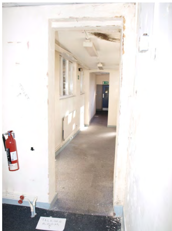
Plate 17: Modern first floor extension to Block 1b corridor – viewed from rear of Block 1a
