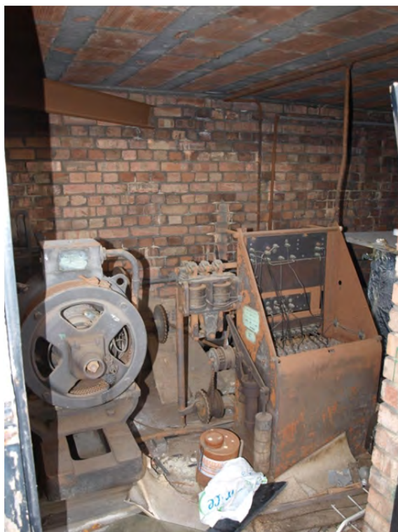
Plate 47: Phase 2 – Block 2b, interior of the roof part of the lift shaft with the mechanism retained
