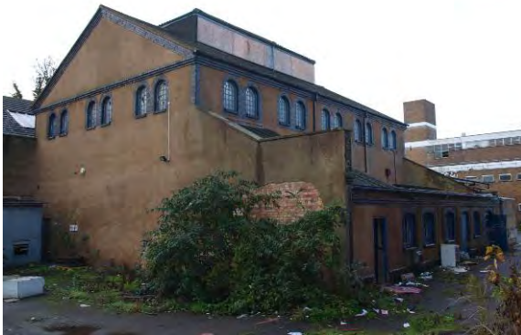
Exterior view of the locally-listed part of the present building (Block A) facing south
