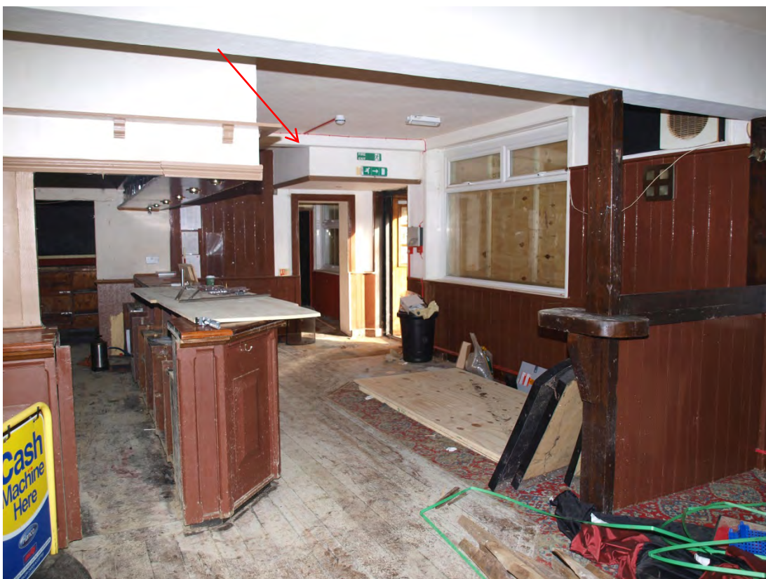
Plate 6: Main bar area within southern end of principal range, looking north-east. Boxing in ceiling marking possible original northern extent of building highlighted (20)
