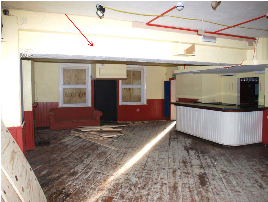
Plate 11: Northern bar area, looking south-east. Line of rear wall of principal range highlighted (17)
