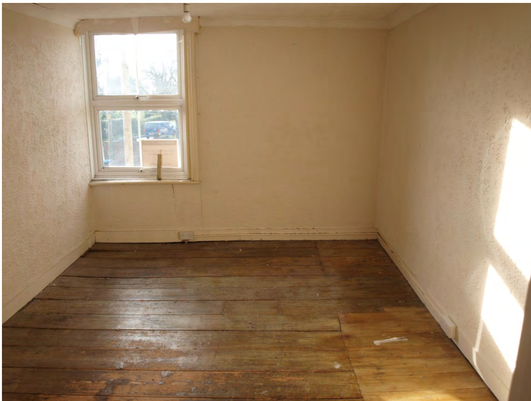
Plate 16: Rear first floor room within southern end of principal range, showing location of earlier chimney-stack preserved within floor-boards, looking south (40)
