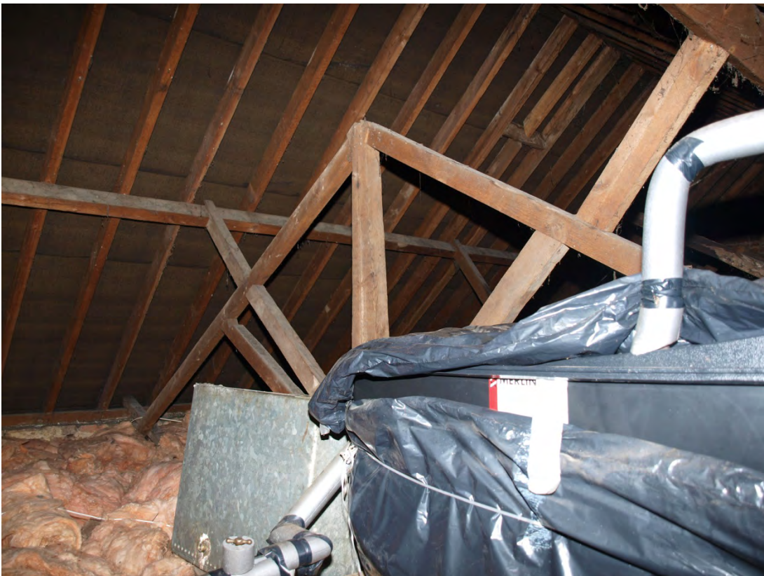
Plate 20: Earlier roof truss preserved within southern end of the roof, looking south-east (55)
