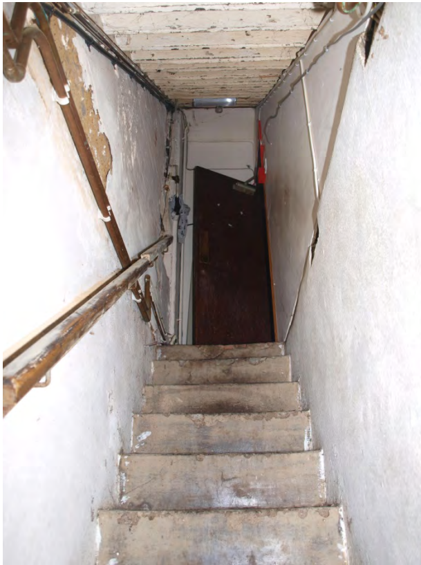
Plate 9: Cellar steps with redundant staircase to first floor visible above, looking north (32)
