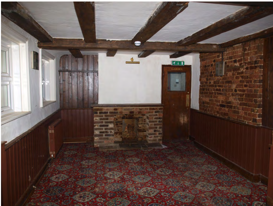
Plate 10: 19 th century addition, now forming part of main bar area, looking west (10)
