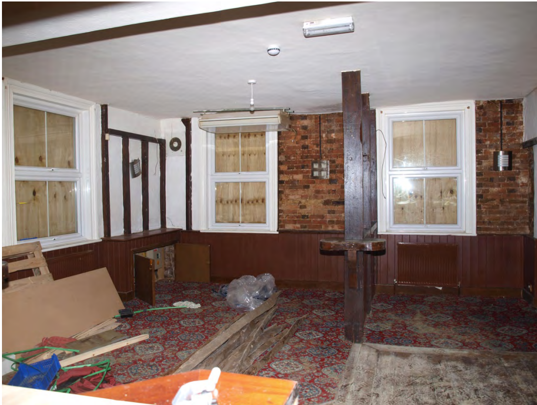
Plate 7: Main bar area within southern end of principal range: brickwork of south wall, looking south (21)
