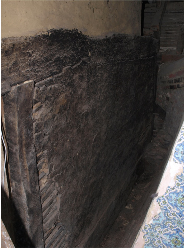
Plate 3: The north facing side of the soot encrusted smoke-bay truss partition of the Phase 1 building (wall-papered part of inserted stack just visible)
