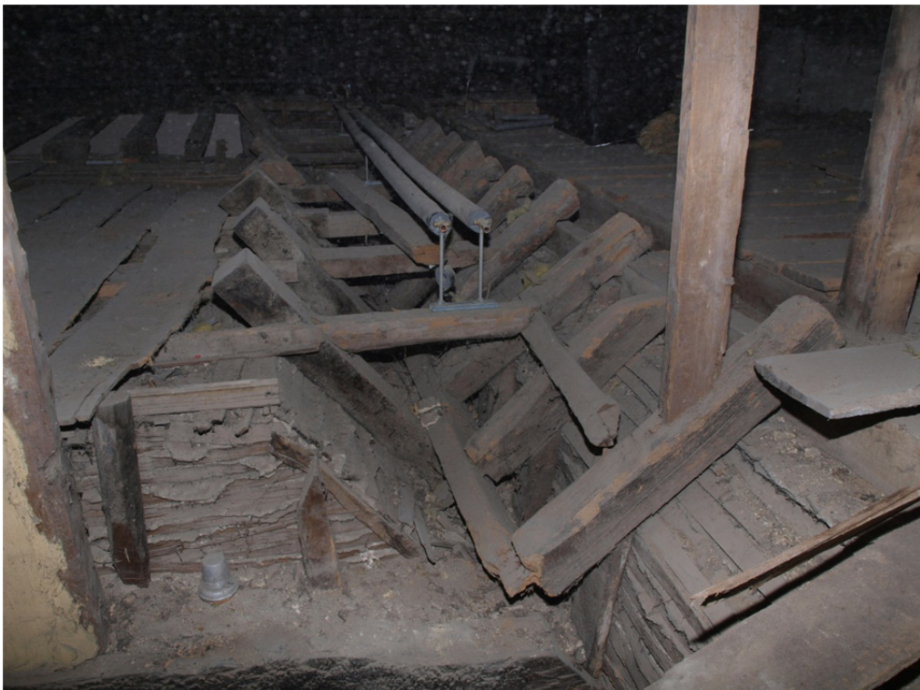
Plate 4: View towards the south of the Phase 1 roof over the Hall with the 18 th C roof supported on a plate over the backs of the original rafters creating an M-profile roof (Truncated in the 19 th C)
