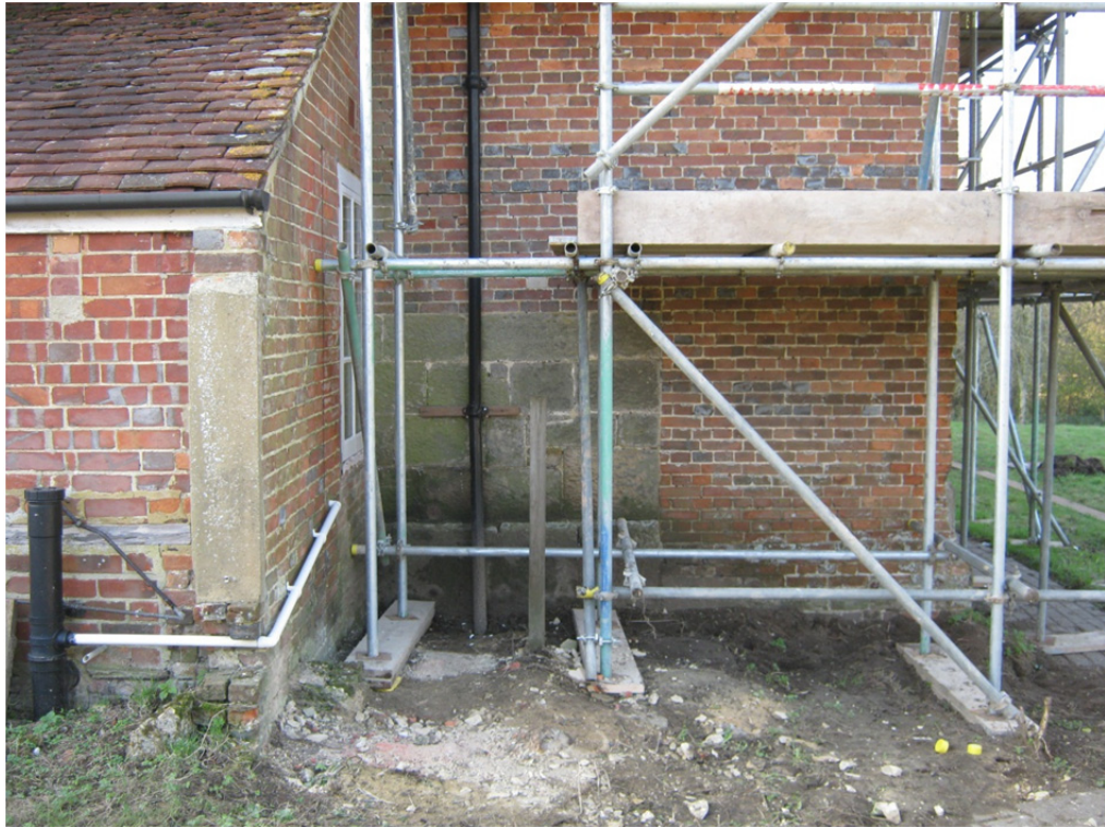
Plate 1: North end elevation with remnant c. 17 th century masonry of the added lean-to outshot
