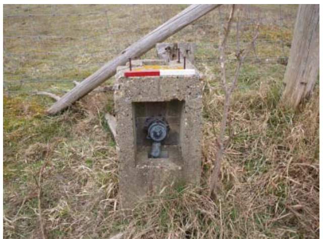
Concrete post at 200 yard position, showing telephone connection
