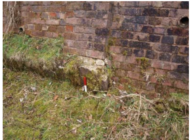
Low concrete step in south retaining wall
