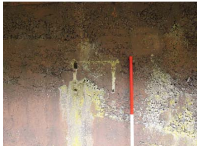
Location of main telephone shelf on markers' gallery wall
