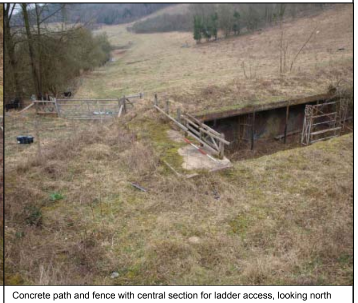
Concrete path and fence with central section for ladder access, looking north
