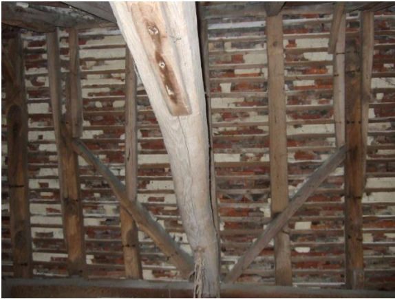
Plate 70: The Oast – indications of the location of the Period B cowl, removed. Staining indicates thatch cover before and after cowl insertion
