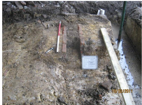
Plate 65: The Barn Watching Brief– probable drain cut into the subsoil of the eastern end bay of the barn
