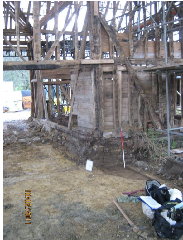
Plate 63: The Barn Watching Brief – brick platform in rear extension abutting Period A rear barn wall
