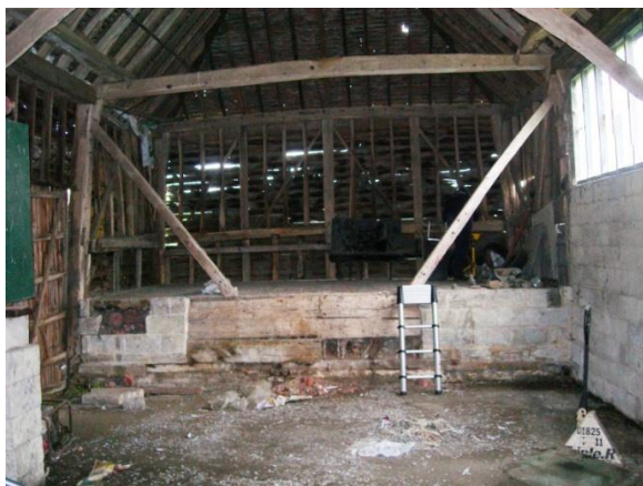
Plate 7: Steddenden Barn – detail of truss with raking shores and remnant of timber partitioning
