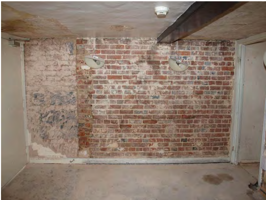
Plate 16: Rear wall of Unit 1 showing blocked inserted doorway, viewed from Room G.03, looking south-west
