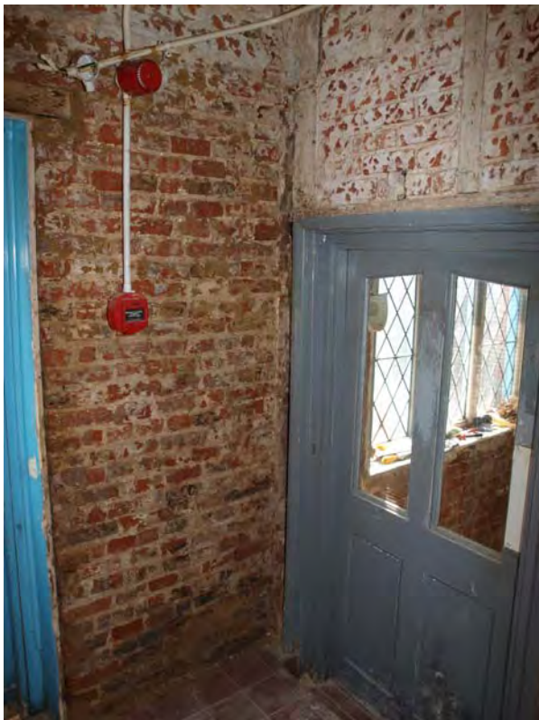
Plate 22: Straight joint within the brickwork at the junction of Units 2 and 3, view from Room G.05, looking south
