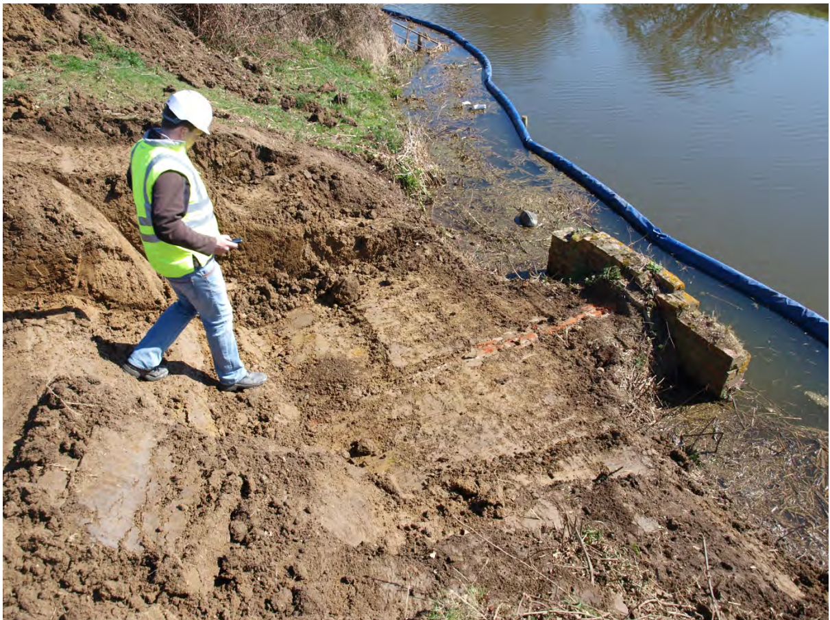
Plate 2: Stage 1 of the excavations which included the removal of the head-wall, looking east
