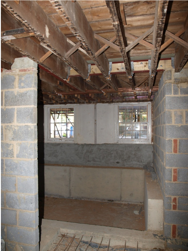
Plate 3: Cross-strutted ceiling over ground floor of Period D western range, looking north
