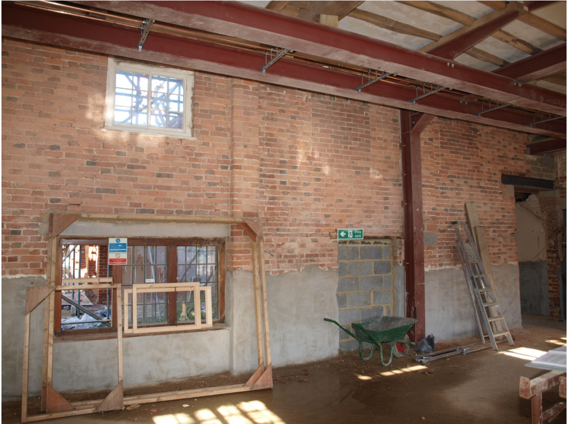
Plate 1: Two blocked window apertures at first floor level in Period B range, looking north-west
