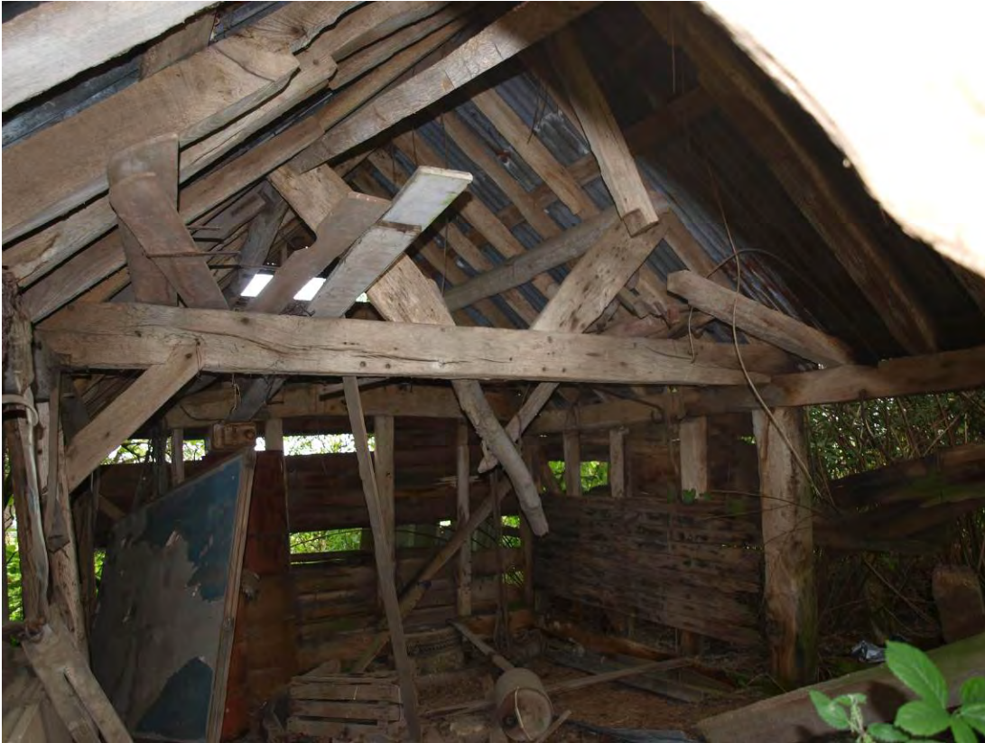
Plate 15: Interior of the smaller of the two buildings at Hares Hill Farm, looking west
