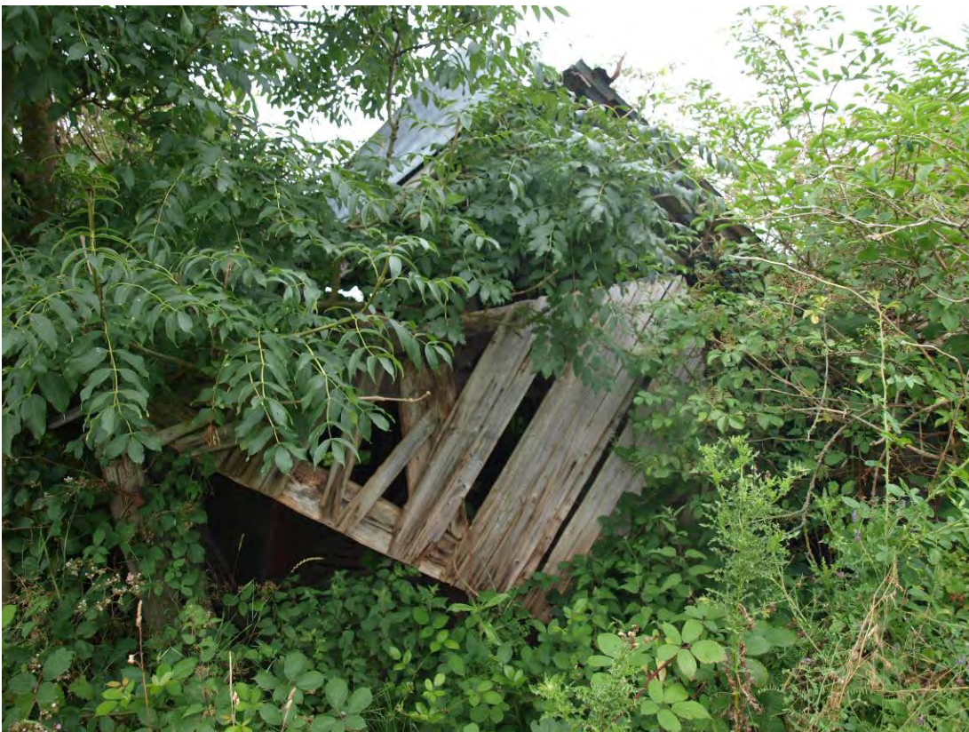
Plate 14: The smaller of the two buildings at Hares Hill Farm, looking west
