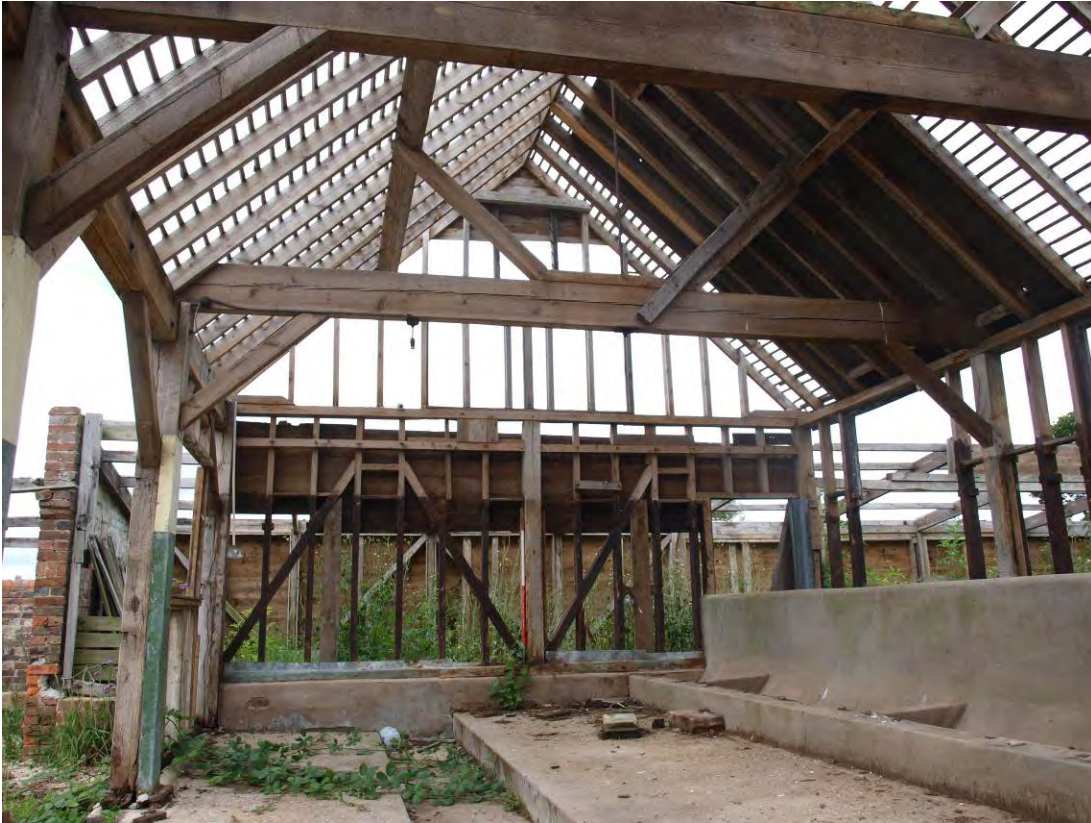
Plate 11: Interior of Building 2, showing west end wall and roof construction, looking west
