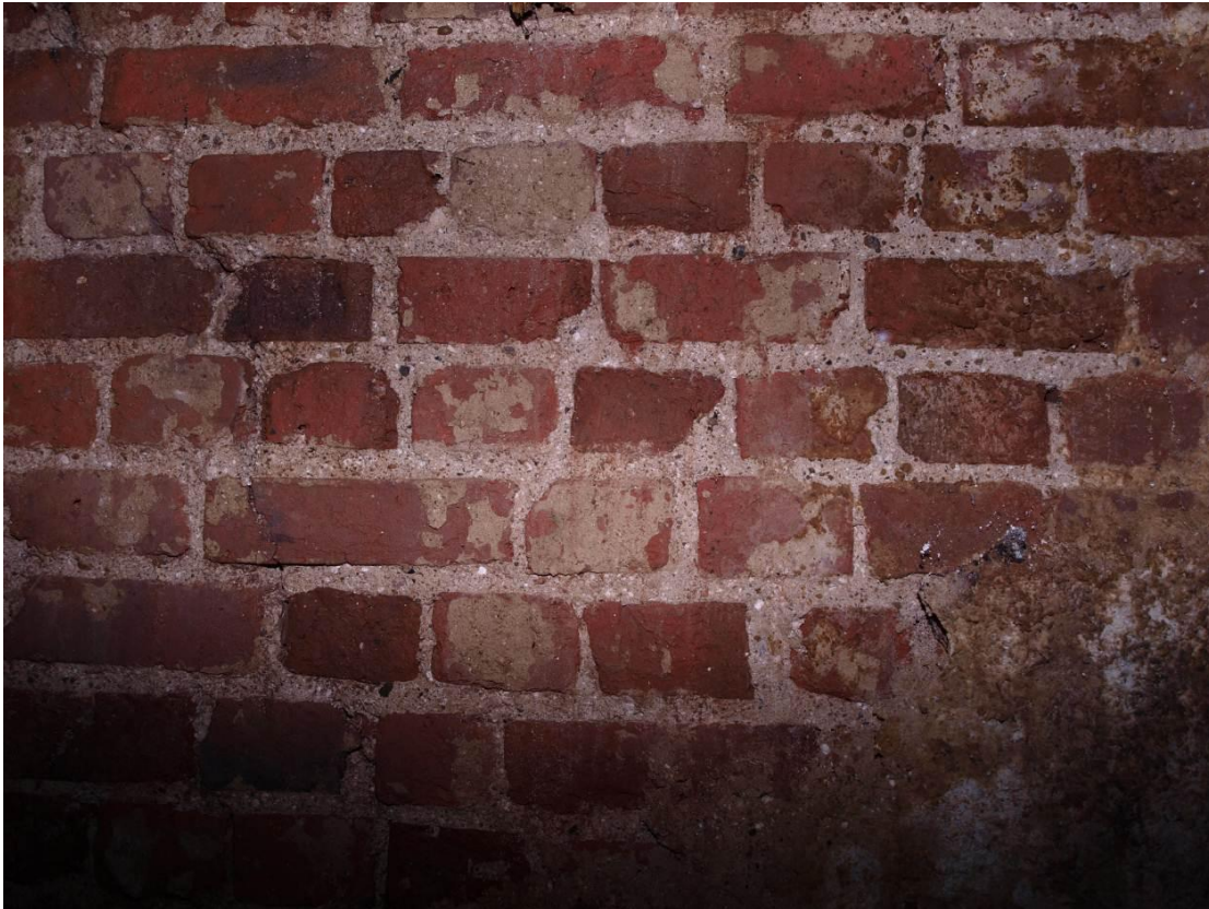
Plate 9: Late-18 th /early-19 th century brickwork to west wall of Room 2, looking west (20)
