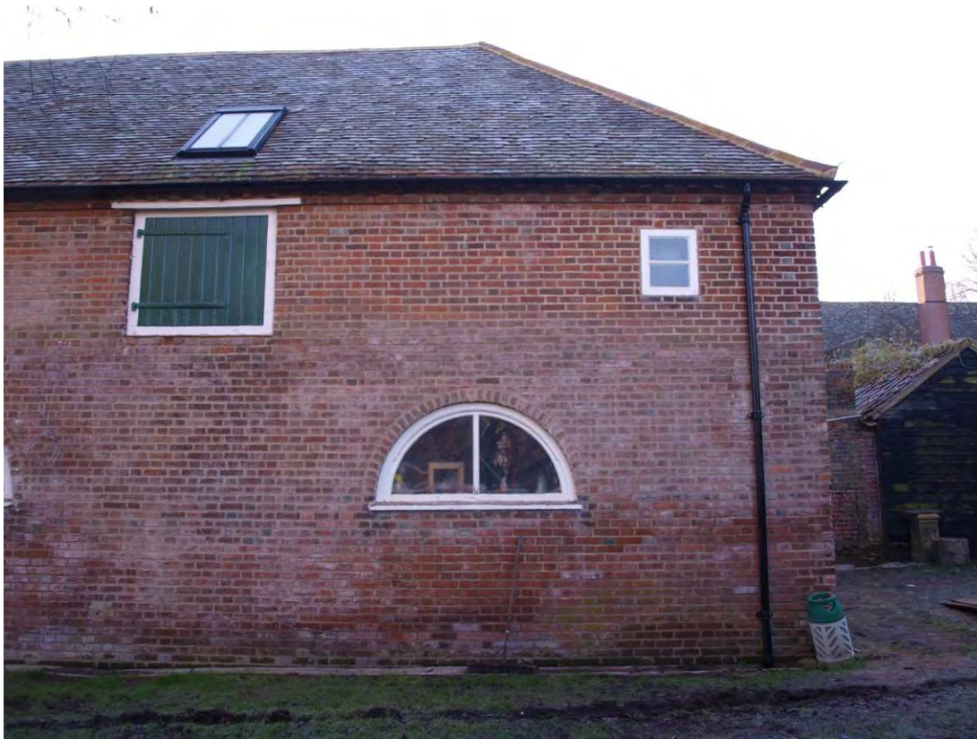
Plate 3: High-set loading doorway and small inserted window on north elevation, looking south (3)
