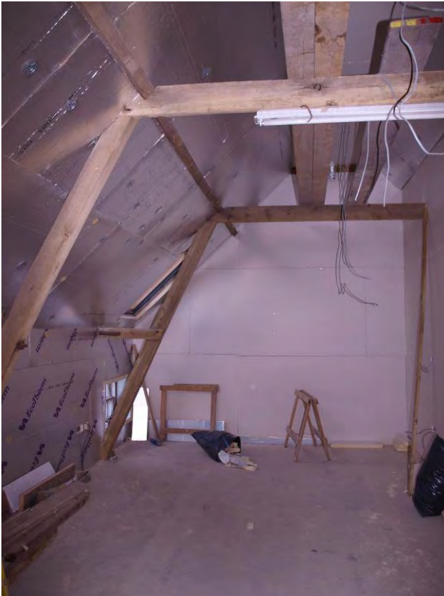
Plate 23: Interrupted tie-beam roof truss (truss in foreground is a later insertion), looking west (49)
