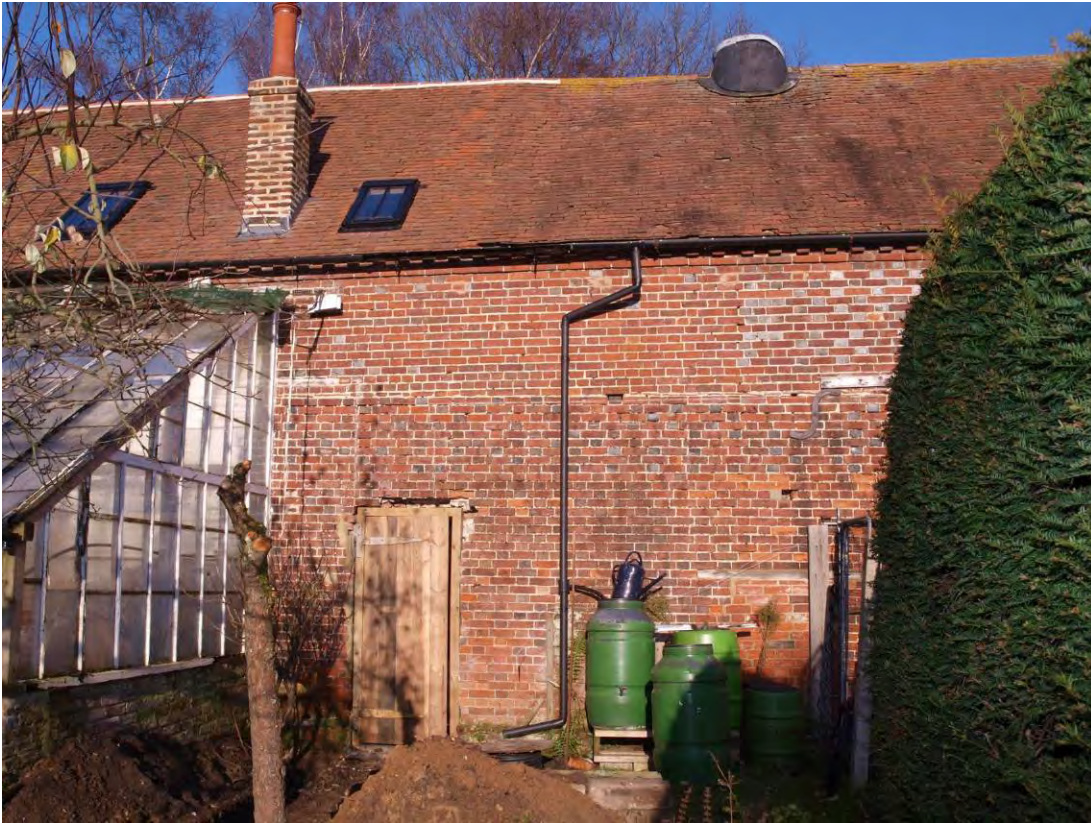
Plate 7: South elevation (eastern end of stable block) showing the two or possibly three phases of brickwork, looking north (12)
