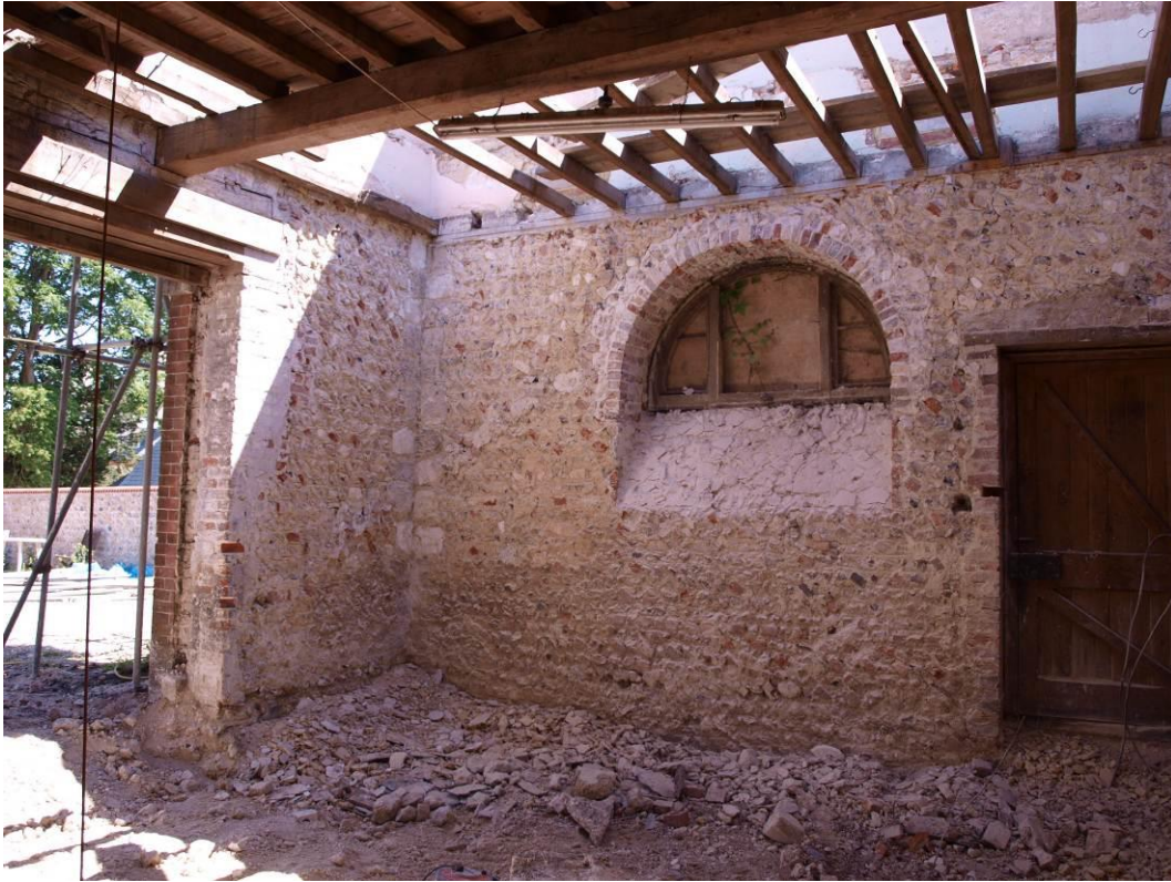
Plate 4.7: Site of former stair in Room 7; the blocked doorway seen externally is not visible internally (4).
