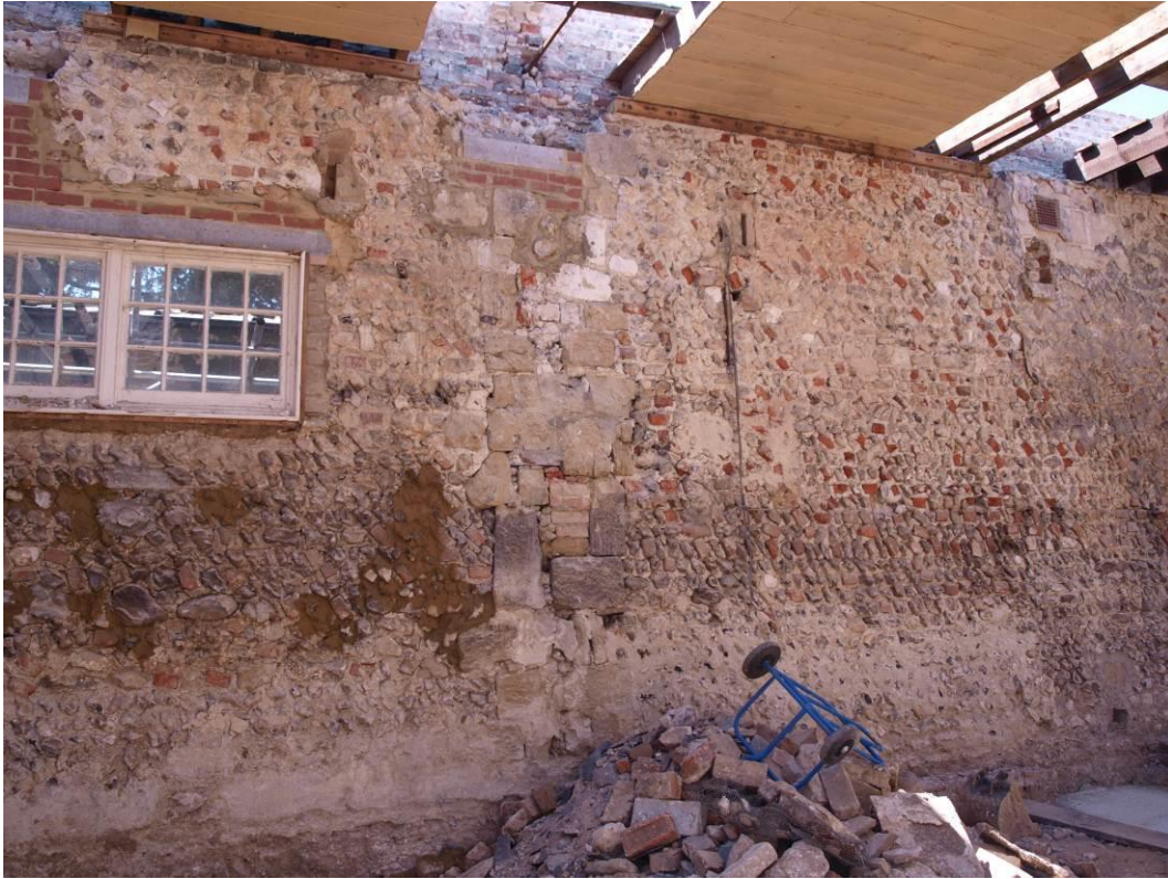
Plate 4.5: Chalk block quoins in south-west wall of Room 5 indicate the former location of an original partition wall (13).
