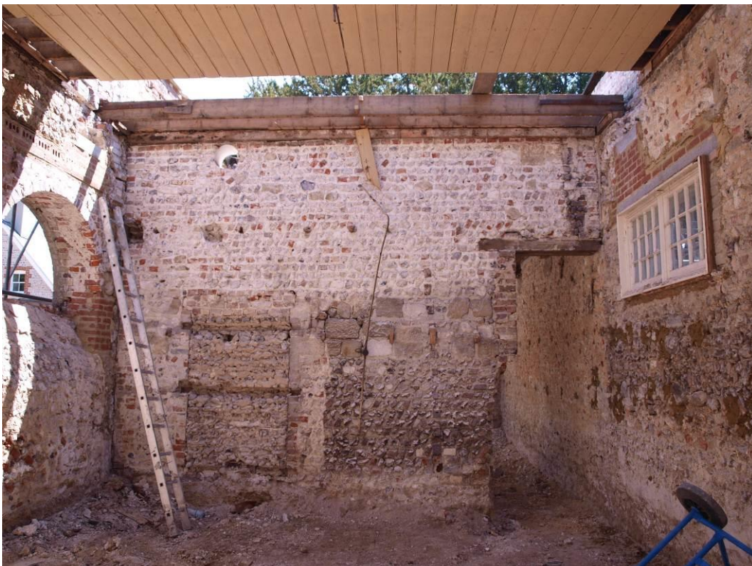
Plate 4.6: Blocked doorway and area of chalk blocks in a later partition wall forming the south-east wall of Room 5 (12).
