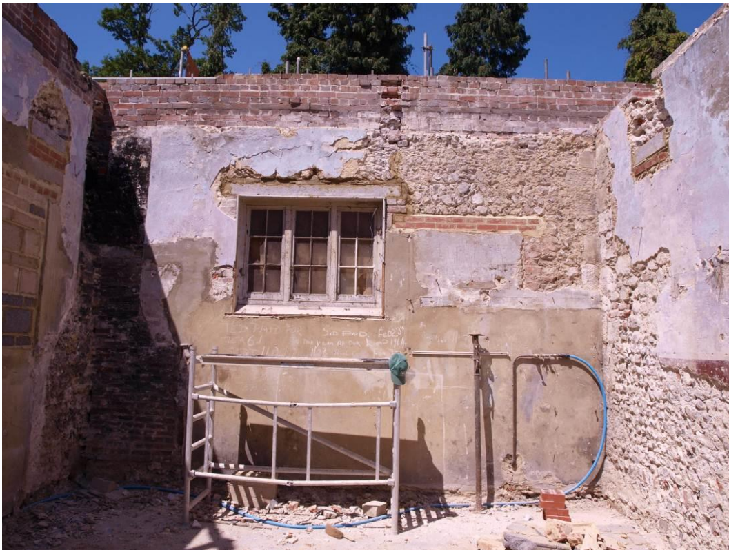
Plate 4.4: North-west wall of Room 2-4; location of former chimney breast to south and chalk block quoin construction of original partition wall to north (28).
