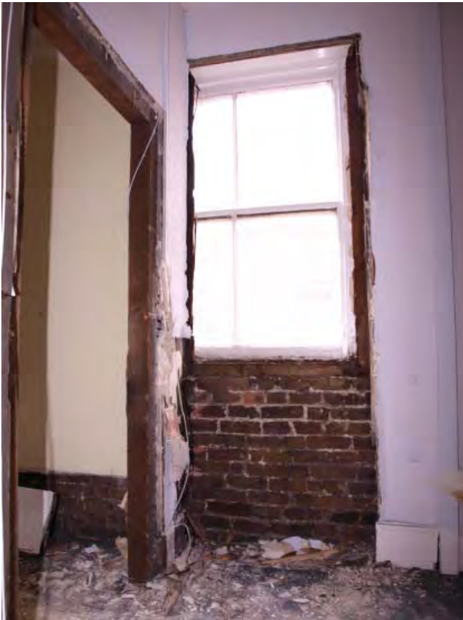
Plate 14 First floor landing (Room 4) showing window bisected by partition wall, looking west (18)
