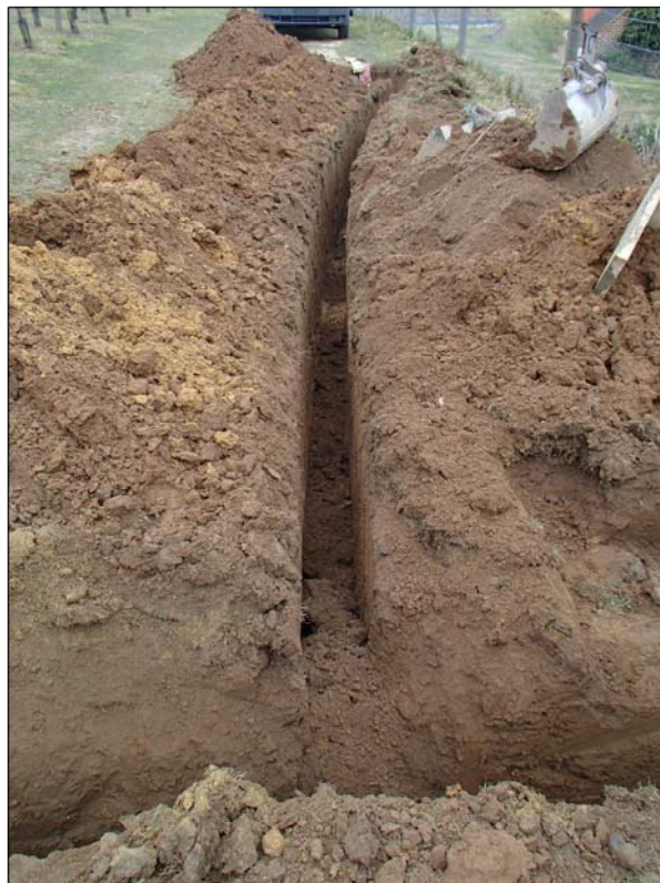
Fig. 3.b Micro Substation Area Facing East
