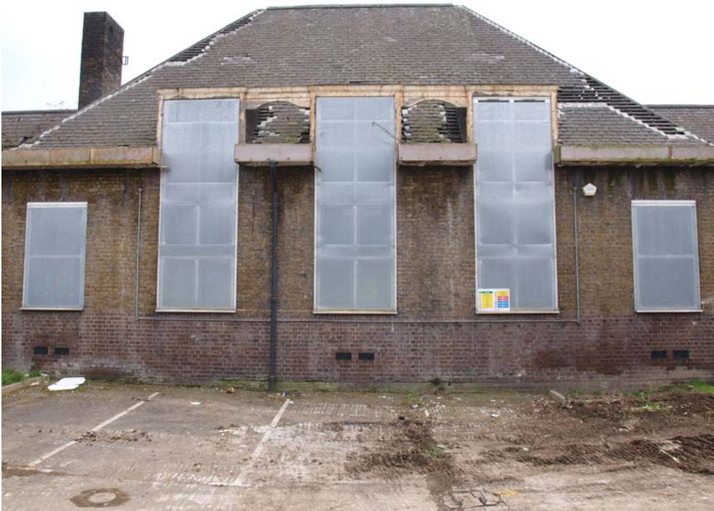
Plate 2. West elevation (central block), showing lucarne windows rising above the eaves. Facing east.
