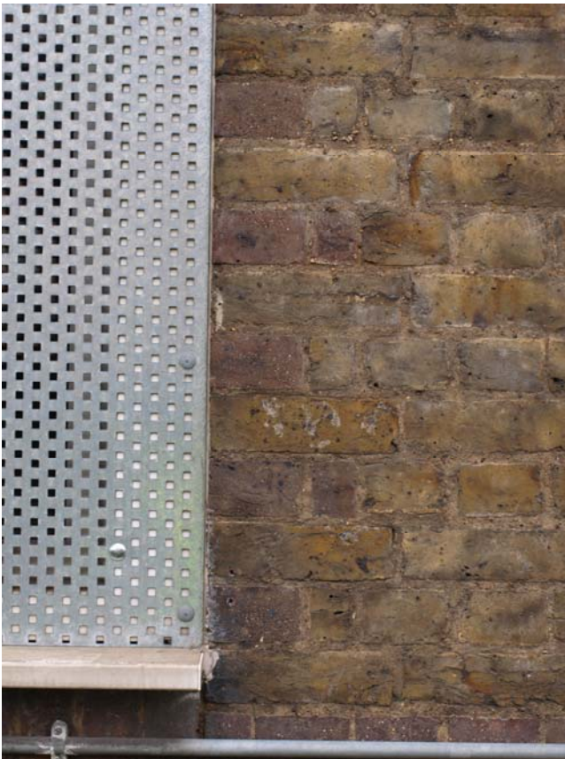
Plate 14. East elevation, detail of brickwork showing alternating red and yellow bricks at window jambs. Facing west.
