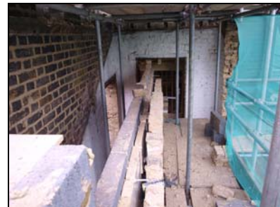
6119-18 (1/18) North elevation, after removal of part of the east end. Facing south
