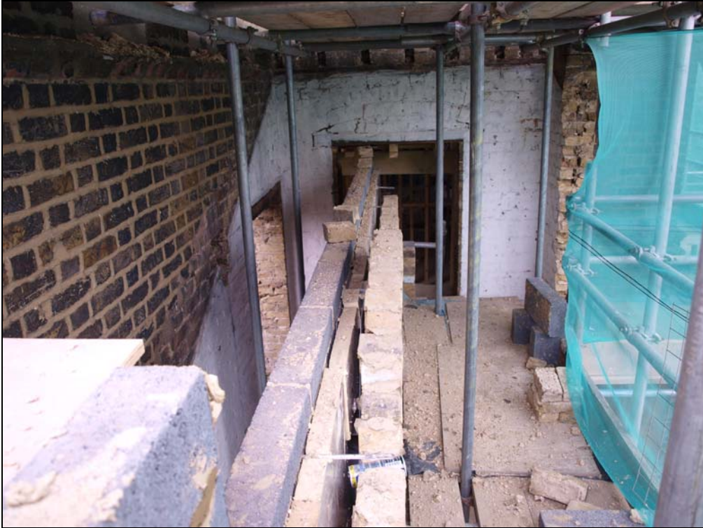
Plate 15. North elevation where the stair block has been removed, sockets visible below scaffold (18)
