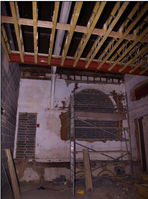
Plate 14. Blocked fire escape and window from interior, east elevation (34)
