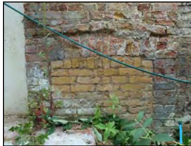
e2668-29 Blocked fireplace, southeast boundary wall. Facing southeast
