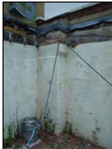
e2668-28 Corner buttress, junction of northeast and southeast boundary walls. Facing east
