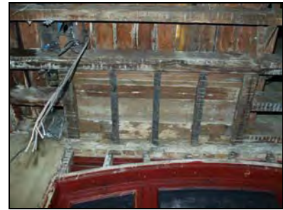
e2668-66 Interior, hearth for fireplace in first floor, viewed from below. Facing southwest
