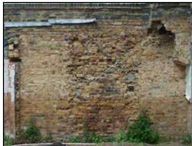
e2668-20 Detail, internal face of southwest boundary wall showing roof scar. Facing southwest
