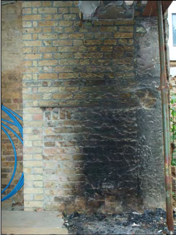
Plate 23. Blocked fireplace in outbuilding. Facing southeast (22)
