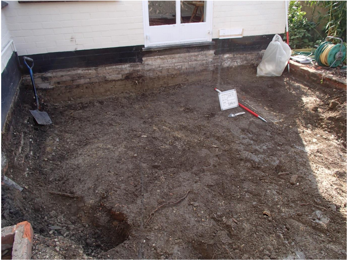
Photograph showing the 19 th / 20 th century pit during the Phase 3 groundworks (the modern garden wall can be seen in the background near to the ranging pole)
