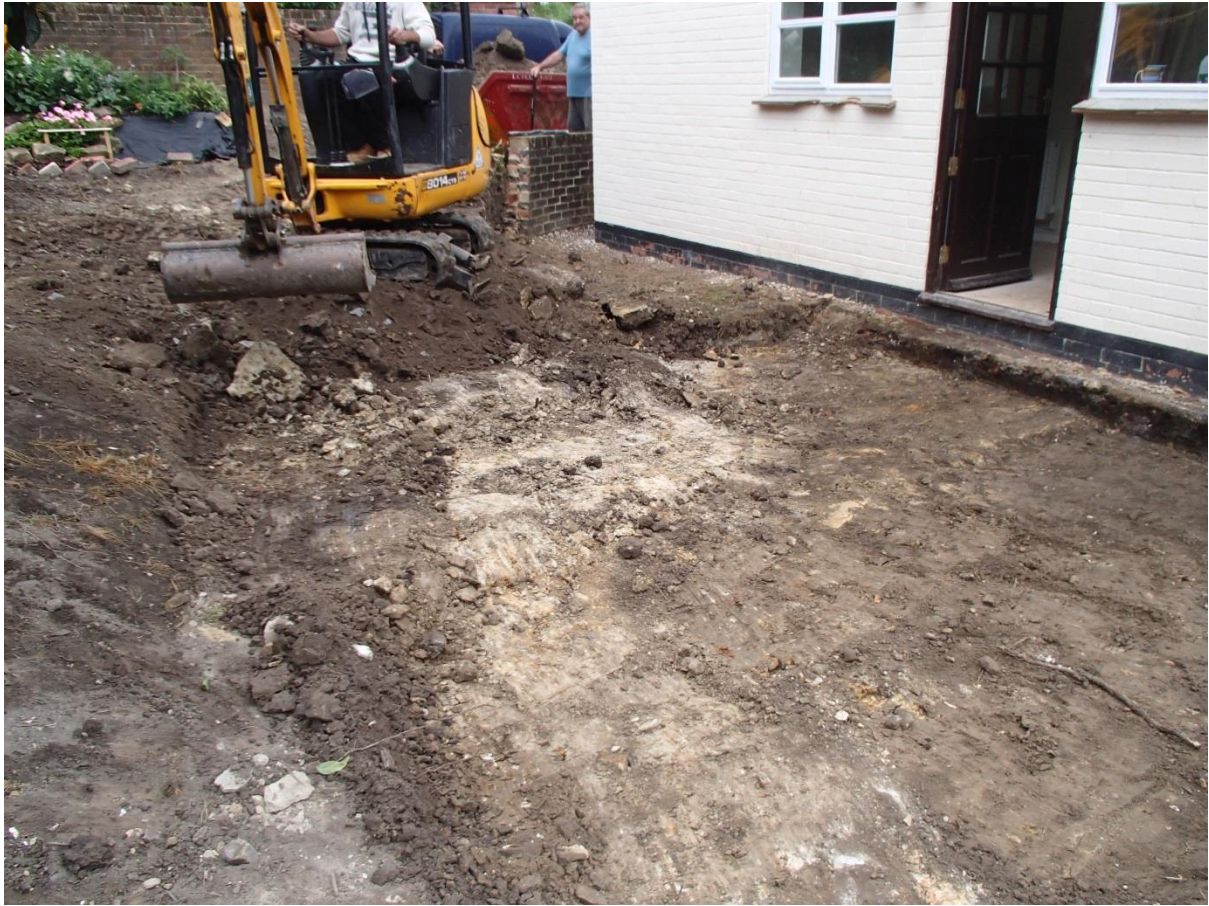
Photograph showing the shallow nature of excavations within the footprint of the new extension to the west of the existing building (Phase 2)
