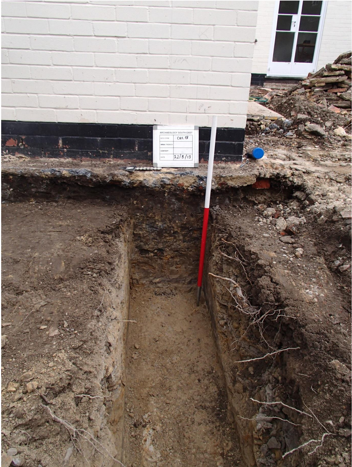
Photograph showing Phase 2 excavations for a foundation trench to the west of the existing building
