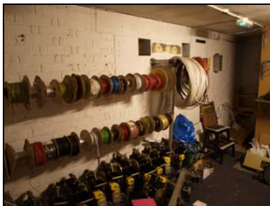
6431-223 Generator Block: HV Intake First Floor. Facing N
