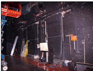
6431-022 Studio 1 Ventillation Ducts. Facing S
