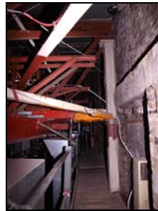
6431-032 Studio 1 Lighting Grid Support. Facing SE
