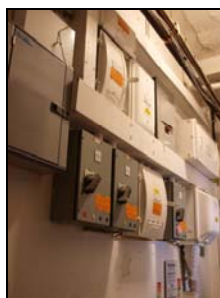
6431-083 Three Storey Block: Electrical Switches. Facing W
