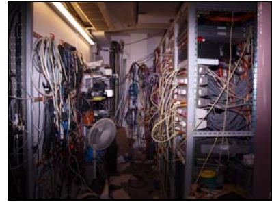
6431-042 Studio 1 Server Room. Facing SE
