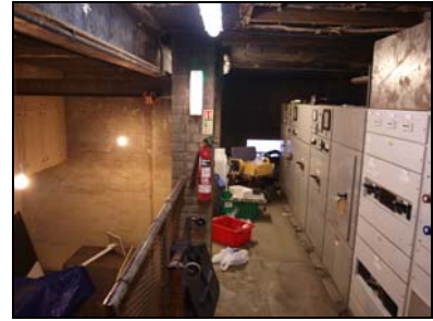
6431-222 Generator Block: HV Intake First Floor. Facing SW
