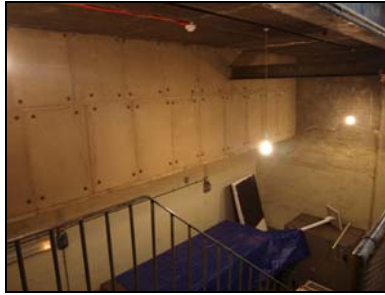
6431-221 Generator Block: High Voltage Intake Room. Facing S
