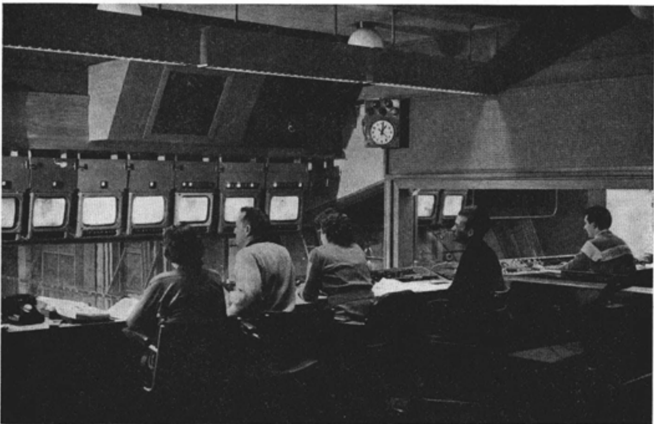
Fig. 3 — R1 Vision and Sound Control Room during rehearsal
