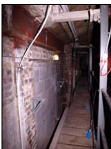
6431-034 Studio 1 Blocked Window. Facing NE
