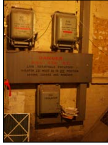
6431-134 Generator Block: BBC-Era Switches. Facing NE
