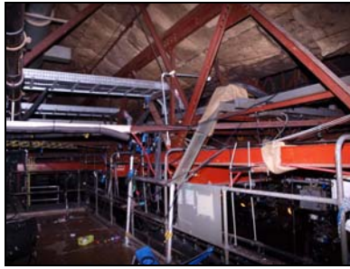
6431-038 Studio 1: Lighting Grid and Roof Truss. Facing SW
