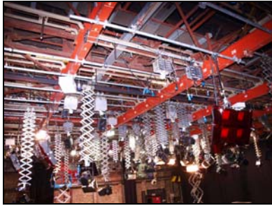
6431-040 Studio 1 Lighting Grid. Facing NW
