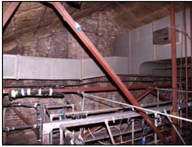
6431-181 Studio 1 Roof: Ventilation Duct & Insulation. Facing SW
