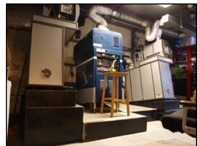
6431-108 Cinema Projection Equipment. Facing SW
