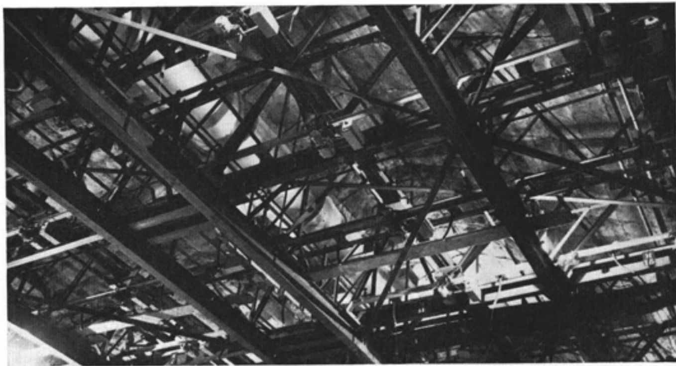
Plate B — Studio 1. Independently supported steelwork incorporating runway beams, motorized lighting batteries, and cable tray supports
