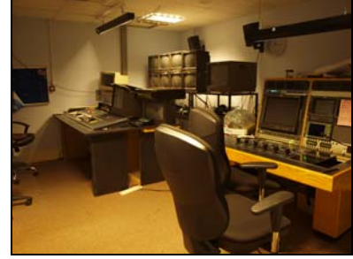
6431-174 Studio 1: Vision Control Room. Facing E
