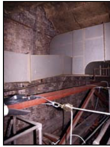
6431-182 Studio 1 Roof: Ventilation Duct & Insulation. Facing W
