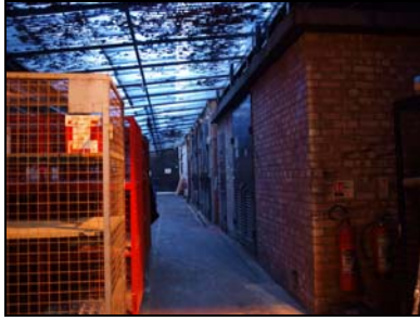
6431-136 Generator Block. Facing NE
