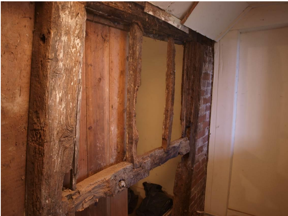
Plate 12: Original window in south wall of Bedroom 02, viewed from the landing to the south (17)
