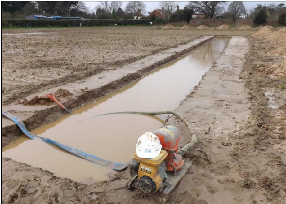
Figure 15. Trench 30 flooded, looking west
