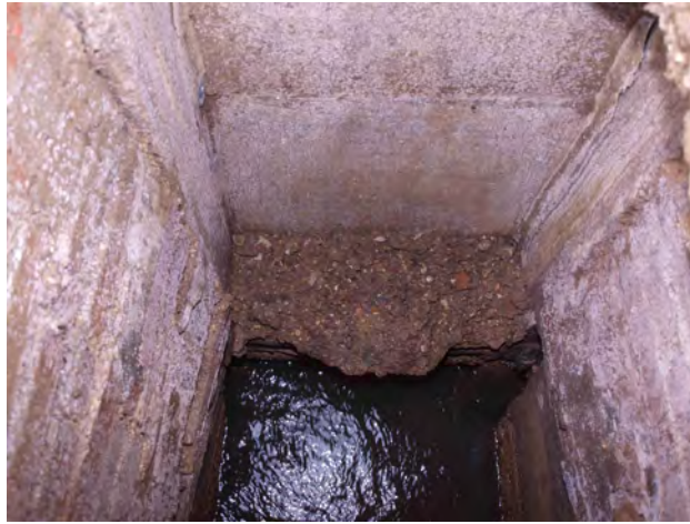
Plate 7: A detail of the interior of the brick lined inspection chamber with the remains of the former eastern sluice gate housing still in situ
