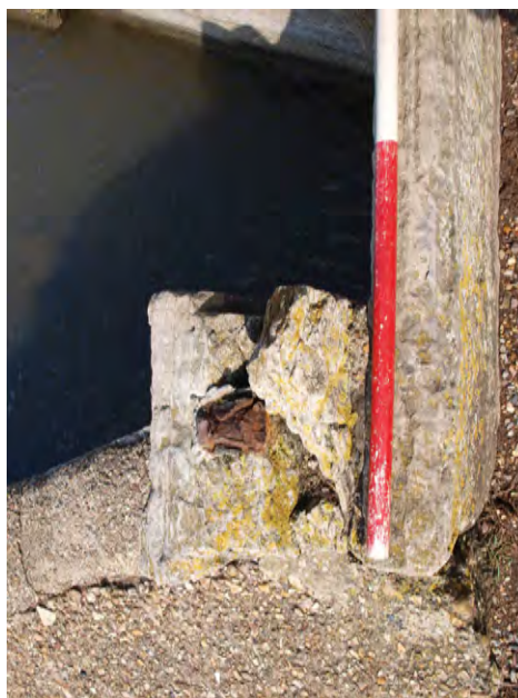
Plate 9: The south west corner of the in situ west sluice gate showing a similar socketed masonry support
