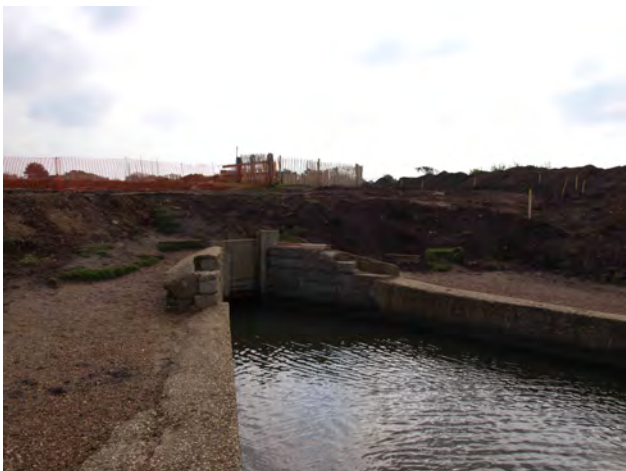
Plate 5: The stone sluice with the shuttered concrete extensions to the wing walls and the concrete repair and capping to the original revetments.
