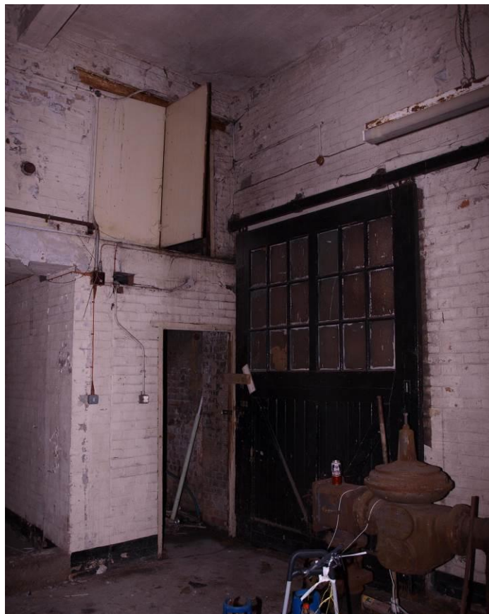
Plate 21 The door leading west from Room 14. Note the storage space above the compartments (Rooms 15 and 16)
