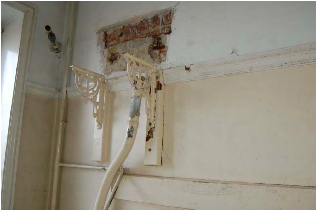
Plate 40: Cast iron cistern bracket in Room F16 in Building 1, viewed to north-east
