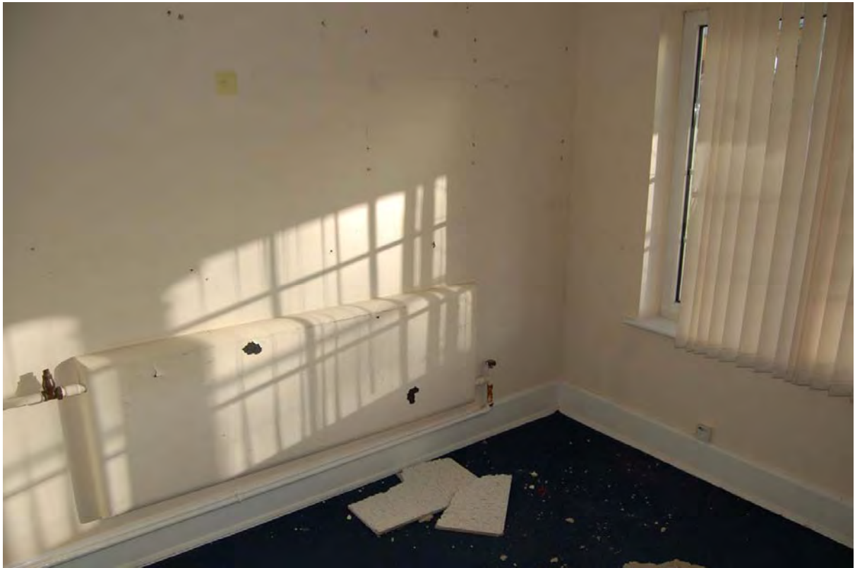
Plate 95: Typical radiator in patients rooms facing onto veranda in Building 6
