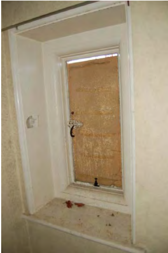
Plate 37: Detail of small window with fancy cast iron handle in Room F07 in Building 1
