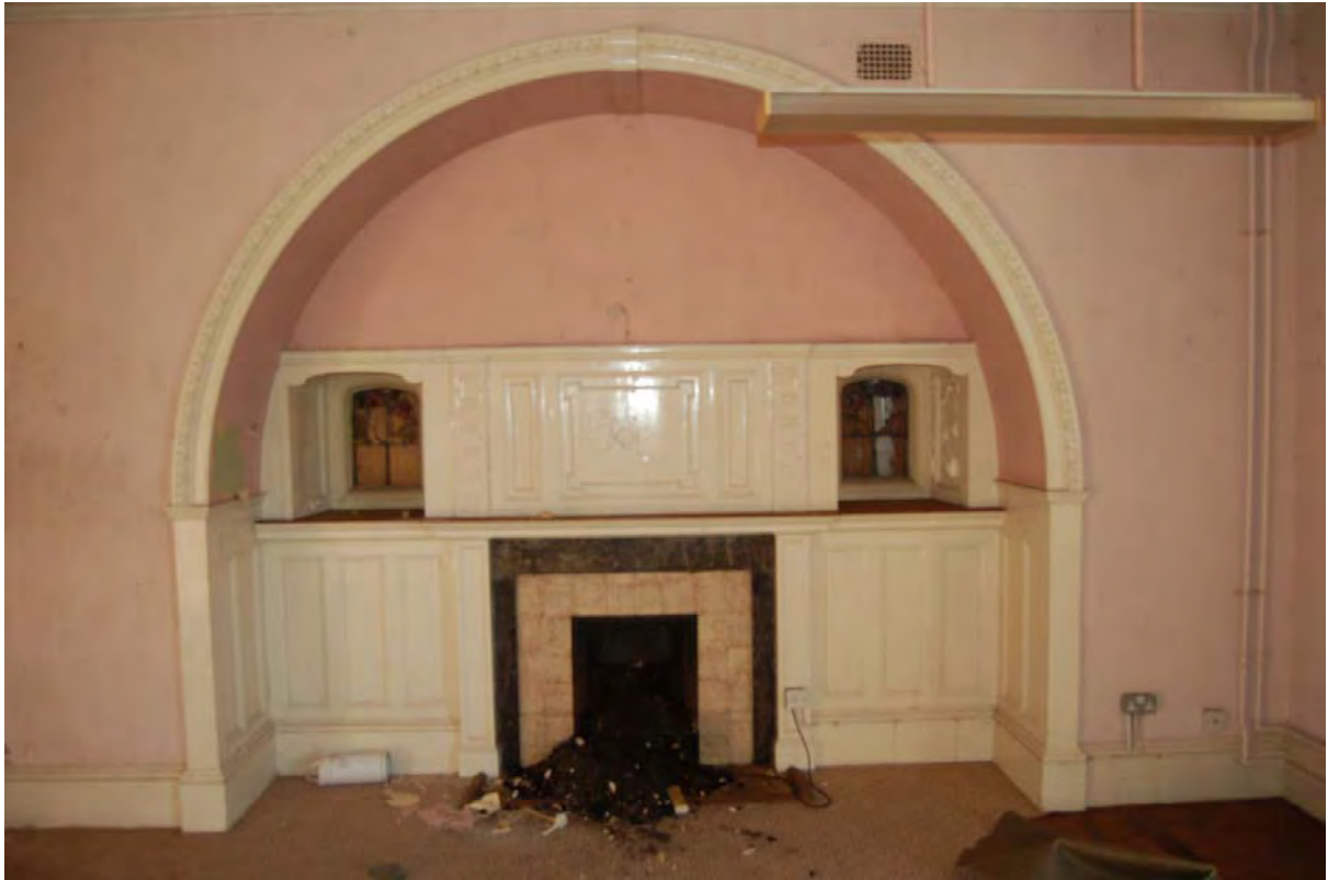
Plate 27: Alcove and fireplace on south-east wall of Room G15, viewed to south-west
