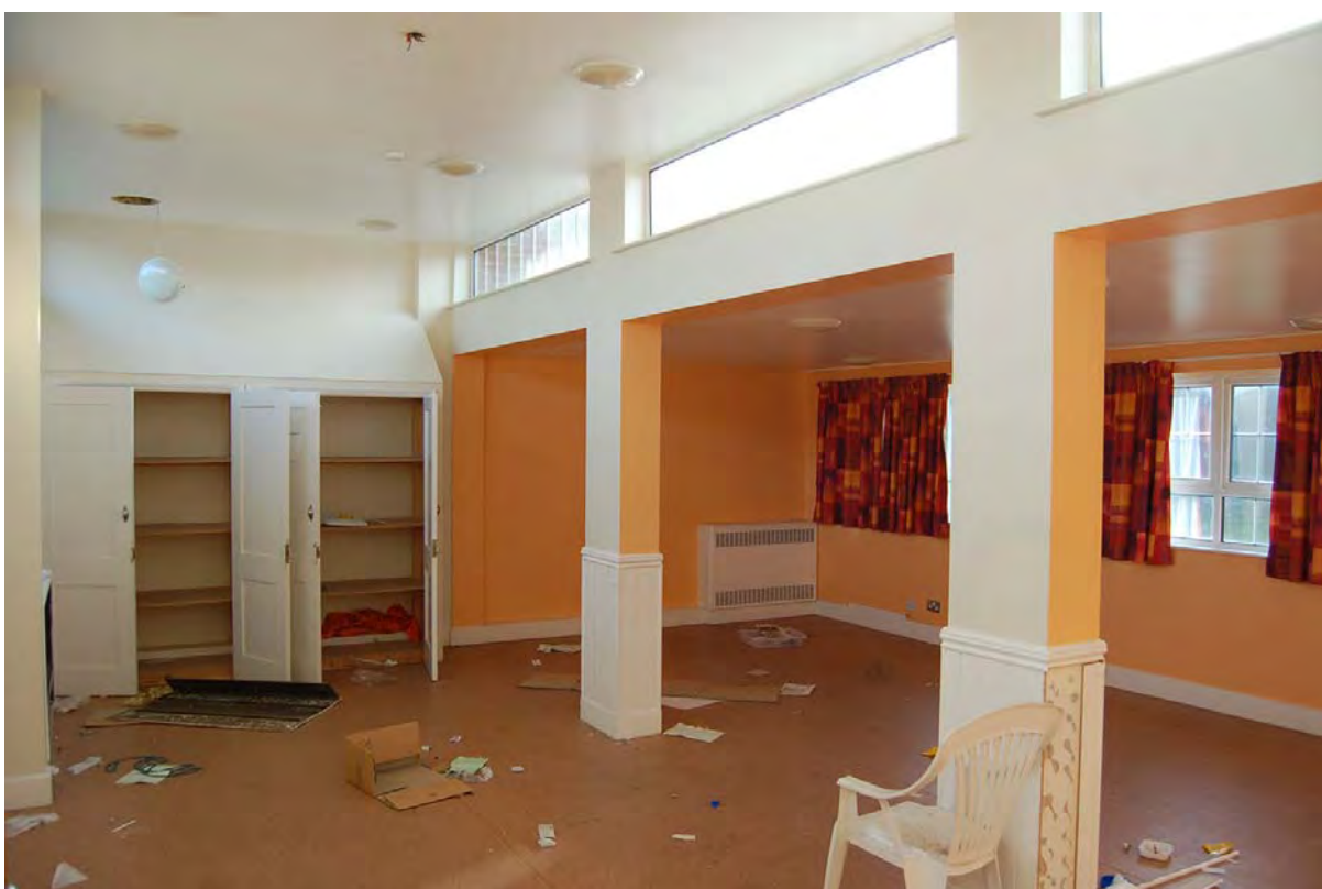
Plate 90: Interior view of modern dayroom occupying part of former west veranda in Building 5
