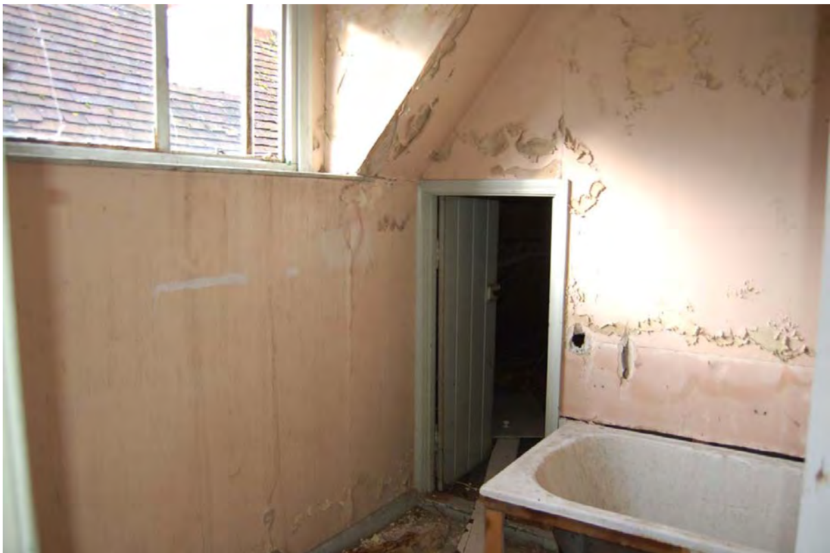
Plate 54: Bathroom A02 and entry to roof space in Building 1, viewed to north-west
