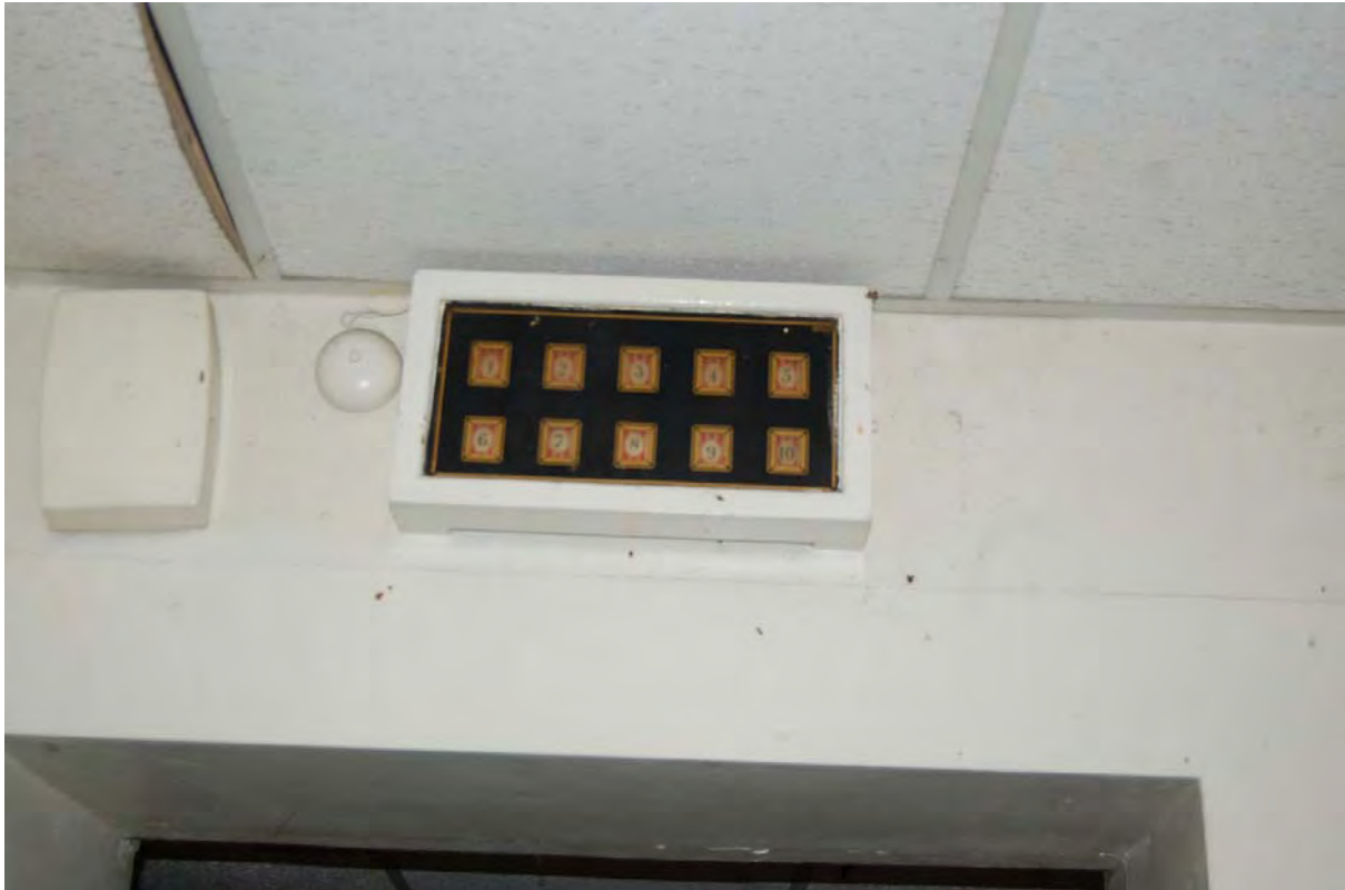
Plate 33: Modern room call panel between corridors G29 and G22
