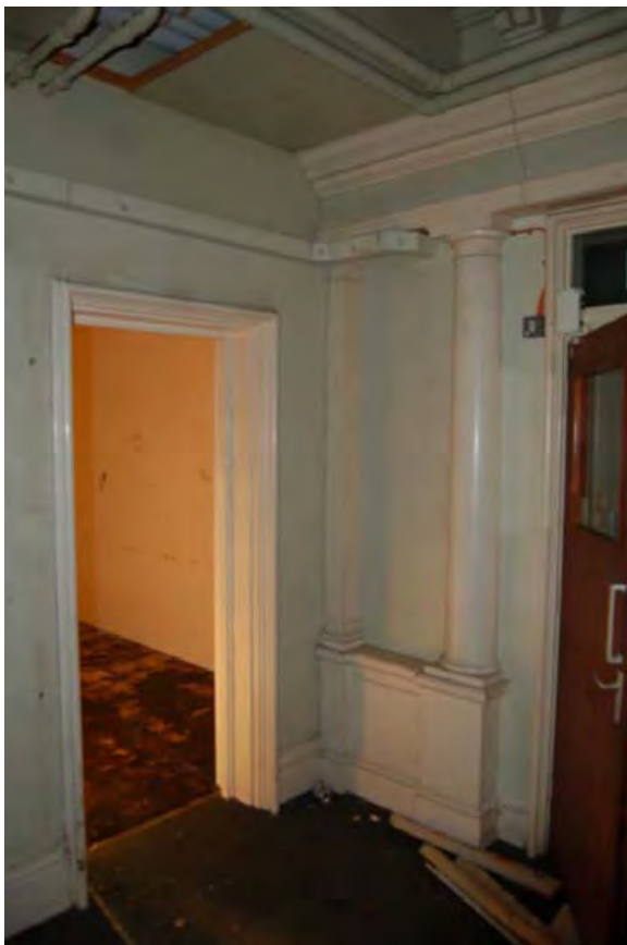
Plate 16: Remains of internal wall detailing in lobby GO3 of Building 1
