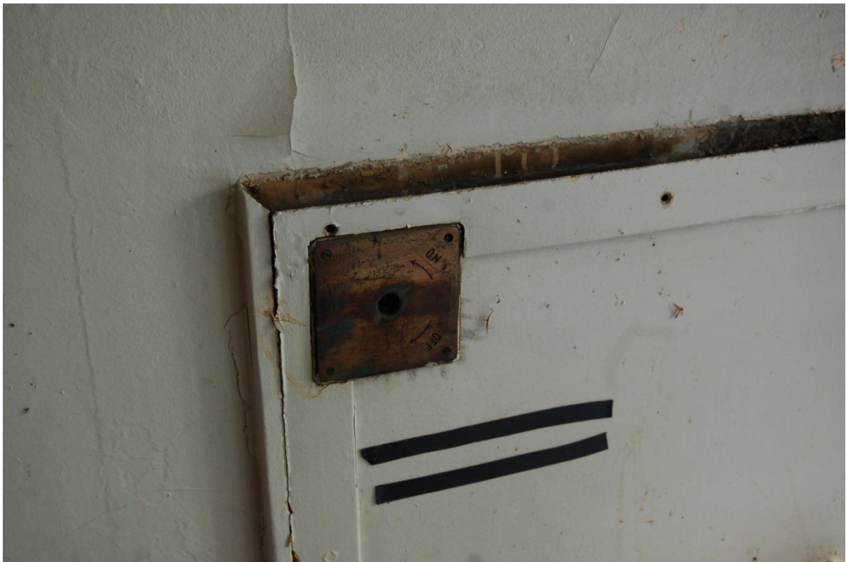
Plate 44: Room 14, radiator control detail
