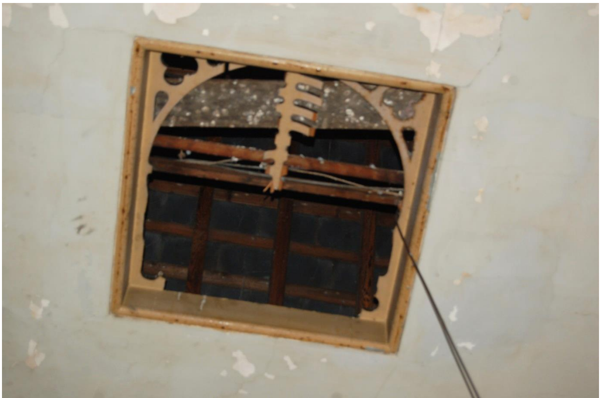
Plate 18 Cast iron ceiling vent
