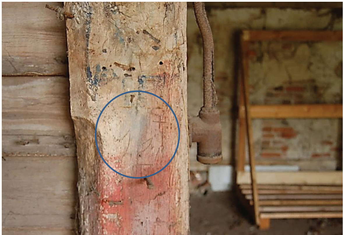
Plate 10 Graffiti on bay post
