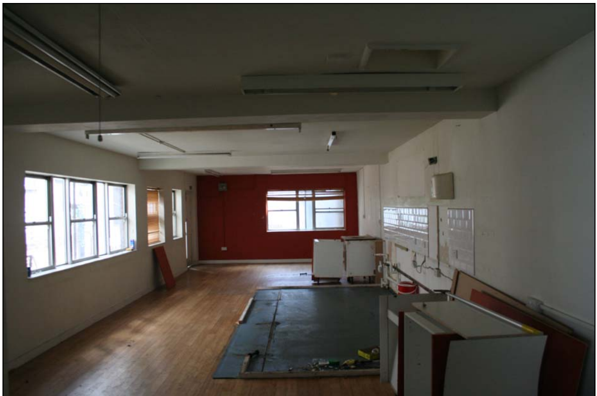
Plate 12. Building A, ground floor, office space to south of lobby area (FCQ14-0055)
