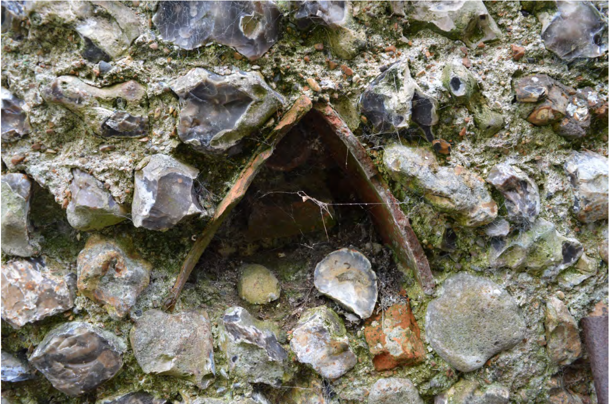
Plate 9: Probable blocked vent to Building 7 (47)
