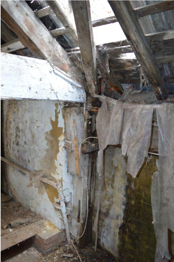
Plate 15: Jowled post on eastern side of Building 12 (15)
