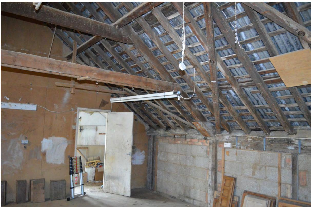
Plate 16: Truncated tie beam in Building 14 (23)
