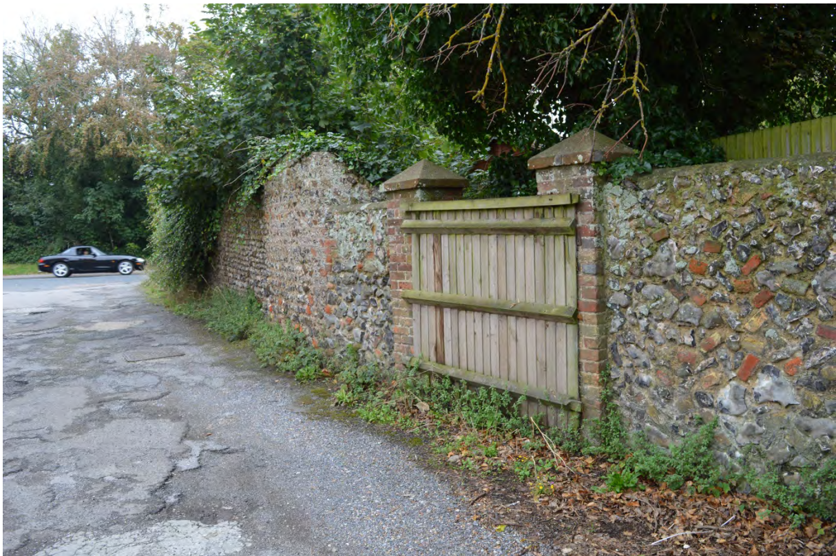
Plate 22: Looking east along the later section of wall, constructed in bungaroosh with brick gate piers; the curved section of wall is visible beyond (61)
