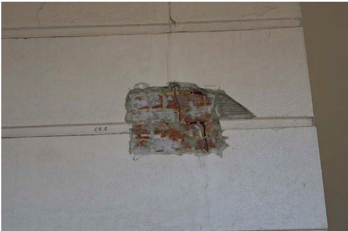
Plate 2: Removal of stucco revealing underlying Fletton brickwork at ground floor level (72)
