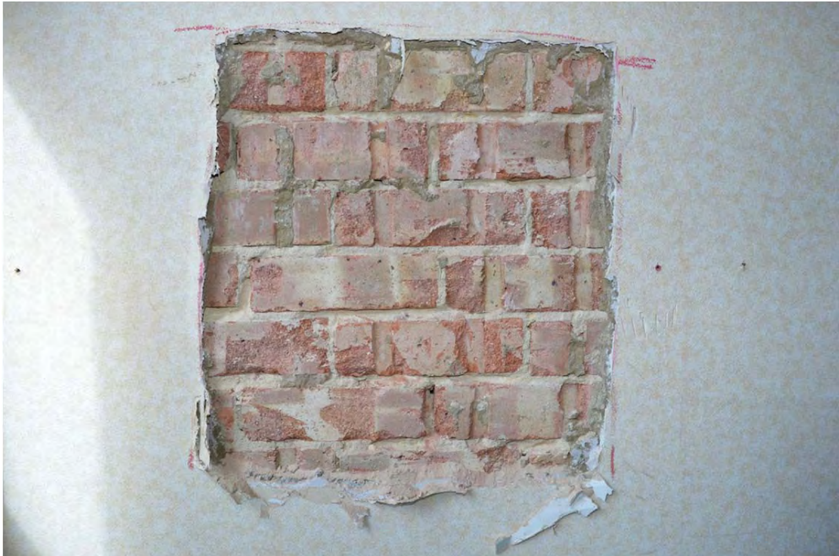
Plate 13: Exposed construction to west party wall of 17 Park Crescent at third floor level (3)
