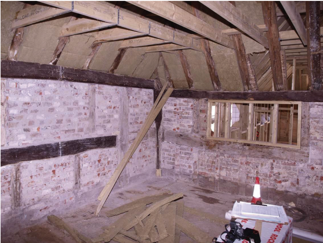
Plate 9: Hall chamber, looking east, showing interior brick/tile cladding to studs of south-east wall (22)
