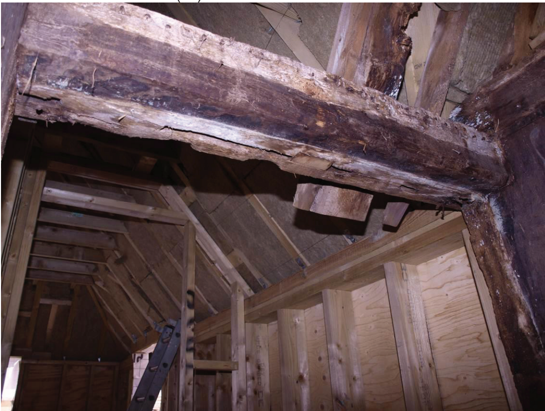
Plate 10: Redundant mortices in soffit of wall-plate on first floor landing (28)
