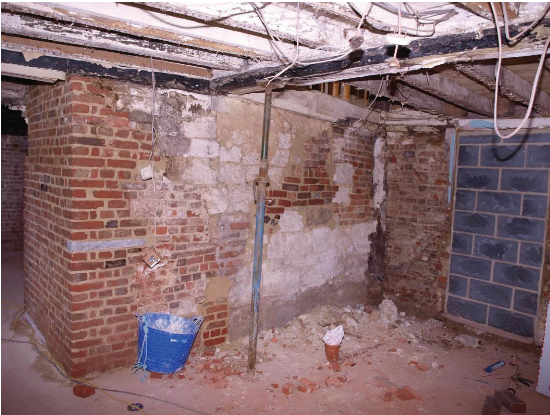
Plate 7: The exposed construction of the back of the chimney stack at ground floor level (1)
