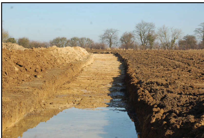
3.3 General view showing the flooded access track in the vicinity of feature [22]
