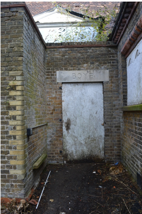
Plate 6: Doorway in late 19 th /early 20 th century addition on west side of south range (29)
