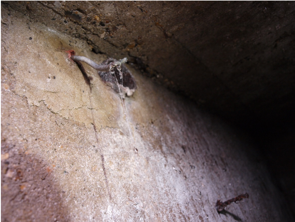
Plate 13: Electrical cable by door within the shelter.
