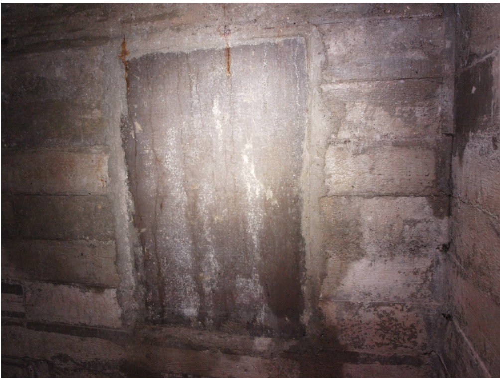
Plate 14: Blocked crawlspace in the north wall of the shelter.
