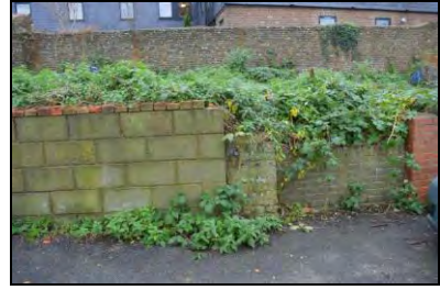
6969-0069 Retaining wall, Section 4, modern in-fill of suspected former access point. Facing west
