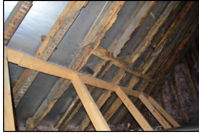
6969-0056 Building 1 roof interior, note the gap in the purlins for a probable loading bay. Facing southwest
