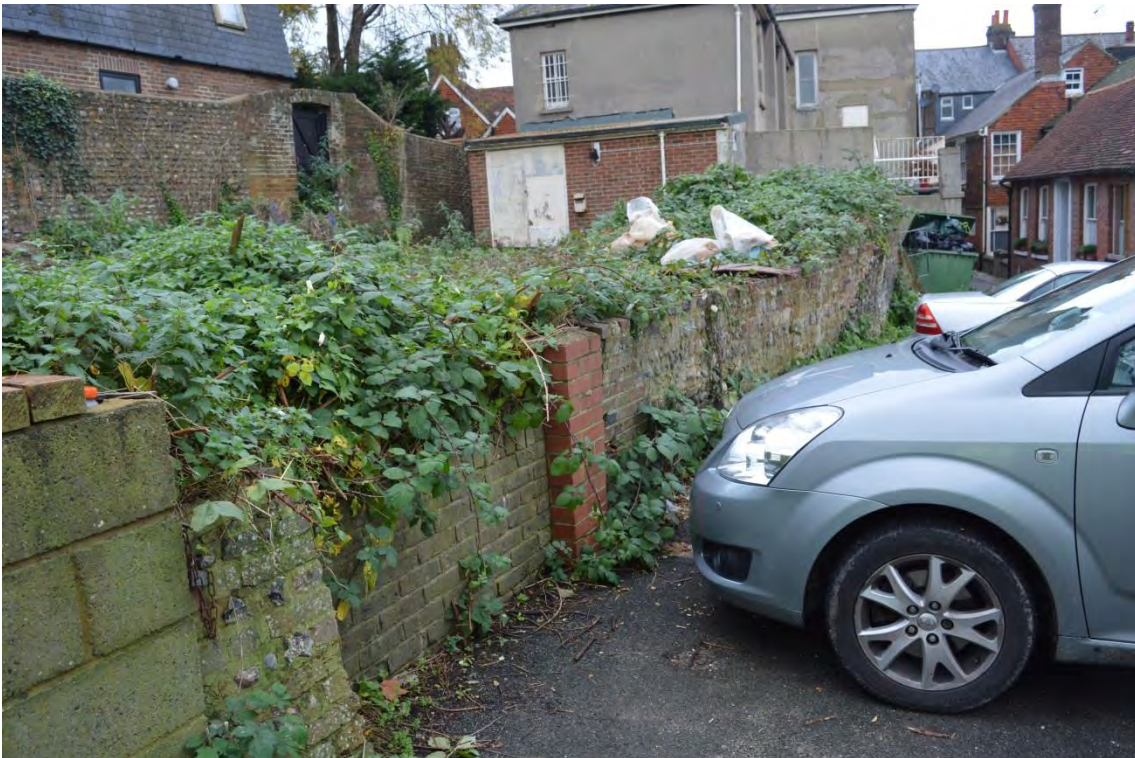
Plate 28: Retaining wall, Section 4, modern in-fill of suspected former access point, facing north-west (6969_0070)
