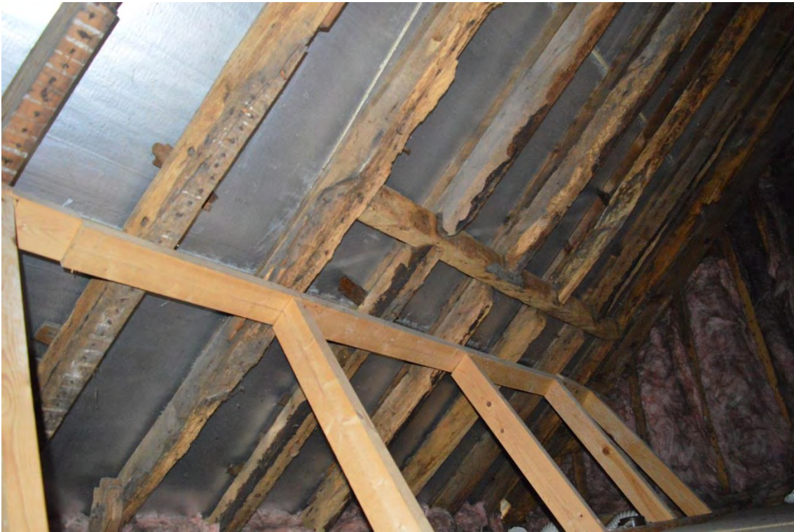
Plate 17: Building 1 roof interior, note the gap in the purlins for a probable loading bay, facing south-west (6969_0056)
