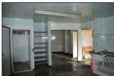
6969-0043 Building 1, interior, main circulation area between the southern and northern ranges. Facing southwest
