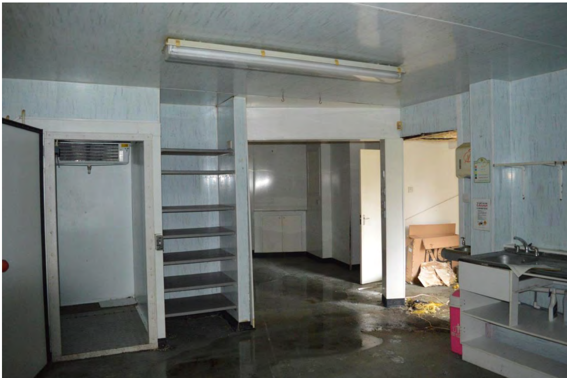
Plate 10: Building 1 interior, main circulation area between the southern and northern ranges, facing south-west (6969_0043)
