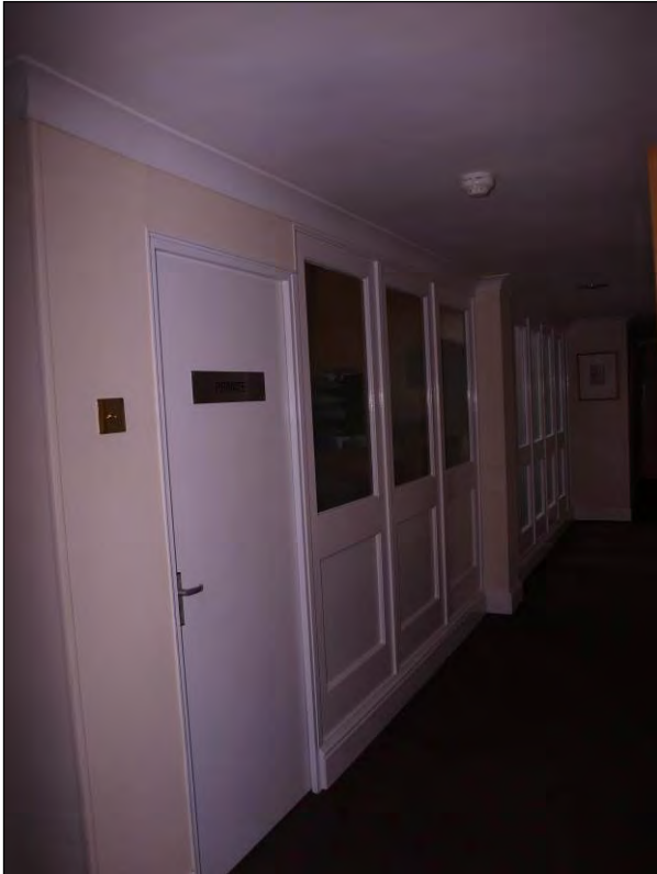
Photo 91: First floor, western extension access corridor, Office door (no access), facing north-east (7195-0091)
