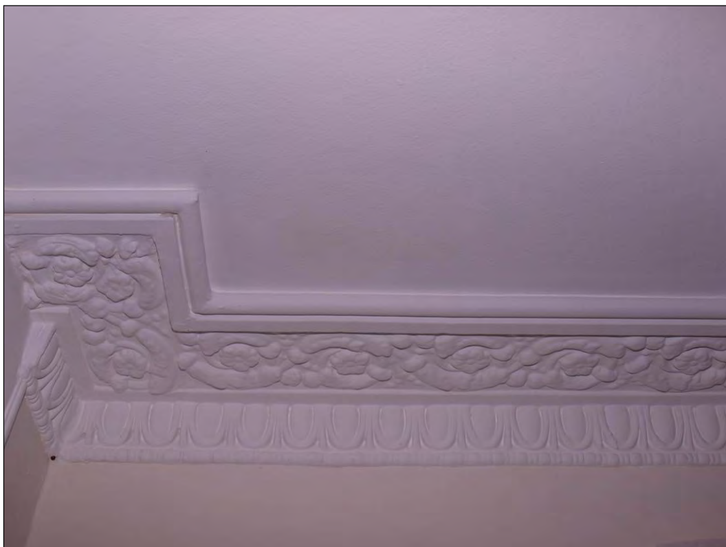
Photo 54: First floor, Room 1, cornice moulding, located to the west of the mock-Tudor extension, facing south (7195-0054)
