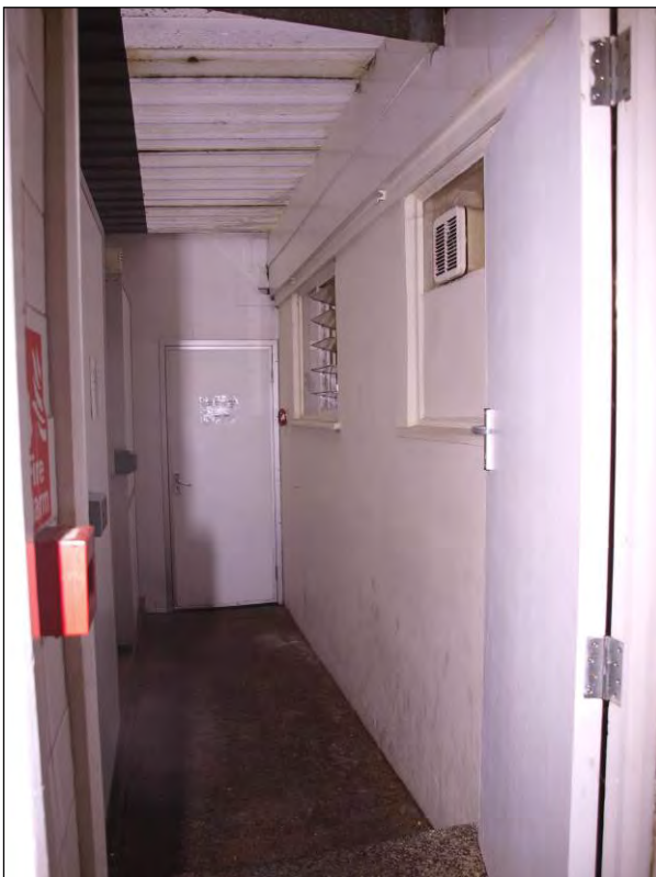
Photo 6: Ground floor, Freezer Store corridor and access to southern end of Outbuilding 1, facing east (7195-0006)
