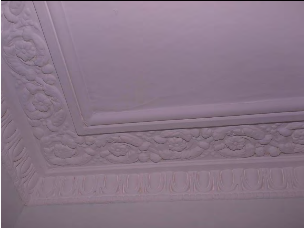
Photo 49: First floor, egg & dart cornice / floral moulding, above Room 1 entrance, facing south (7195-0049)
