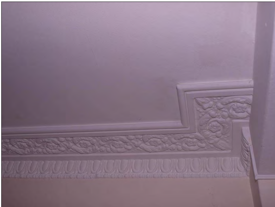
Photo 53: First floor, Room 1, cornice moulding in mock-Tudor frontage replicating that in adjoining area, facing south (7195-0053)
