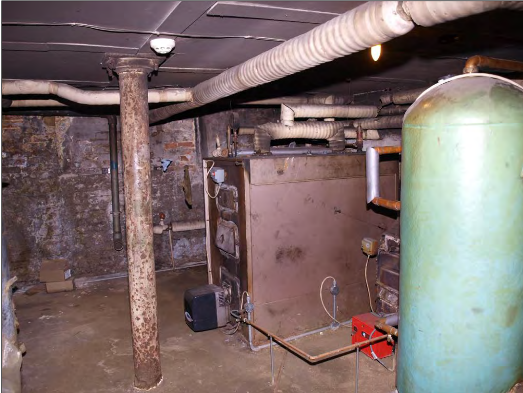
Photo 99: Basement, Boiler Room, facing south-west (7195-0099)
