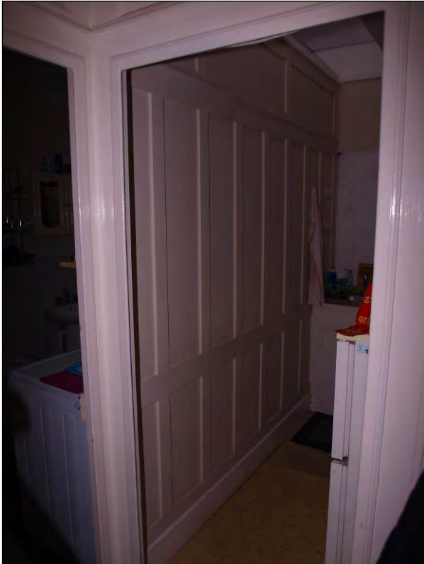
Photo 81: First floor, northern extent (converted self-contained accommodation), Kitchen / Bathroom partition, facing north-west (7195-0081)
