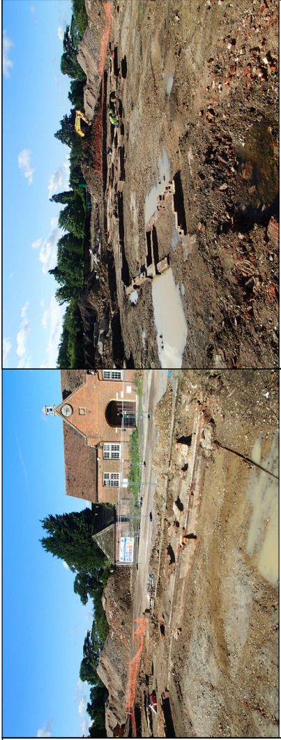
3.1 Western side of Area 1 showing yard wall and pliers to structure 7. Coach house to rear. View SW.
