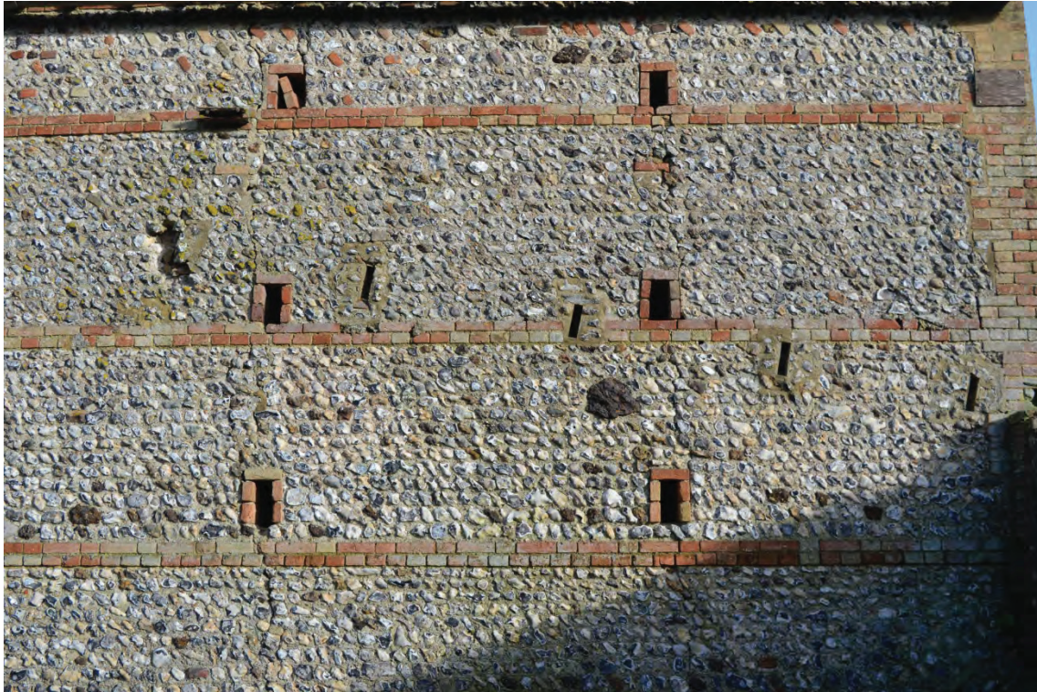
Plate 9: New Barn, detail of redundant inserted sockets on the eastern side of the southern elevation (7251_0011)
