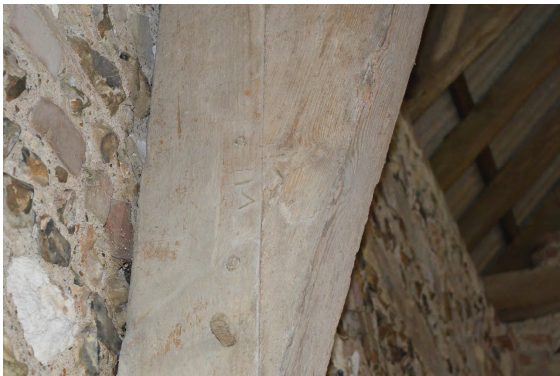
Plate 15: New Barn, detail of neatly chiselled carpenters marks to south end of Truss 7, facing south-west (7251_0035)
