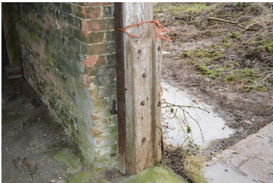
Plate 18: New Barn, grooved block for lower leap boards attached to northern post of Truss 5, facing north-west (7251_0033)
