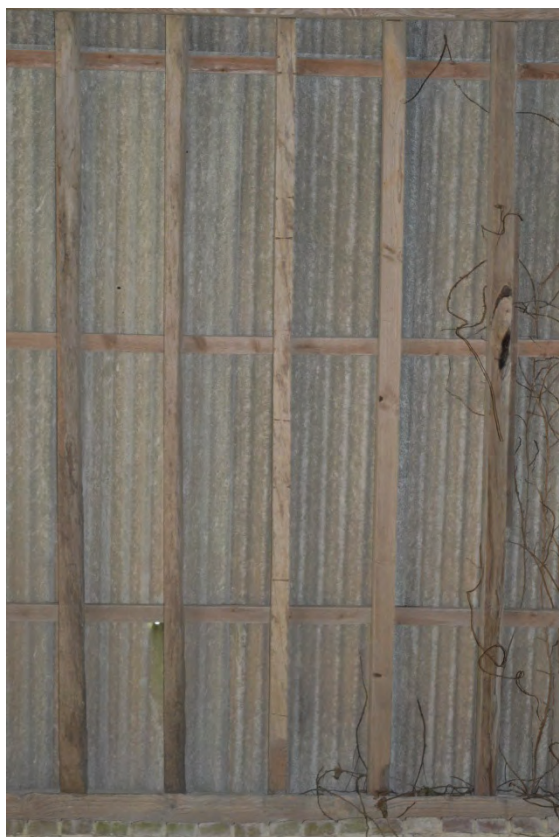
Plate 21: New Barn, detail of stained rafters caused by securing a former thatch roof, facing south (7251_0030)
