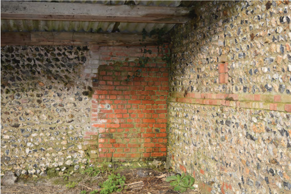
Plate 25: Detail of former opening within the west wall of the main, facing west (7251_0009)
