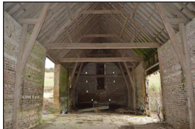
7251-0023 New Barn, interior view of midstreys and east storage bay. Facing east
