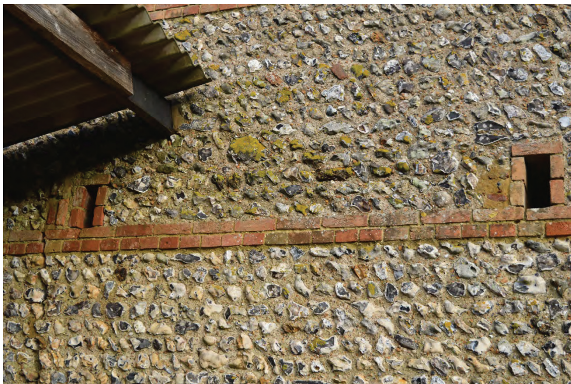
Plate 7: New Barn, detail of patch repairs to western side of southern elevation, facing north (7251_0008)
