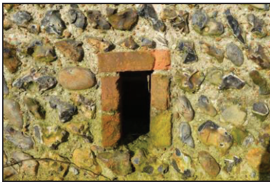
7251-0004 New Barn, detail of a ventilation hole on the east elevation. Facing west
