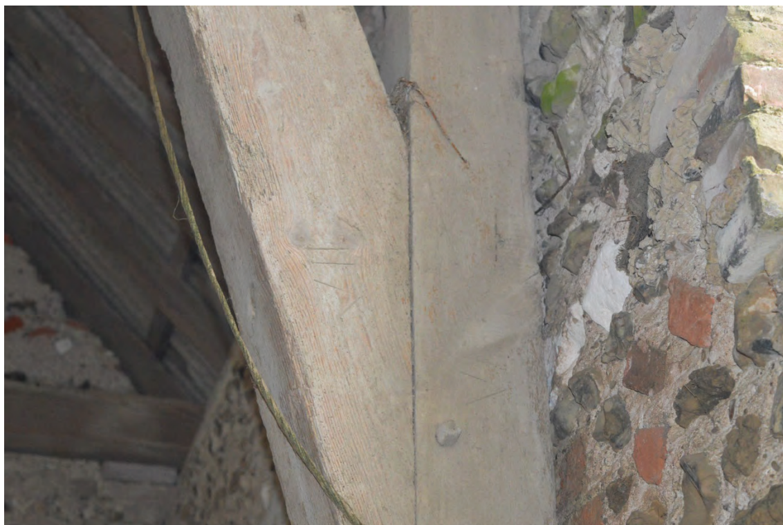
Plate 14: New Barn, detail of scribed carpenter's marks to north end of Truss 7, facing north-west (7251_0036)
