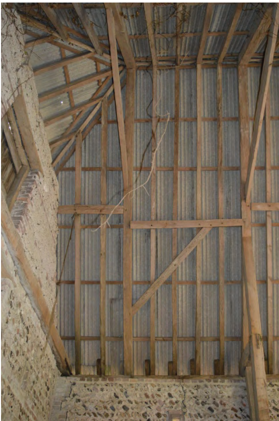
Plate 12: New Barn, interior view of the eastern storage bay roof construction, facing south (7251_0028)
