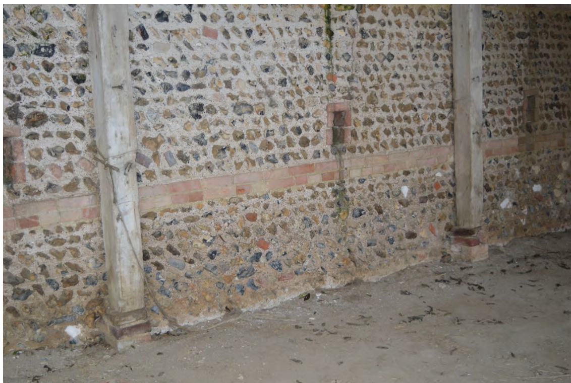
Plate 13: New Barn, interior view of supporting brick plinths situated to the west end of the southern elevation, facing south-west (7251_0037)
