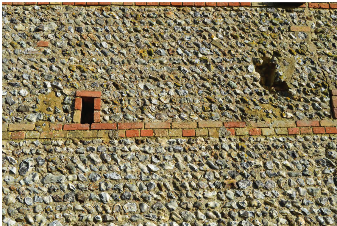
Plate 8: New Barn, detail of patch repairs to eastern side of southern elevation, facing north (7251_0010)
