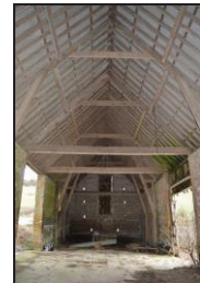
7251-0024 New Barn, interior view of roof construction over midstreys bay. Facing east
