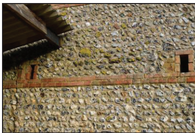
7251-0008 New Barn, detail of patch repairs to western side of southern elevation. Facing north
