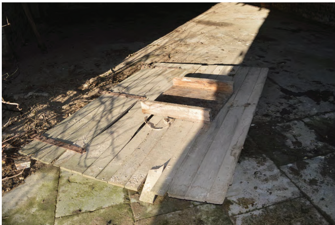
Plate 3: Detail of timber boarded door (of modern construction) from either the north or south elevation (now detached) (7251_0019)
