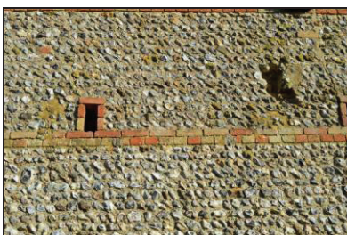
7251-0010 New Barn, detail of patch repairs to eastern side of southern elevation. Facing north
