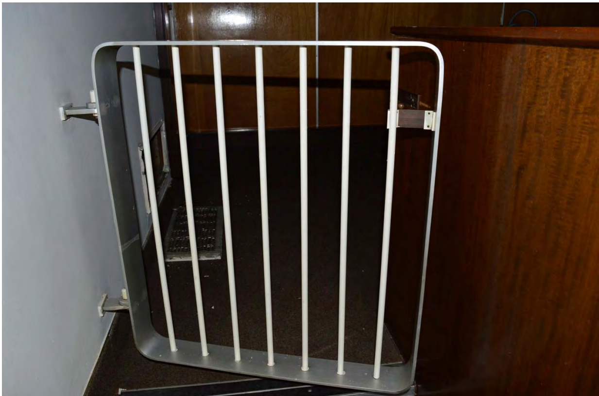
Plate 18: Magistrates court, detail of metal gate separating magistrates bench and seating area (7338_049)
