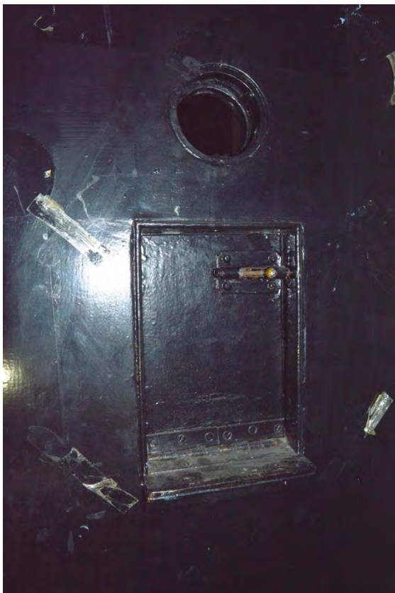
Plate 50: Magistrates court, detail of original cell door to Room B3 in western range (7338_170)
