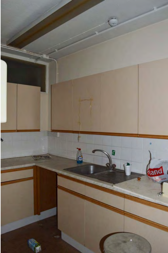
Plate 65: Magistrates court, view of kitchen in the northern range at first floor level (7338_143)
