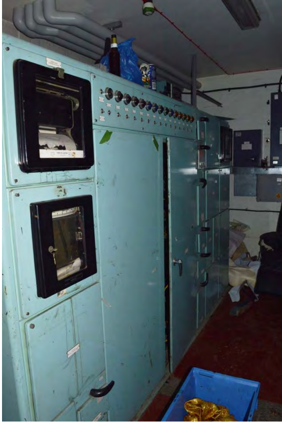
Plate 83: Police station, detail of early heating system machinery within the basement (7338_233)
