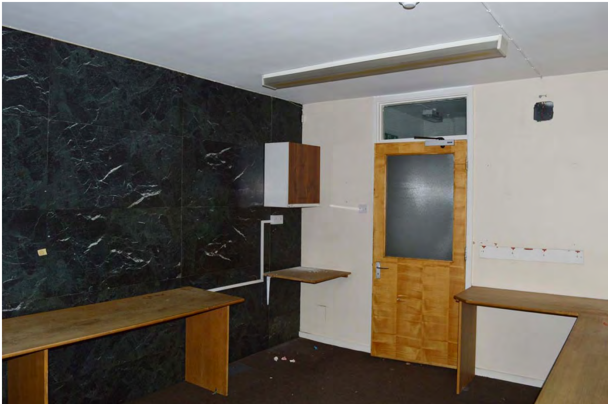
Plate 67: Magistrates court, view of northern mezzanine office, original lobby extent at first floor (7338_148)
