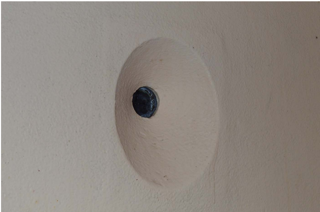
Plate 56: Magistrates court, view of inspection window to Room B7 cell in the western range (7338_180)
