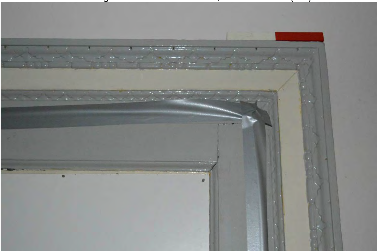
Plate 66: Detail of architrave to original entrance to Room B10, from room side (330)
