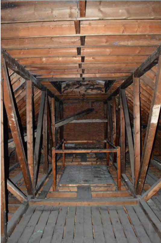
Plate 117: Roof above south range showing borrowed light to first floor corridor below (298)
