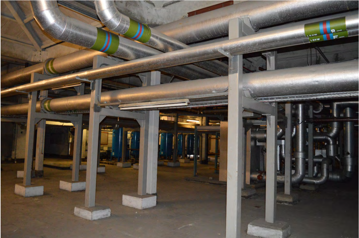
Plate 29: Fifth floor chilling plant (23)
