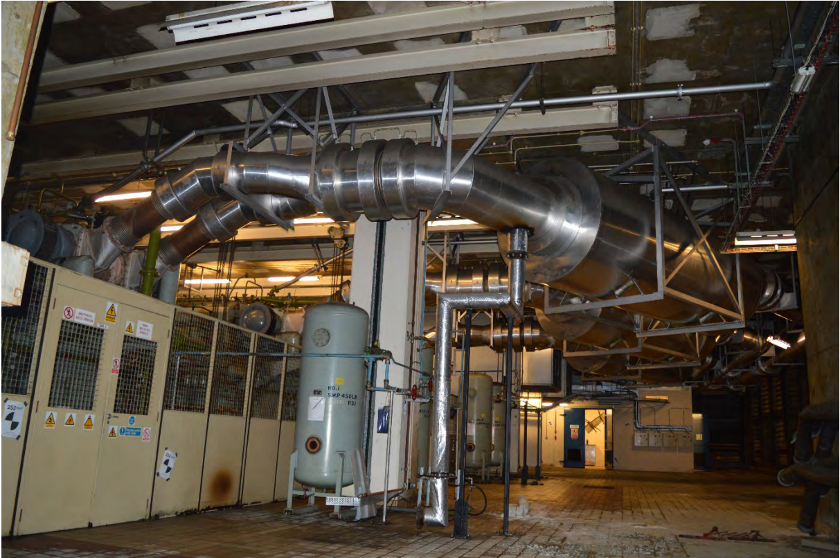
Plate 21: Engine exhausts in sub-basement (57)
