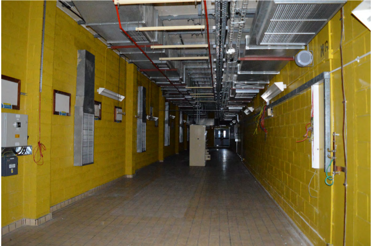
Plate 25: Interior of first floor substation (160)
