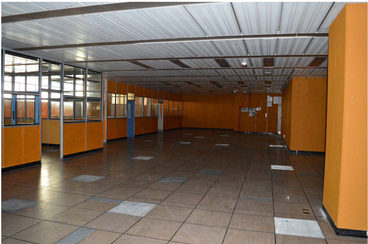
Plate 26: First floor telex switchroom (167)
