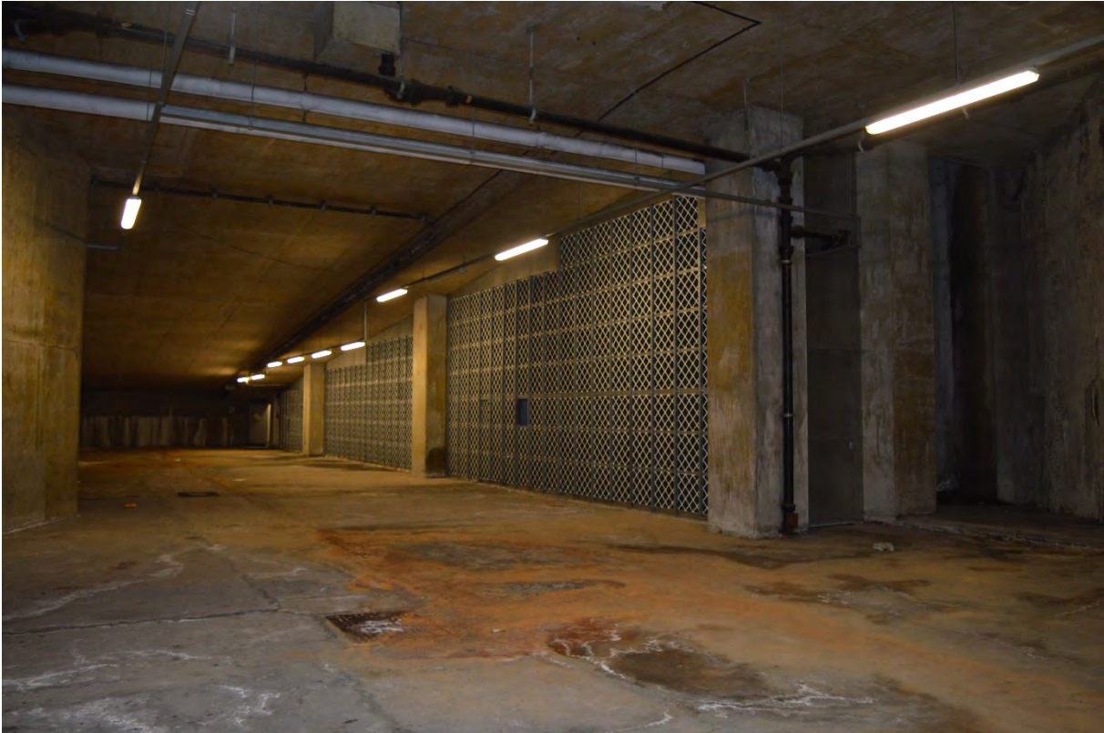
Plate 23: Air inlet on south wall of sub-basement, beneath vehicle ramp (61)
