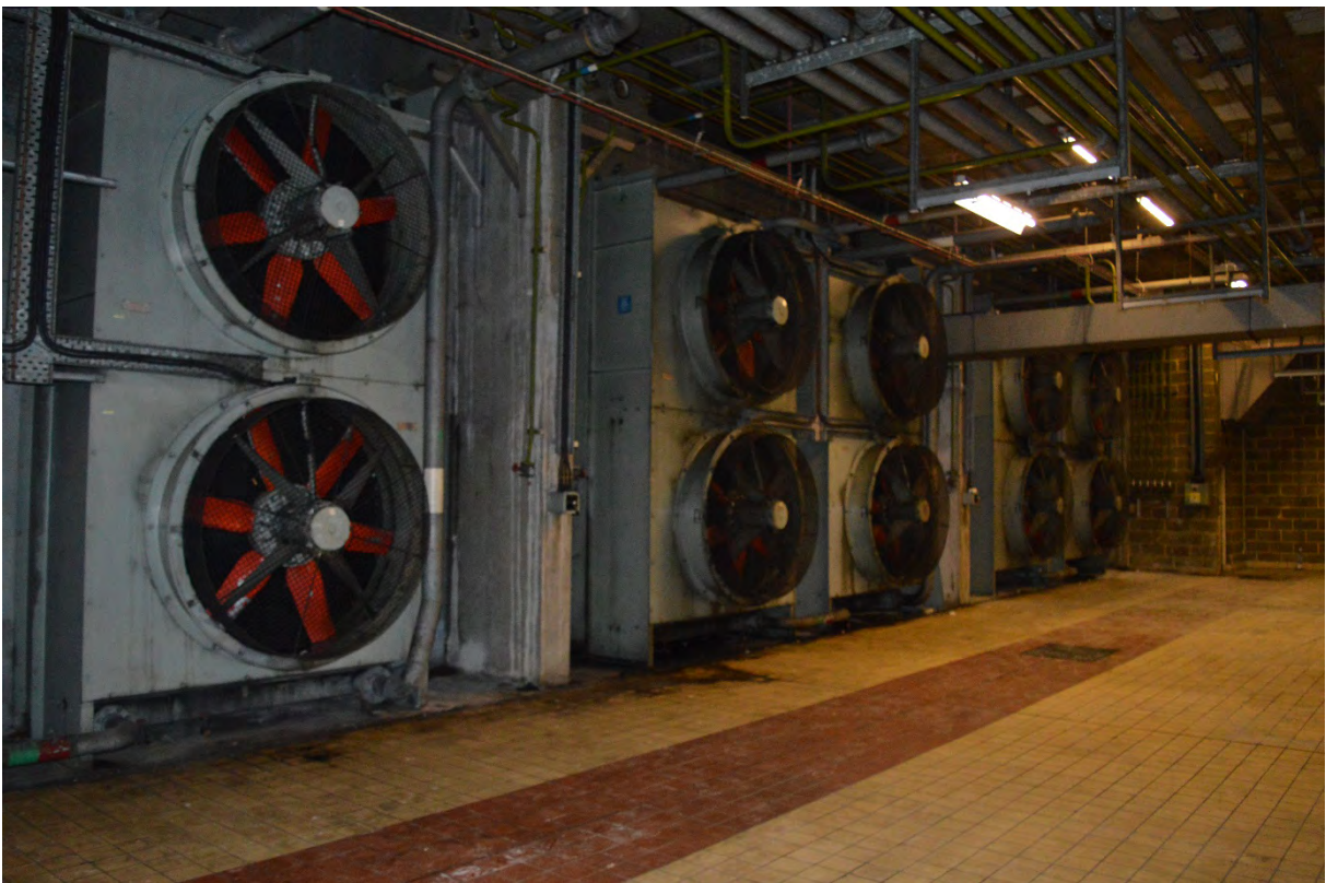
Plate 22: Extractor fans on west wall of sub-basement (56)
