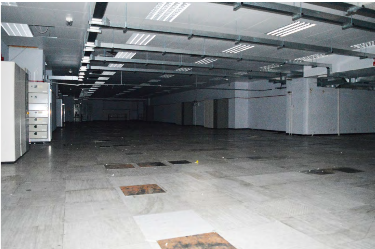
Plate 12: Ground floor data centre, with metal plates in floor marking cable inlets (171)
