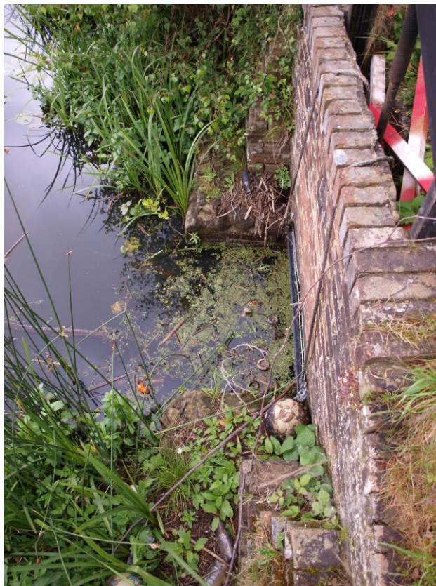
Plate 8 – Detail of head race Penstock, showing earlier sandstone foundations to later brick culvert
