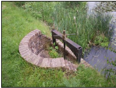
6621-0019 Penstock. Facing southeast
