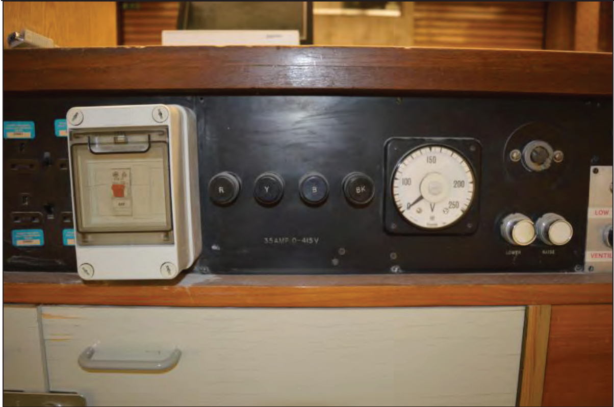
Plate 39. Shawcross Building, Lecture Theatre AS02, detail of sound operation switches, facing W (7499-0039)
