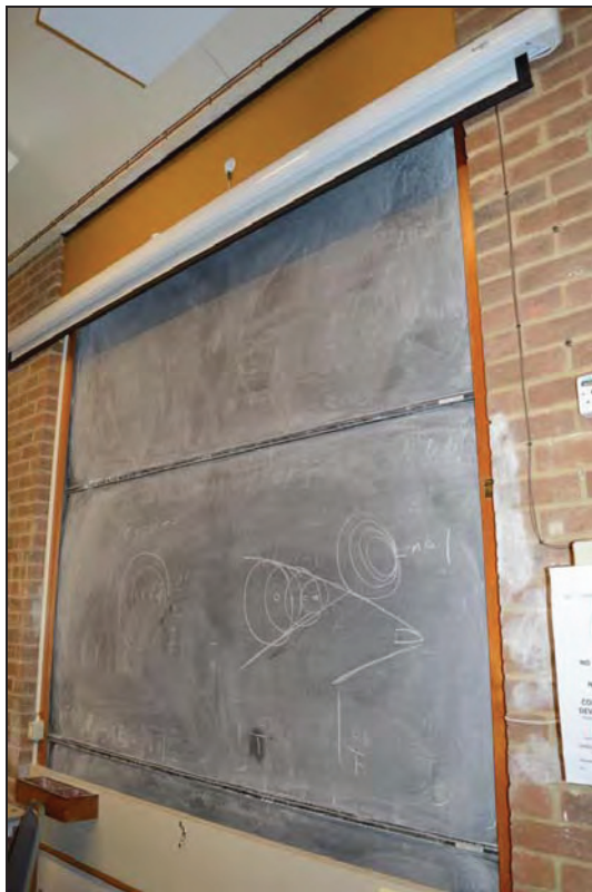
Plate 76. Arts A Building, Lecture Theatre A103, detail of blackboard and motorised projector screen above, facing NE (7499-0076)
