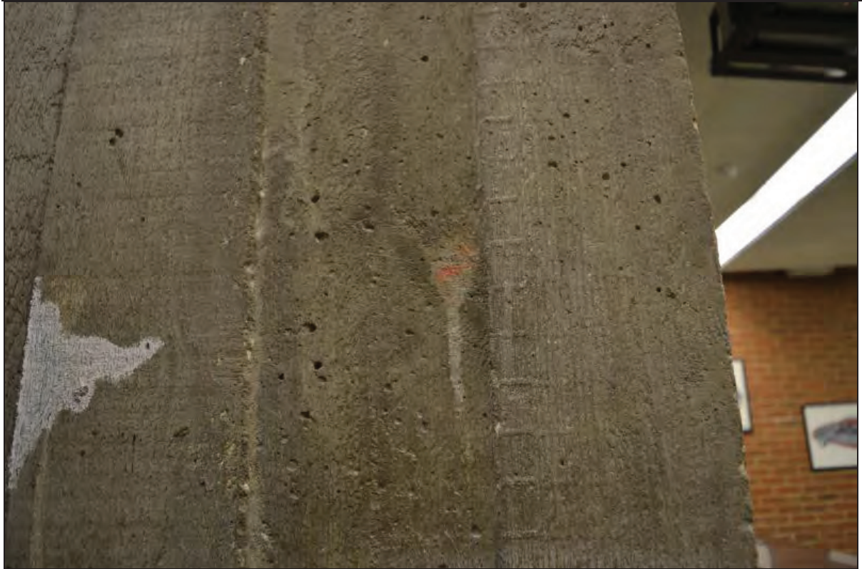
Plate 33. Shawcross Building, Lecture Theatre AS02, detail of bare-wood cast concrete finish of projector control room, facing N (7499-0033)
