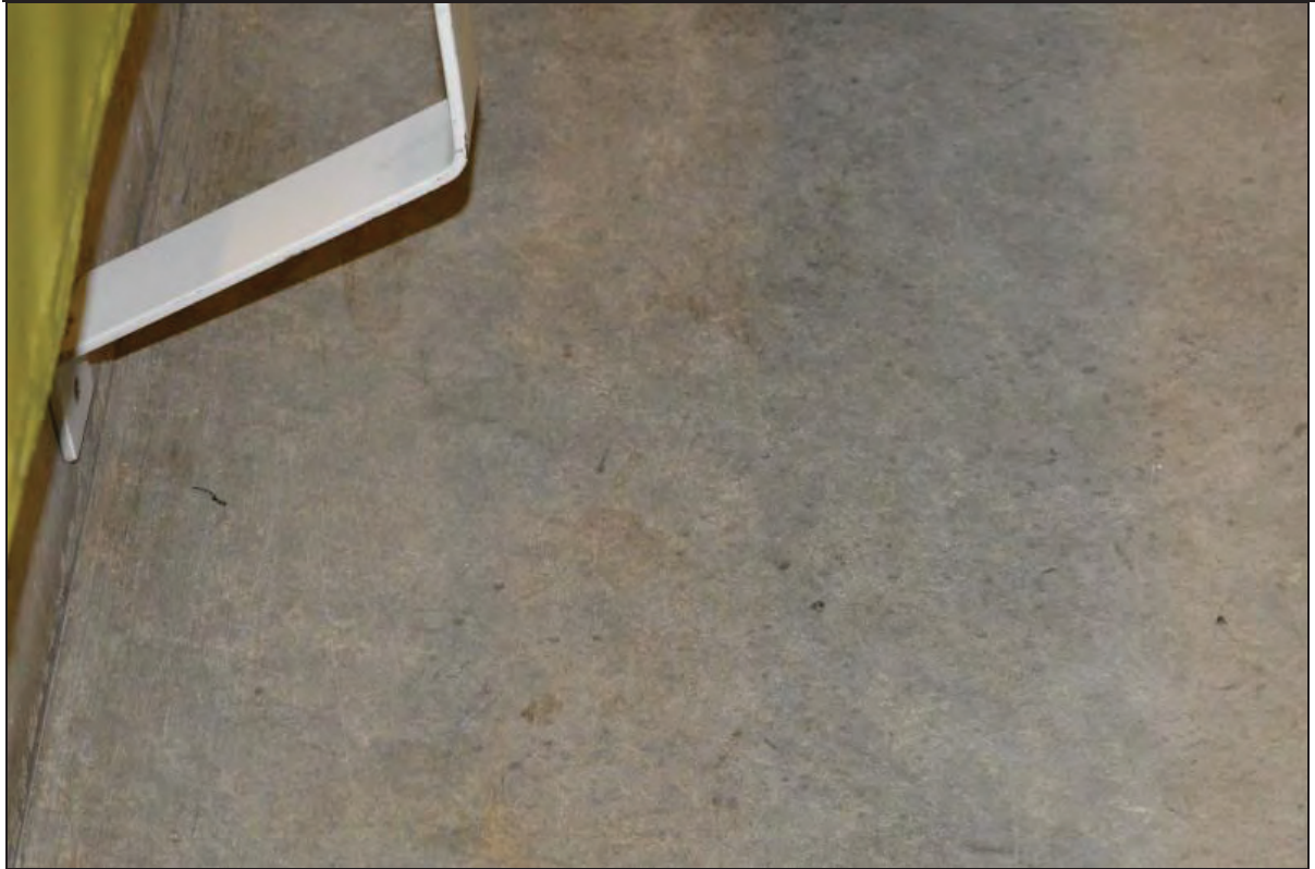
Plate 93. Arts A Building, Lecture Theatre A05, detail of modern linoleum floor covering under seating, facing N (7499-0093)
