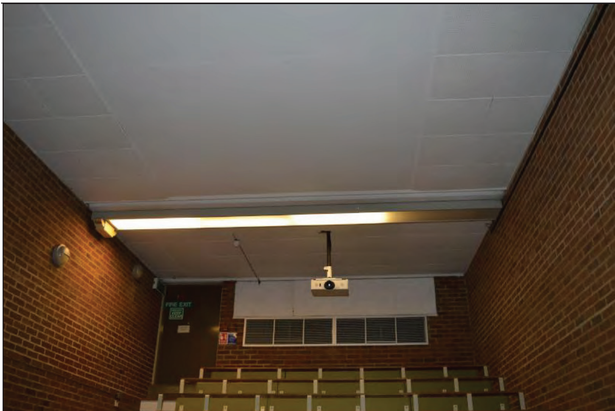
Plate 89. Arts A Building, Lecture Theatre A05, view of fibreboard ceiling and strip lighting, facing W (7499-0089)
