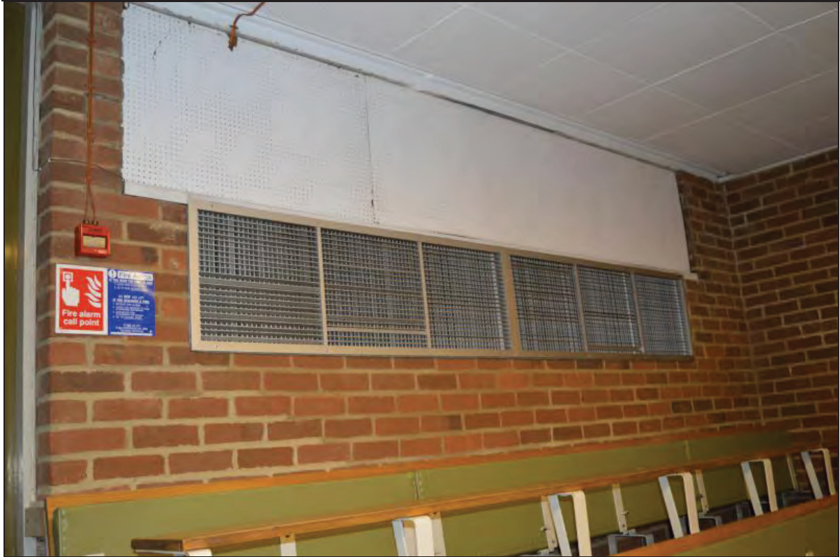
Plate 101. Arts A Building, Lecture Theatre A05, view of rear wall and ventilation grille, facing W (7499-0101)
