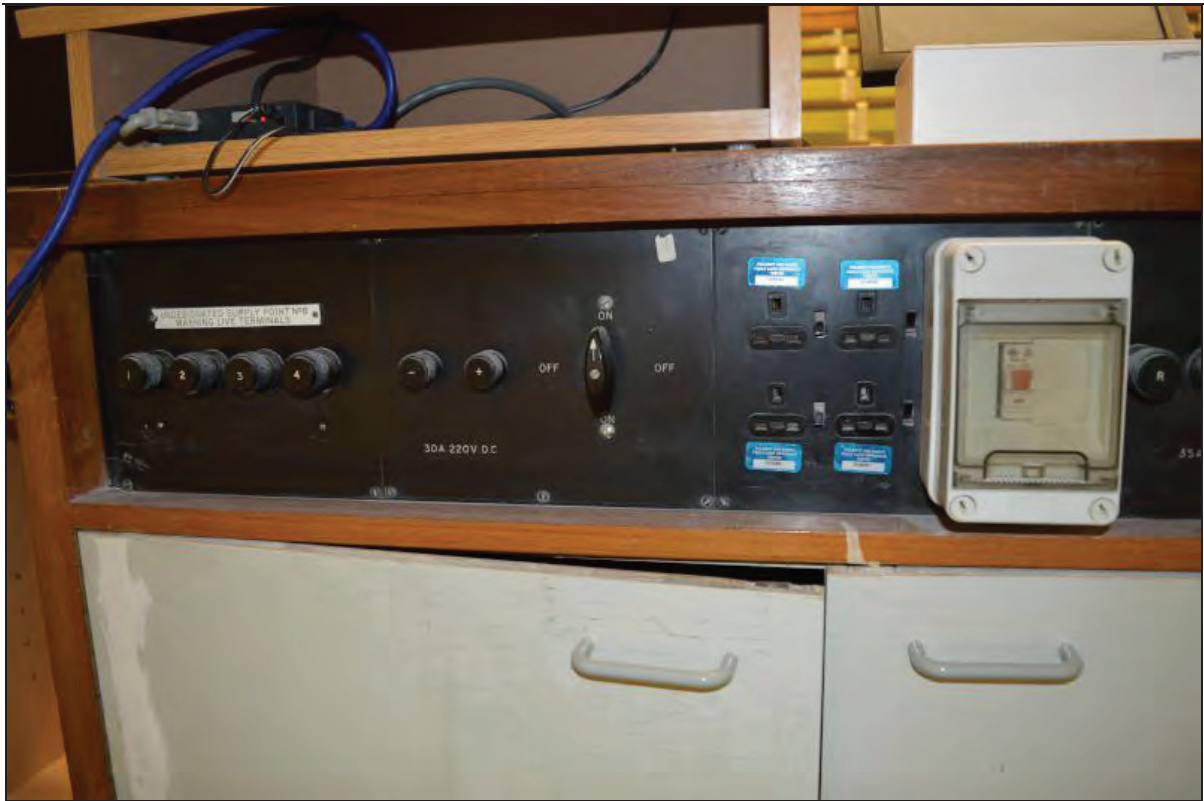
Plate 13. Shawcross Building, Lecture Theatre AS01, detail of projector switches, facing E (7499-0013)
