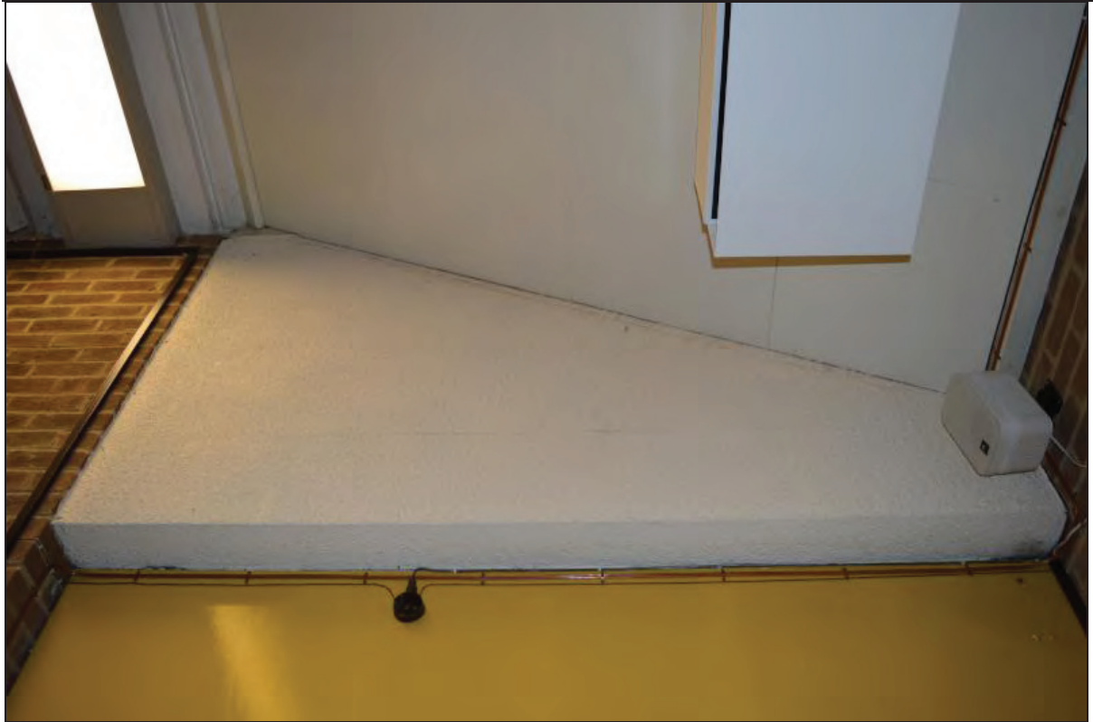
Plate 79. Arts A Building, Lecture Theatre A103, detail of concrete wall cover above external door and slanted ceiling arrangement, facing N (7499-0079)
