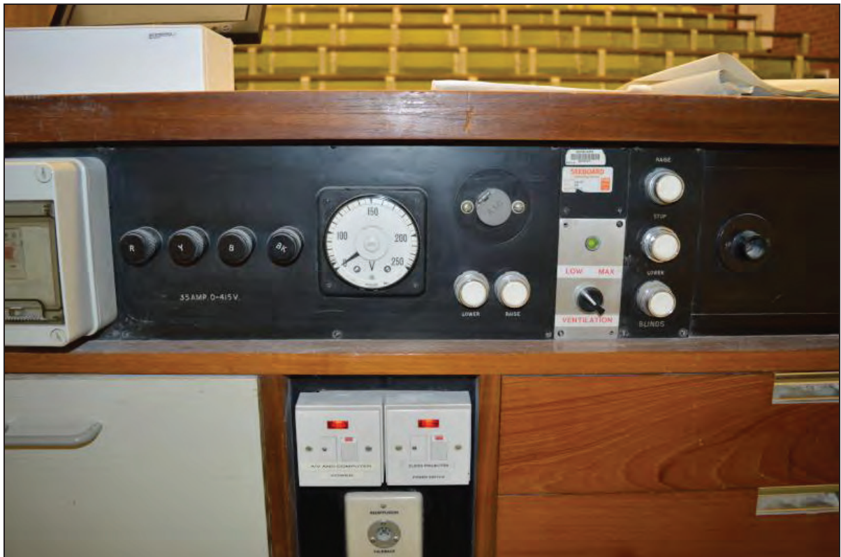
Plate 12. Shawcross Building, Lecture Theatre AS01, detail of sound/lighting operation switches, facing E (7499-0012)
