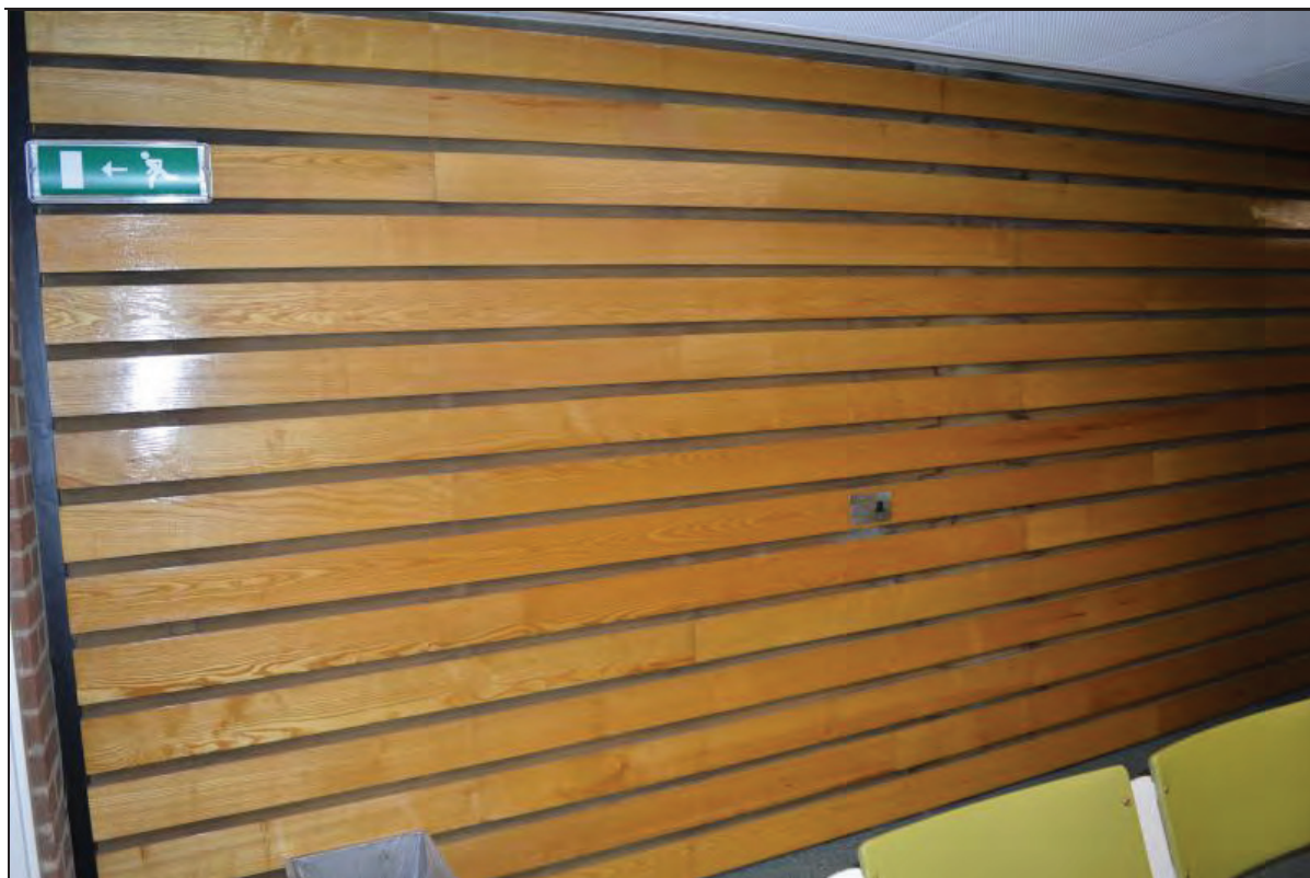
Plate 45. Shawcross Building, Lecture Theatre AS02, detail of horizontal timber clad rear wall finish, facing NW (7499-0045)
