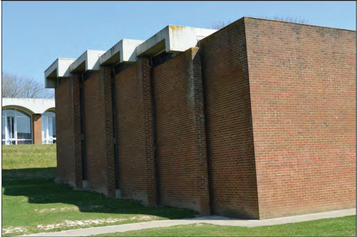
Plate 145. Arts A Building, detail of western elevation of Grade II* main entrance, facing NE (7499-0145)
