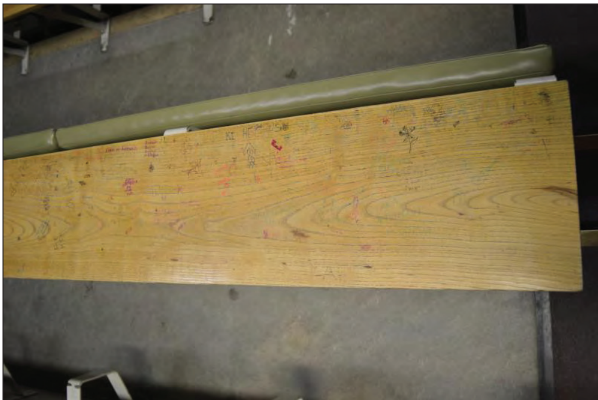
Plate 100. Arts A Building, Lecture Theatre A05, close-up of timber writing desk graffiti, facing N (7499-0100)
