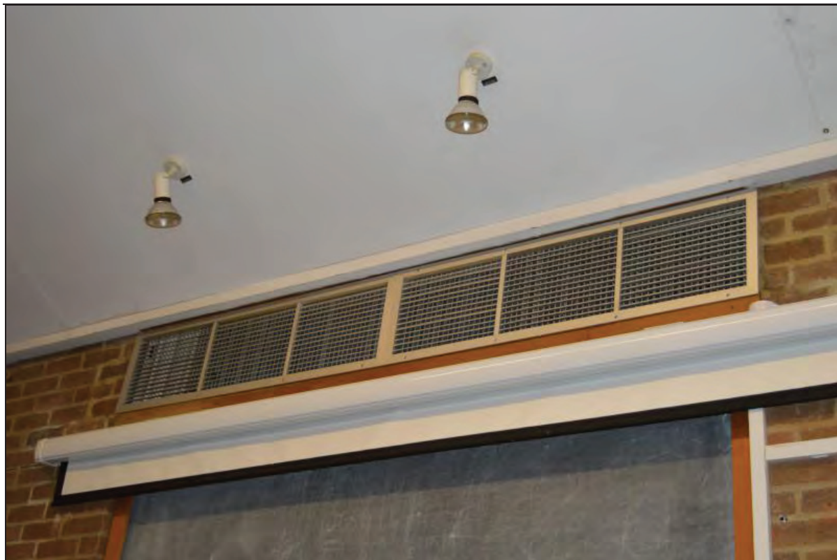
Plate 111. Arts A Building, Lecture Theatre A05, detail of modern plasterboard ceiling, spot lighting and ventilation grille, facing NE (7499-0111)
