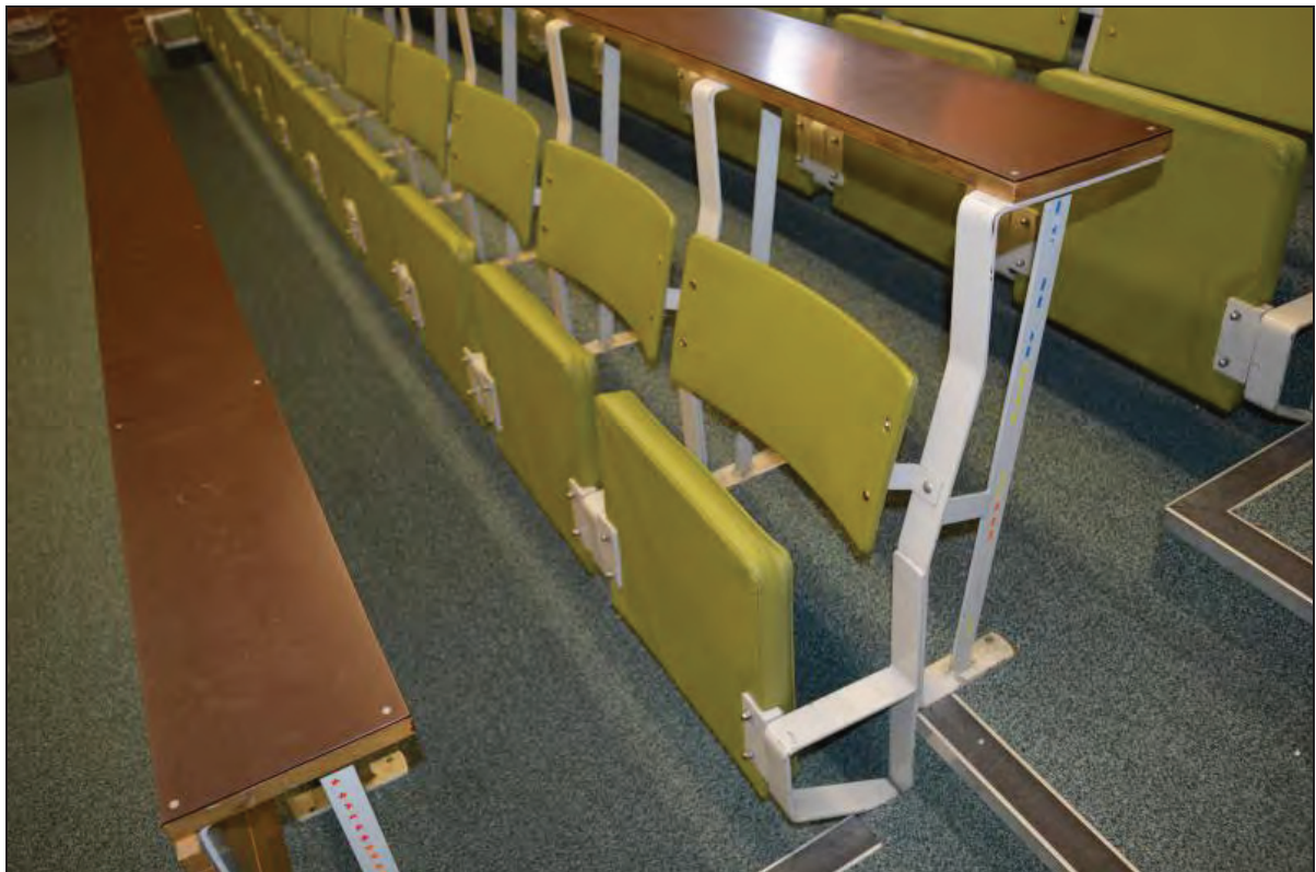
Plate 18. Shawcross Building, Lecture Theatre AS01, detail of tip-up seating and metal frame fixing, facing NE (7499-0018)
