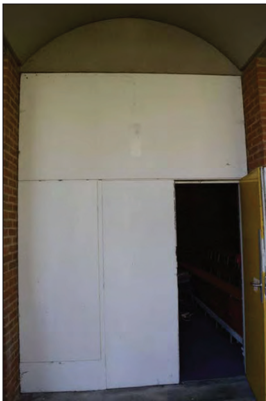
Plate 78. Arts A Building, Lecture Theatre A103, view of external access door, facing S (7499-0078)
