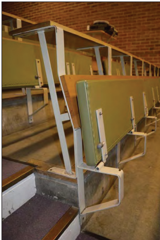
Plate 64. Arts A Building, Lecture Theatre A103, detail of metal frame fixing and concrete tiered floor, facing NW (7499-0064)
