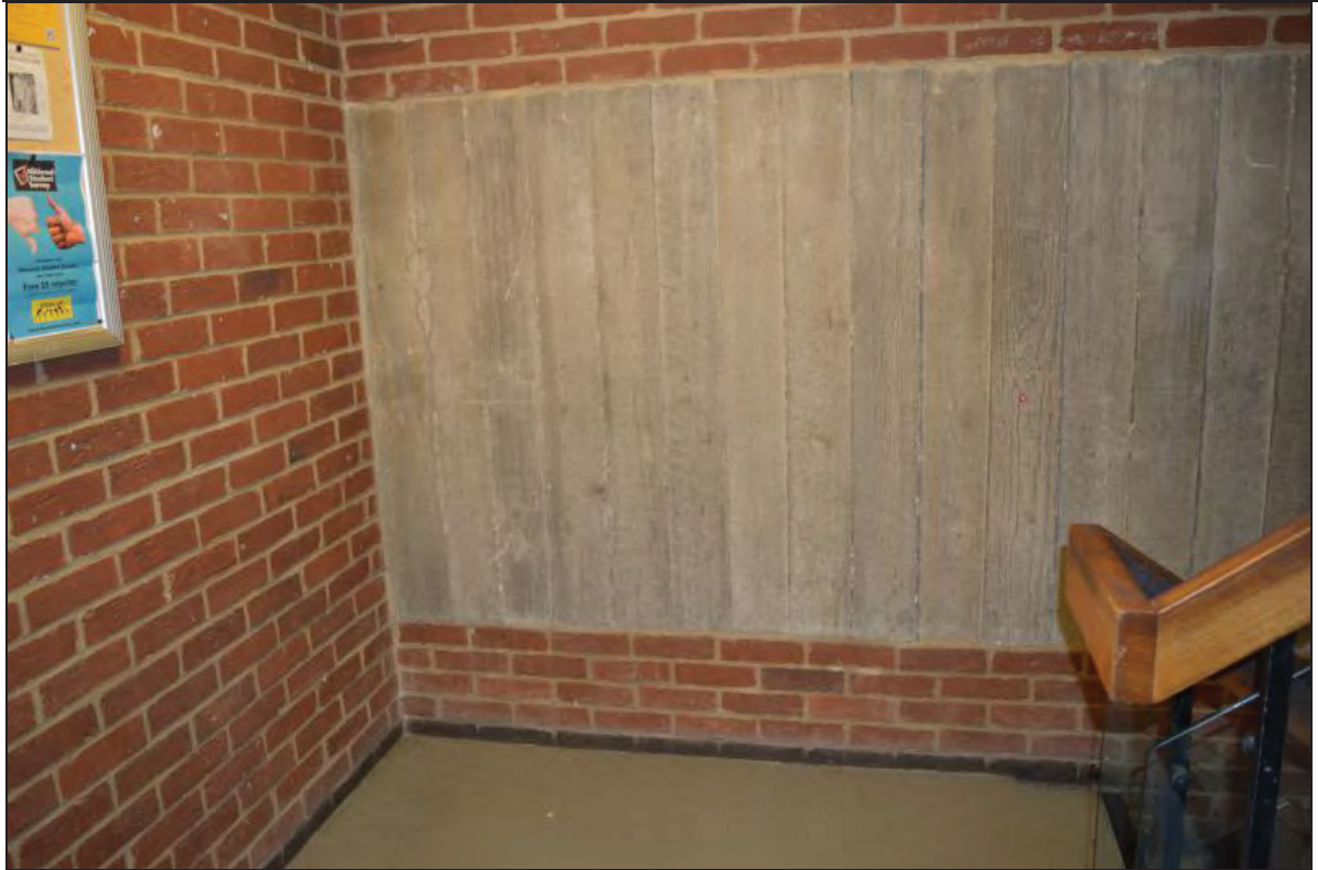
Plate 53. Shawcross Building, detail of bare-wood cast concrete wall finish opposite the south-west entrance to Theatre AS01, facing S (7499-0053)
