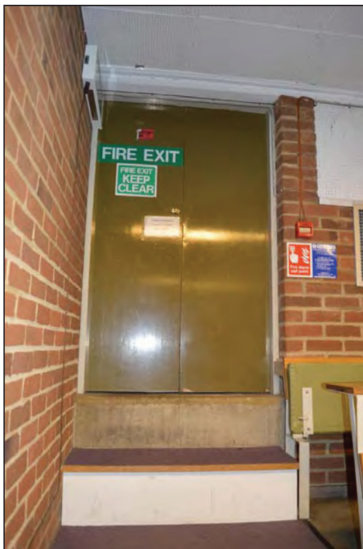
Plate 102. Arts A Building, Lecture Theatre A05, view of rear fire exit, facing W (7499-0102)
