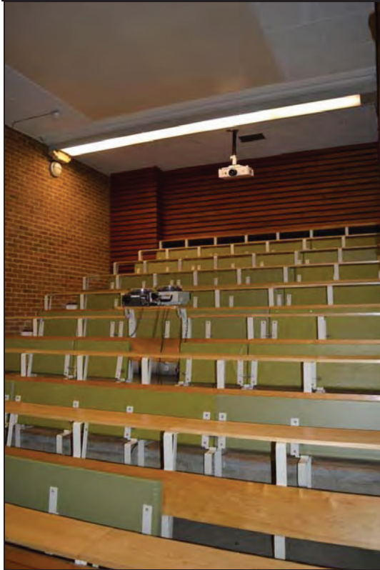
Plate 59. Arts A Building, Lecture Theatre A103, view of tiered seating and desk mounted projector, facing SW (7499-0059)
