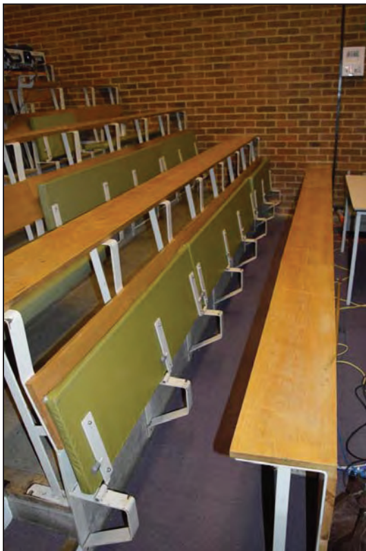
Plate 110. Arts A Building, Lecture Theatre A05, detail of tip-up bench arrangement and writing desk, facing NW (7499-0110)
