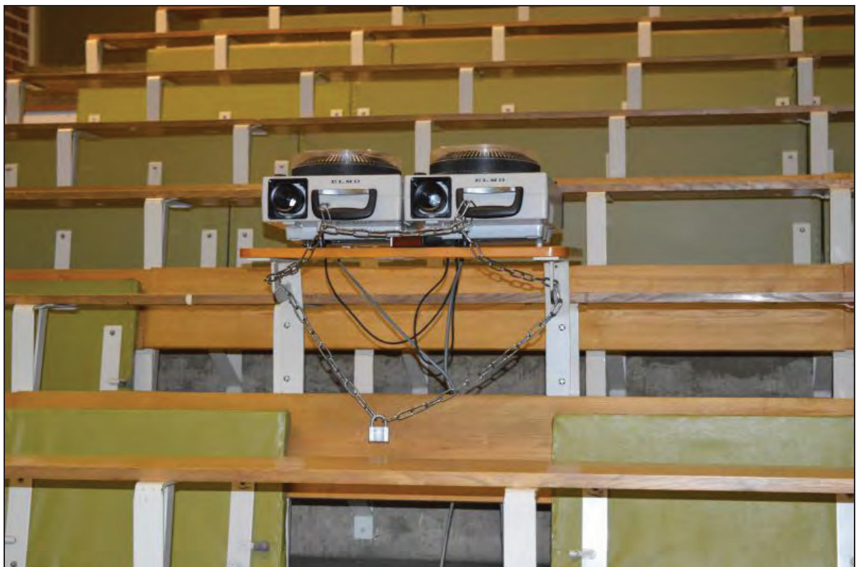
Plate 86. Arts A Building, Lecture Theatre A05, detail of desk mounted projector (note seat removal), facing W (7499-0086)
