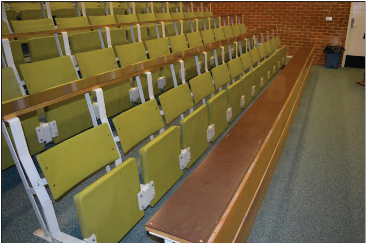
Plate 8. Shawcross Building, Lecture Theatre AS01, view of front row of seating and detail of timber modesty panel, facing SE (7499-0008)
