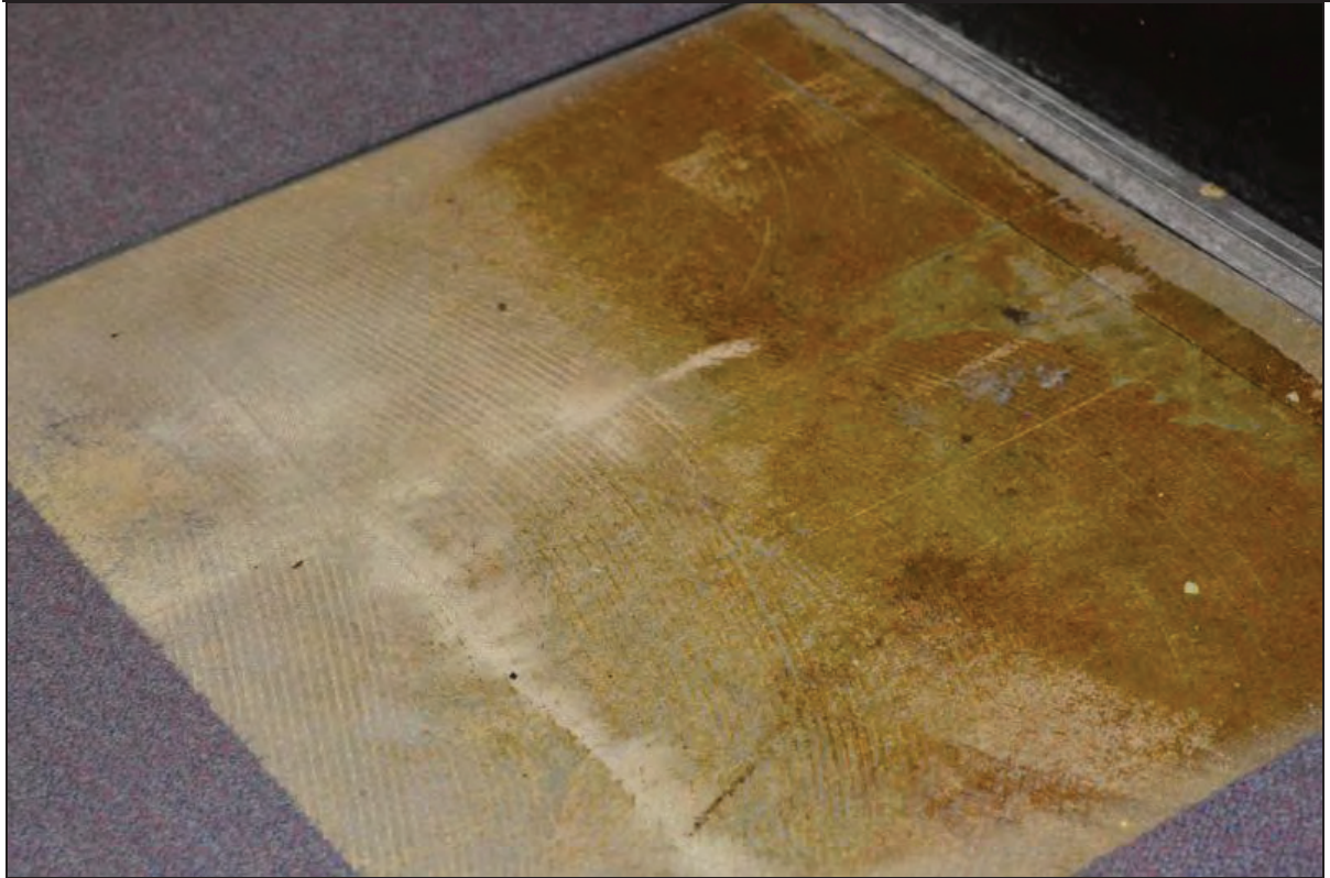
Plate 71. Arts A Building, Lecture Theatre A103, concrete floor covering under modern carpet tiles, facing SE (7499-0071)
