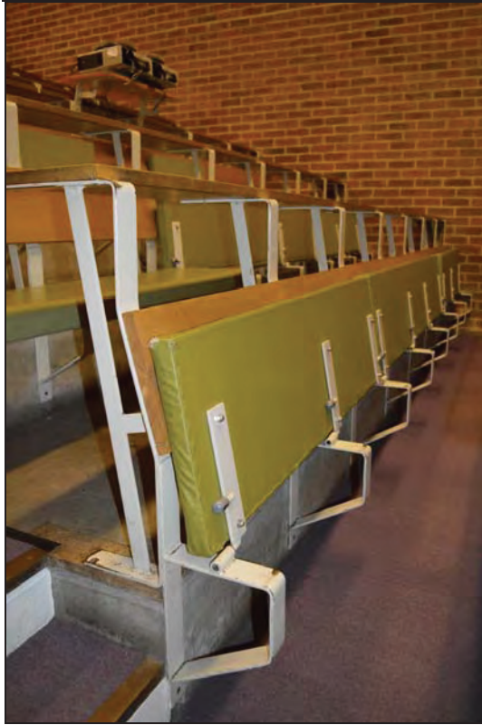
Plate 91. Arts A Building, Lecture Theatre A05, detail of tiered tip-up benches and metal frame, facing NW (7499-0091)
