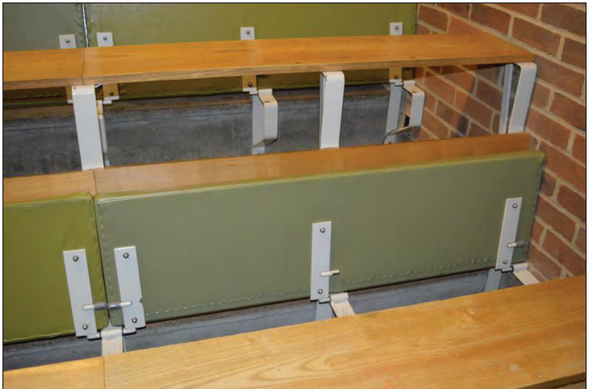
Plate 88. Arts A Building, Lecture Theatre A05, detail of metal tip-up bench supports, facing W (7499-0088)
