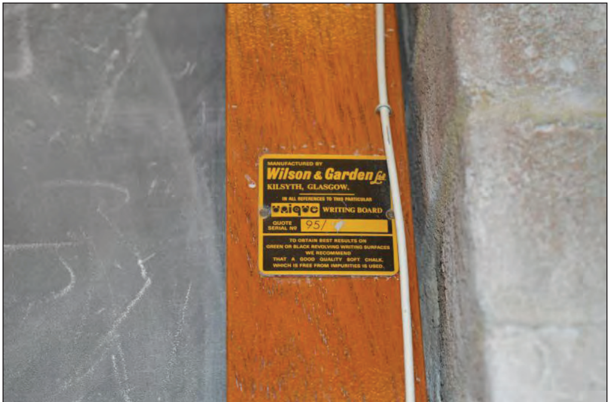
Plate 74. Arts A Building, Lecture Theatre A103, makers mark of roller section blackboard ('Wilson & Garden), facing E (7499-0074)
