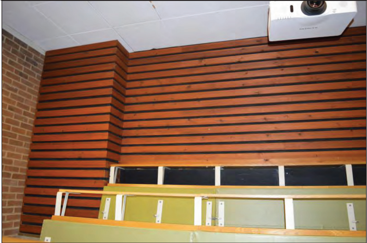
Plate 65. Arts A Building, Lecture Theatre A103, rear horizontal timber clad wall covering with ground-level ventilation ducts, facing W (7499-0065)
