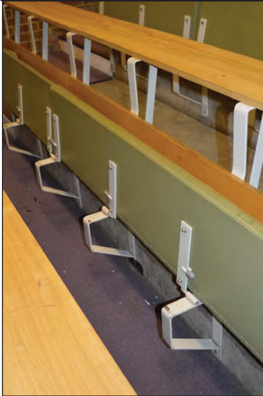
Plate 81. Arts A Building, Lecture Theatre A103, detail of tip-up bench supports, facing SW (7499-0081)
