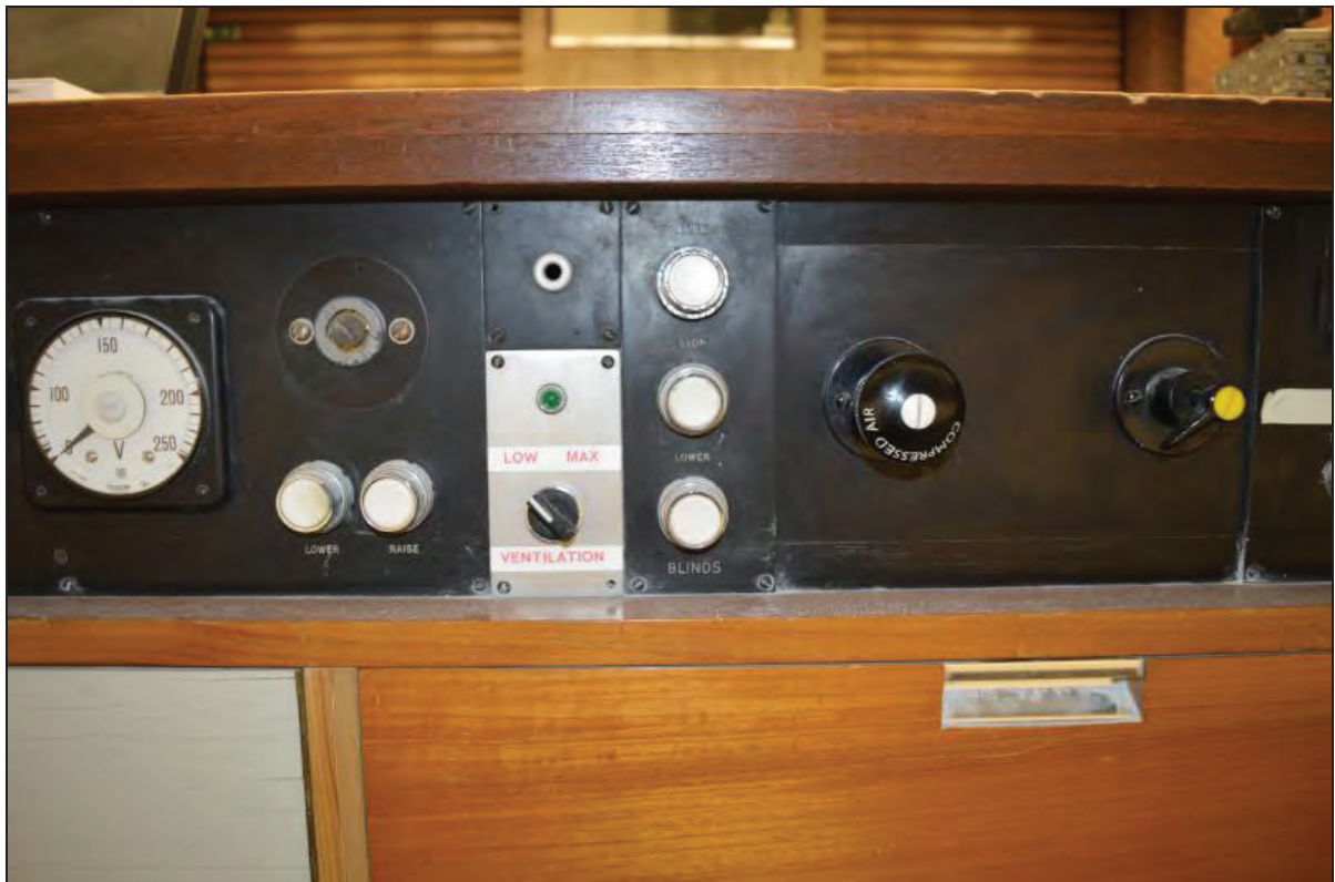
Plate 40. Shawcross Building, Lecture Theatre AS02, detail of sound/lighting/projector operation switches, facing W (7499-0040)
