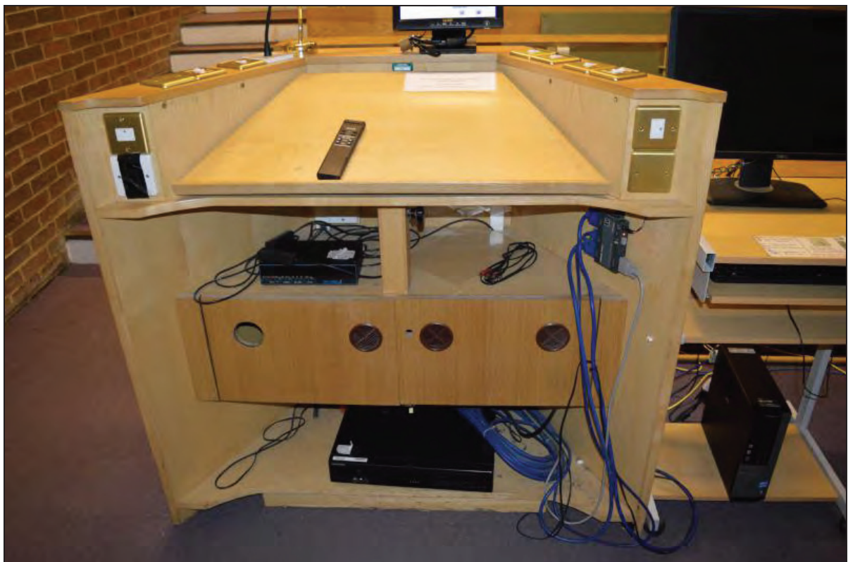
Plate 114. Arts A Building, Lecture Theatre A05, detail of sound/lighting equipment and operation switches, facing W (7499-0114)
