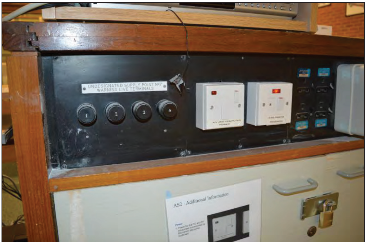
Plate 38. Shawcross Building, Lecture Theatre AS02, detail of lighting/projector operation switches, facing W (7499-0038)
