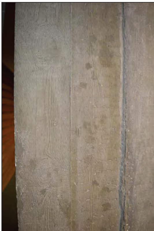
Plate 32. Shawcross Building, Lecture Theatre AS02, detail of bare-wood cast concrete finish of projector control room, facing N (7499-0032)
