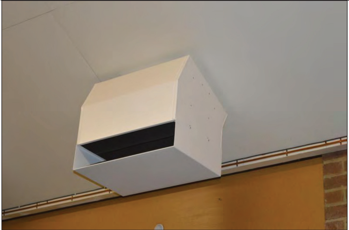
Plate 73. Arts A Building, Lecture Theatre A103, close-up of ceiling ventilation ducts, facing NE (7499-0073)
