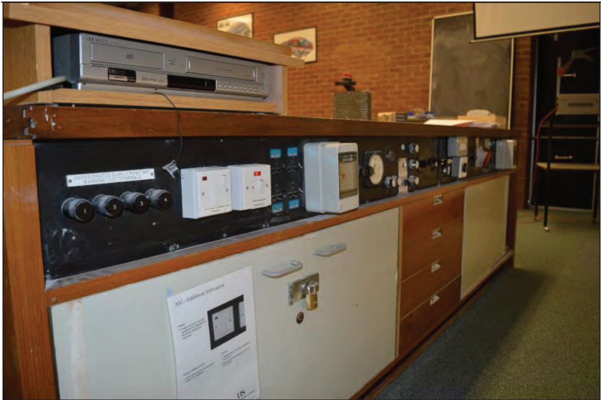
Plate 37. Shawcross Building, Lecture Theatre AS02, detail of sound/lighting/projector operation switches, facing NW (7499-0037)
