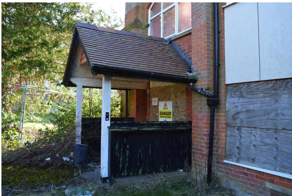
Plate 20: Building 6, detail of porch situated to the southern end of the east elevation, facing south-west (7335_0051)
