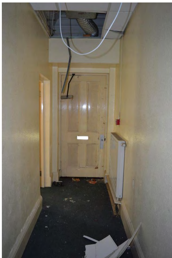
Plate 37: Building 9, ground floor, current entrance located to the south-west wall, facing south-west (7335_0141)
