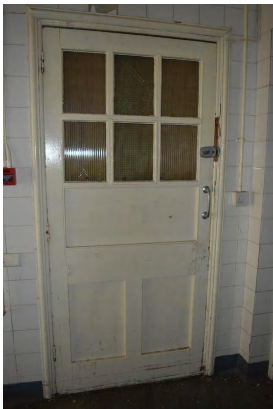
Plate 11: Building 5, ground floor, detail of external door to western range, providing access to Room 9, facing south (7335_0103)
