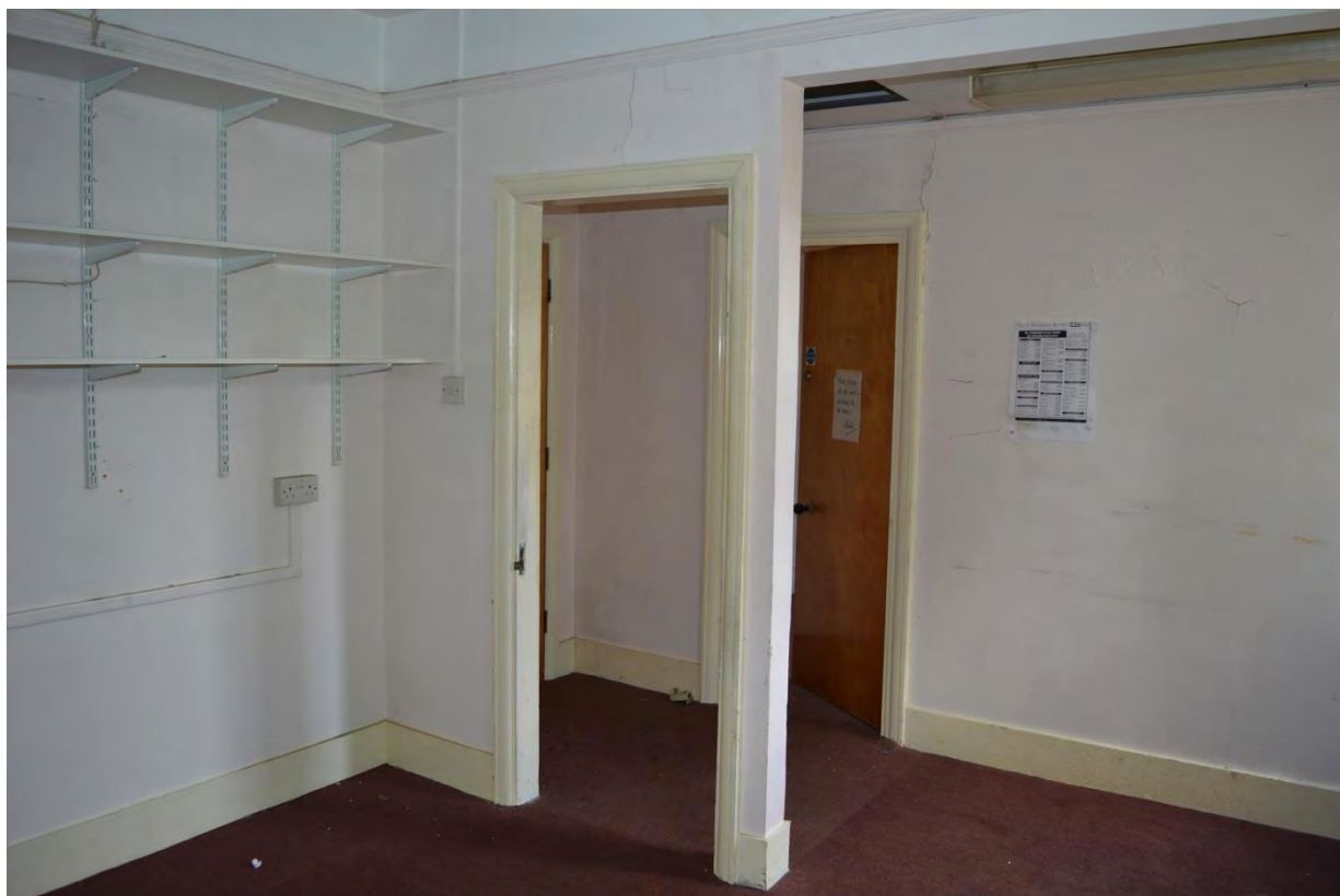
Plate 73: Building 11, ground floor, redundant door fitting resulting from internal alteration, facing north-west (7335_0083)
