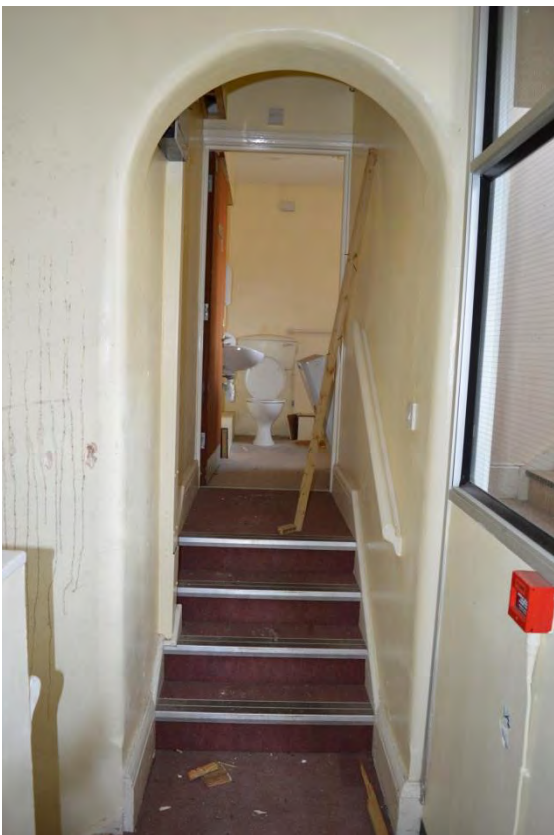
Plate 46: Building 9, first floor, lower landing layout and Room 12 arched entrance, facing north-east (7335_0164)
