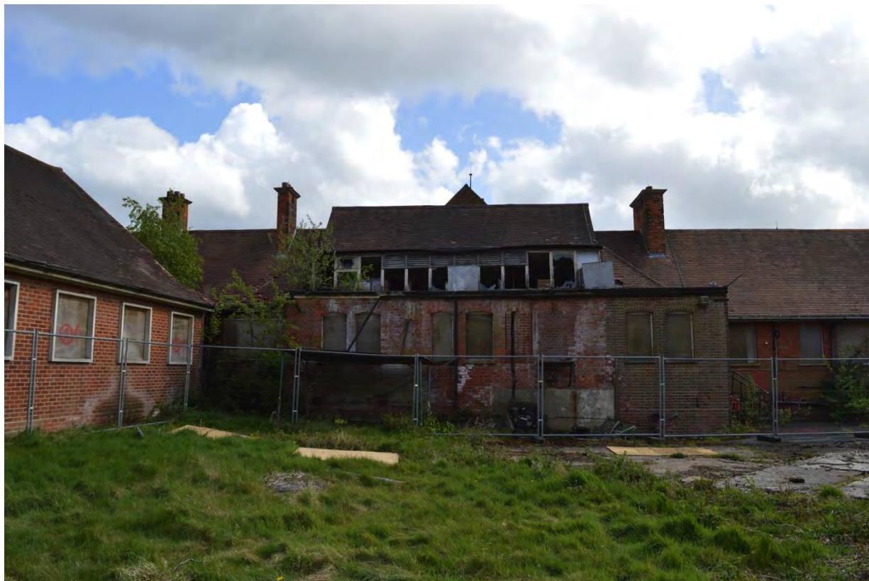
Plate 5: Building 5, view of the north elevation of the central block, facing south (7335_0177)
