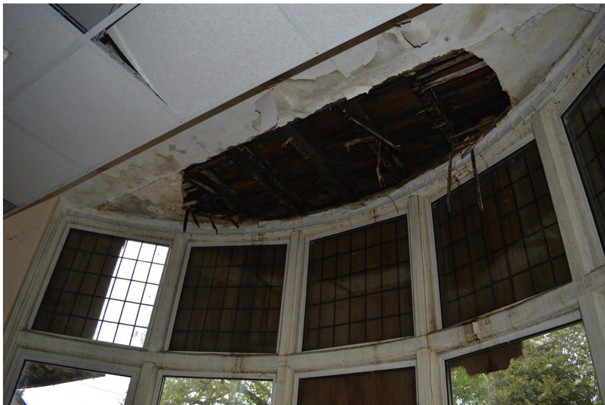
Plate 59: Building 10, ground floor, detail of lath and plaster ceiling within Room 3, facing north-east (7335_0058)
