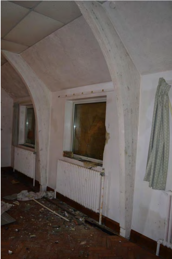
Plate 9: Building 5, ground floor, Room 7, detail of bay and concrete truss arrangement, facing south-west (7335_0096)
