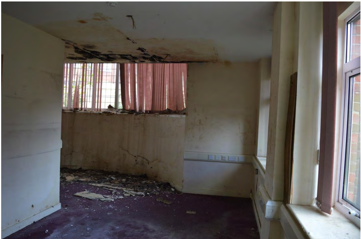
Plate 22: Building 6, ground floor, sub-divided office space to the southern end, facing south (7335_0133)
