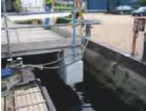
1. Detailed Survey 12, Chainage 105 Wood Wharf 1 – WWS1 (3) Change from Sheet Piles to Brick work
