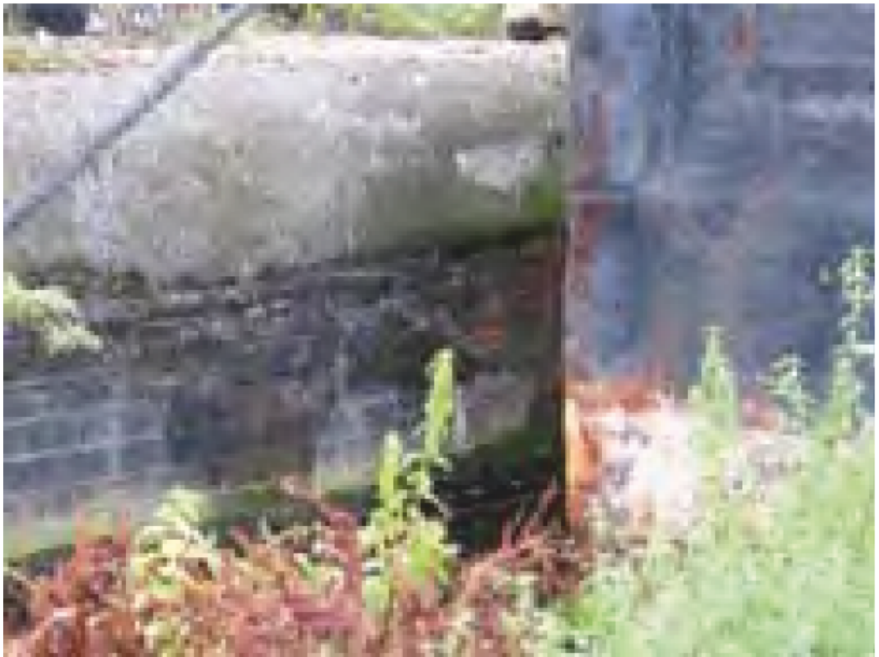
Plate 9: 'Blue' brick refacing and concrete capping to the south side of the Export Dock
