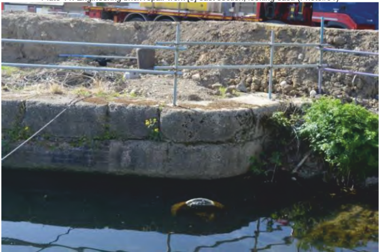
Plate 12: Concrete wall section [4] to east of former Junction Dock entrance. Looking southeast. (Photo#16)
