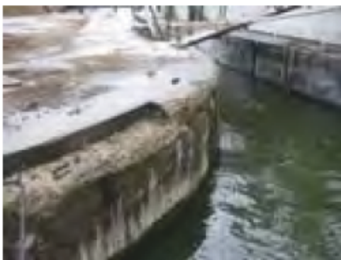
5. Detailed Survey 16, Chainage 8 Wood Wharf 2 – WWS2 (4) Change from Brickwork to Concrete 520 – ARUP – Wood Wharf Dock Survey
