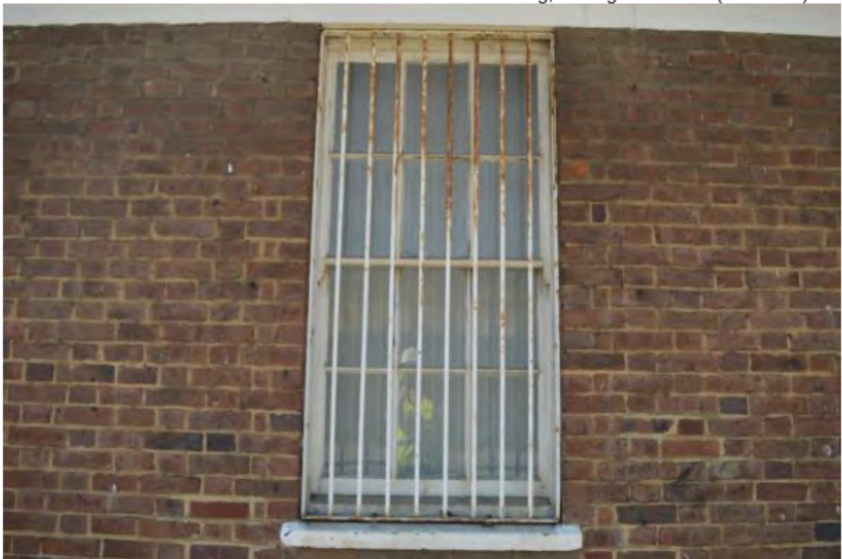
Plate 40: Sash window protected by iron bars in the north elevation of the Canal and River Trust Building. Looking south. (Photo#26)
