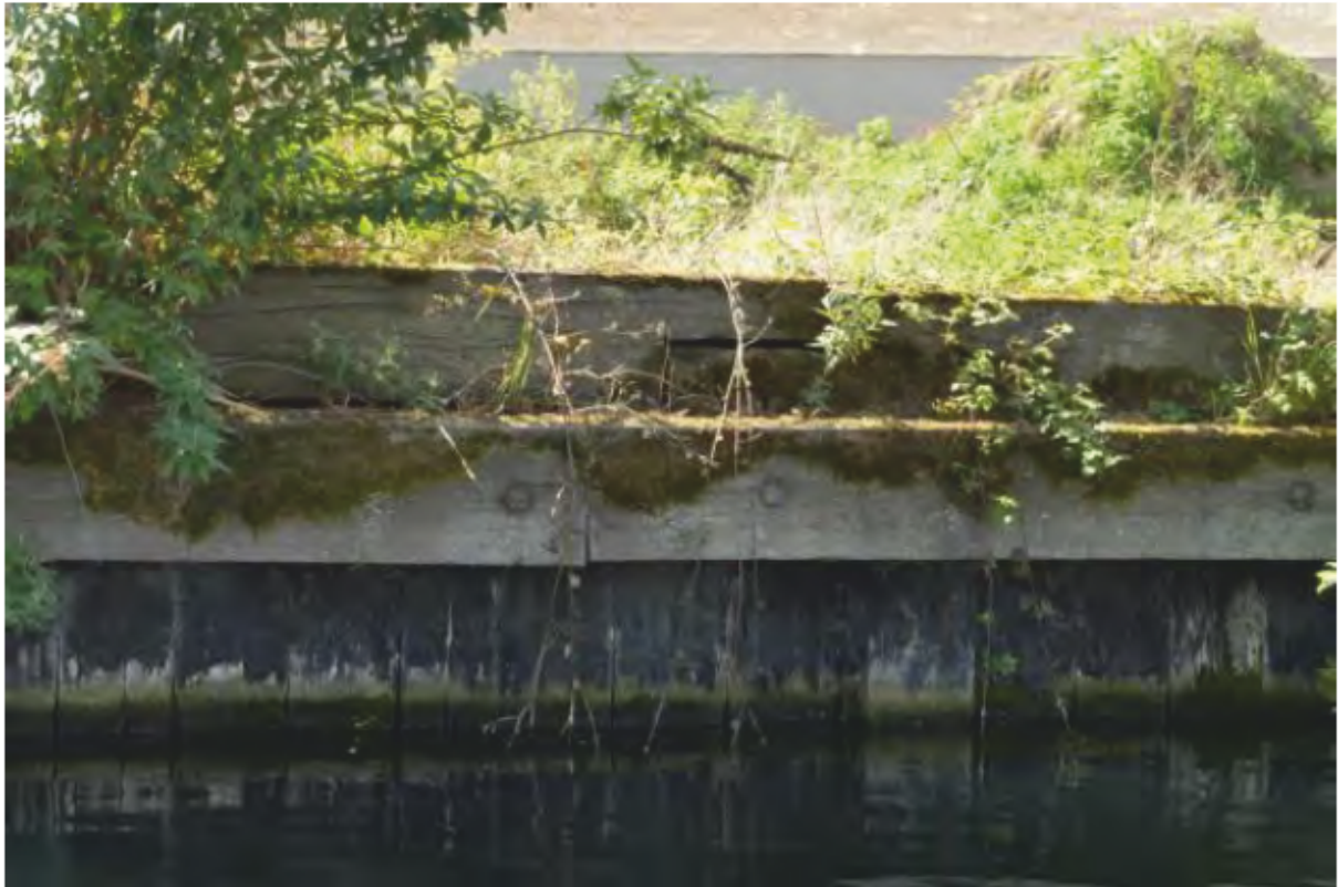
Plate 7: Curtain joint in the timber capping beam [2]. Looking south. (Photo#80)
