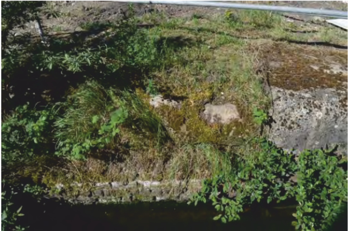
Plate 15: Mid-19 th -century brickwork to west of the former Junction Dock [6]. Looking south. (Photo#18)
