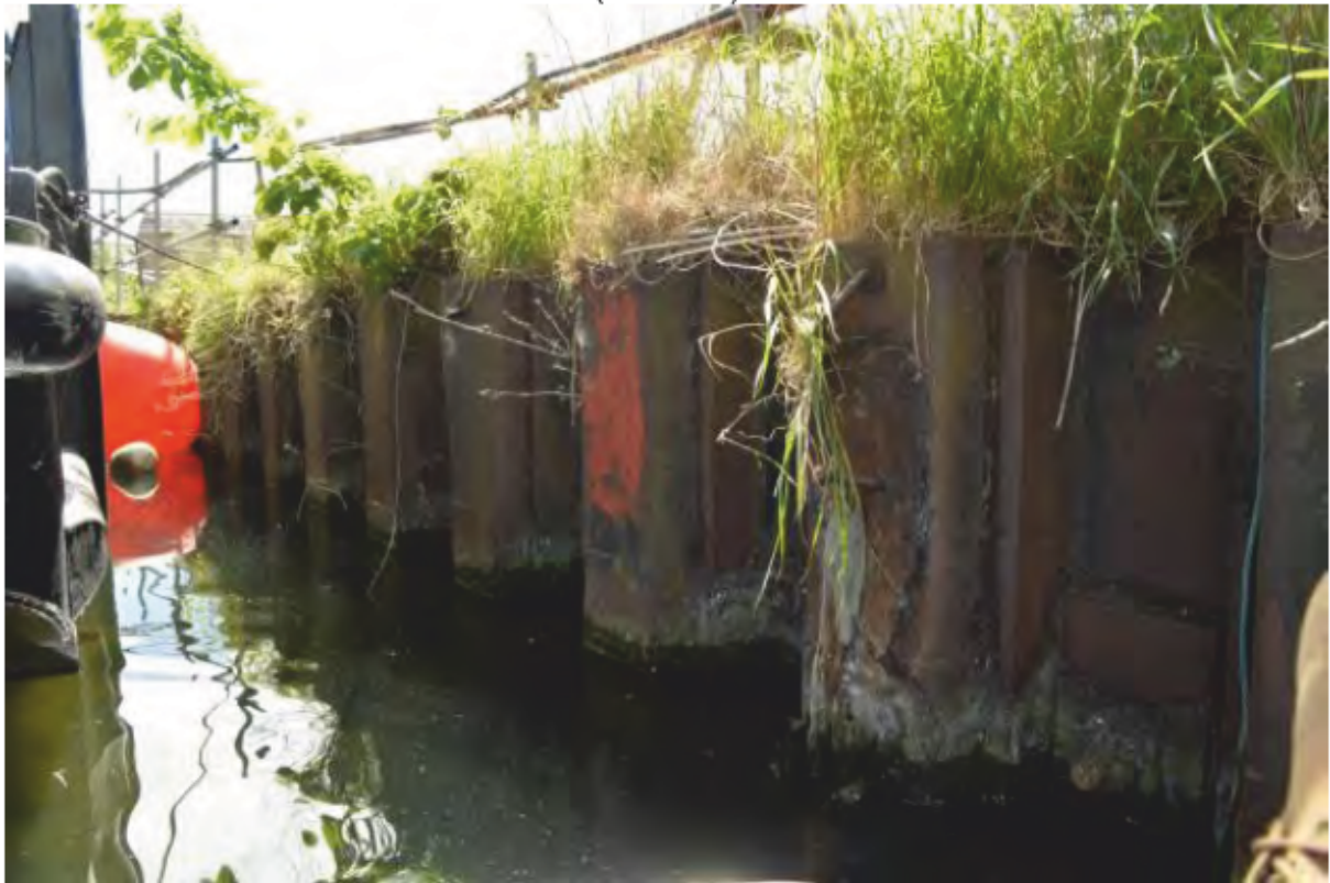
Plate 16: Larssen sheet pile wall section [7]. Note remnant timber revetment. Looking east. (Photo#95)
