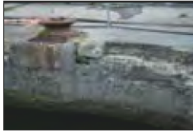
7525-0149 7525_West India Dock_South Dock_North Wall_Exposed Granite Coping in North East Corner of the South Dock. Facing north
