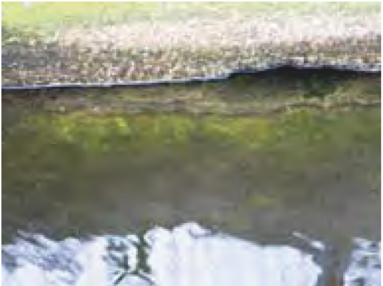
Plate 3: Concrete walls of the canal to the Import Dock extending below the water line
