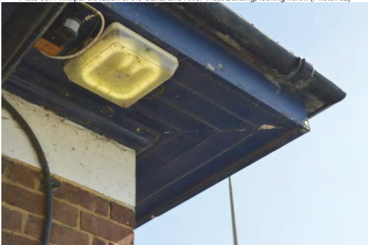
Plate 34: Canal and River Trust Building wooden soffit, fascia, and moulded cornice, looking northeast. (Photo#50)
