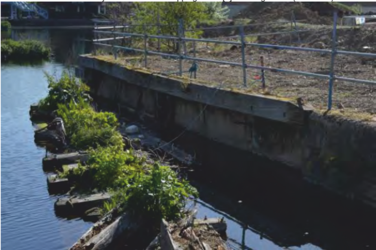
Plate 8: Exposed concrete behind the collapsed timber revetment [2]. (Photo#14)
