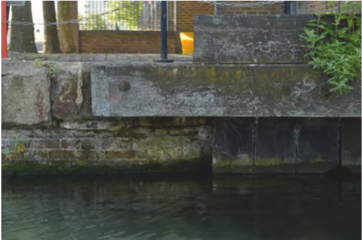
Plate 3: 1878 wall section [1] and later timber revetted wall intersection. (Photo#78)
