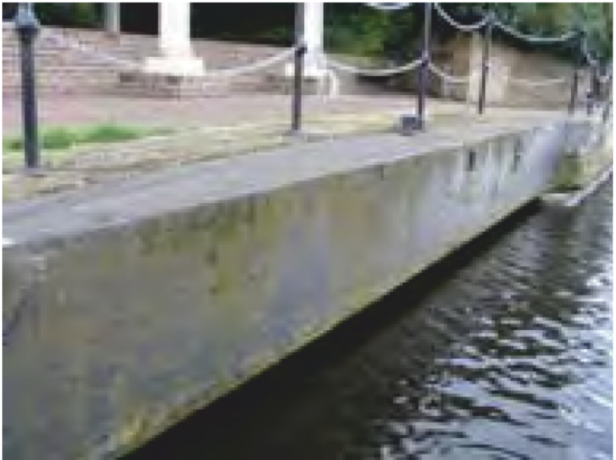
Plate 5: Surviving part of the swing bridge at the entrance to poplar dock
