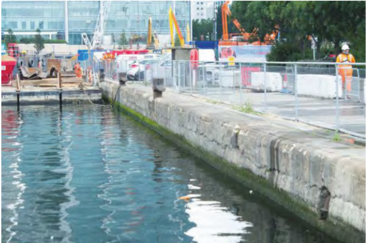
Plate 31: Eastern section of the North Wall of the South Dock, looking west. (Photo#151)
