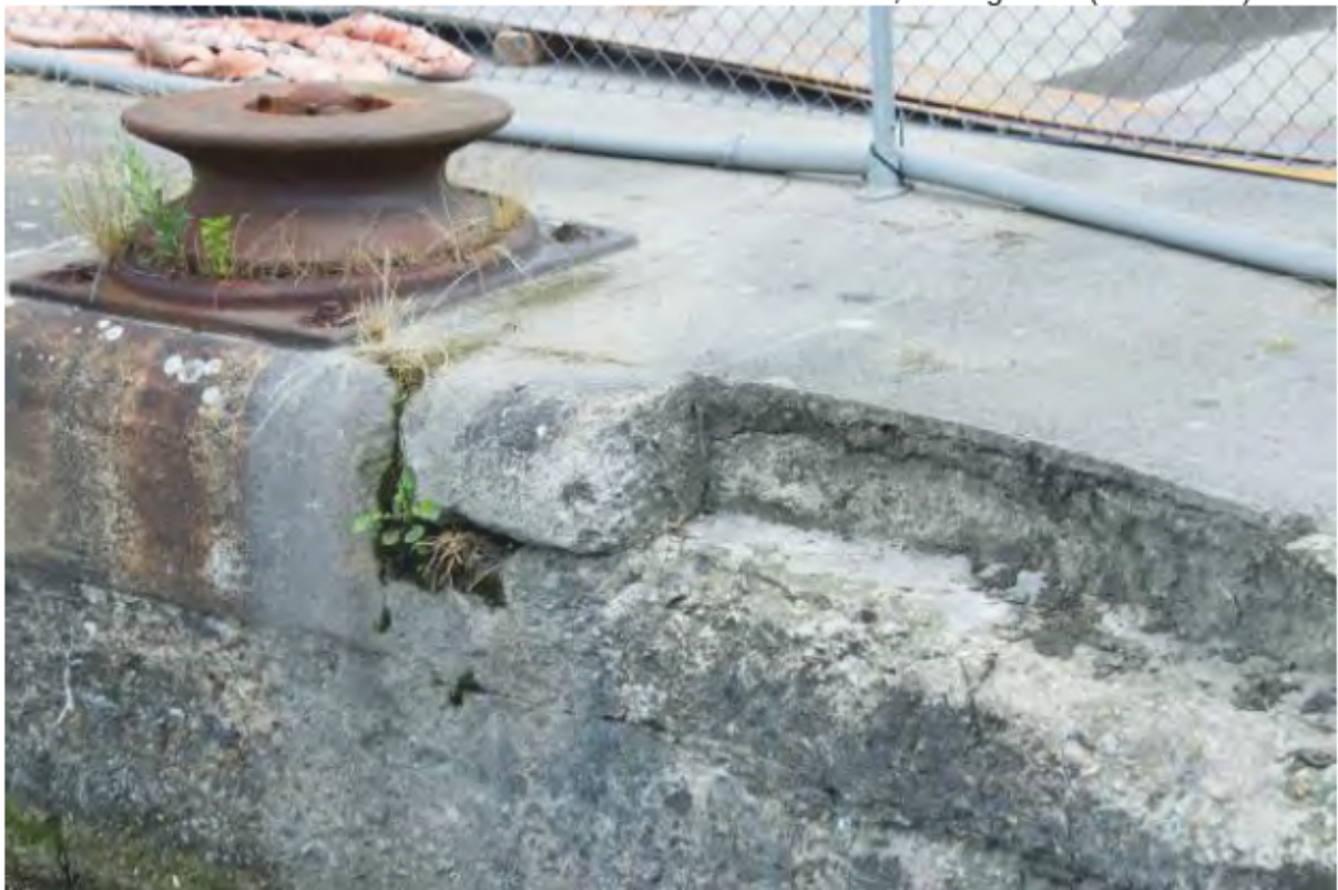
Plate 32: Extant granite coping at the east end of the North Wall of the South Dock. Note the single-bitt mooring bollard. Looking northwest. (Photo#150)
