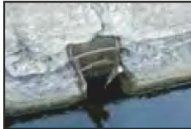
7525-0152 7525_West India Dock_South Dock_East Wall_Ladder set in Aggregate Concrete Below Granite Coping. Facing east
