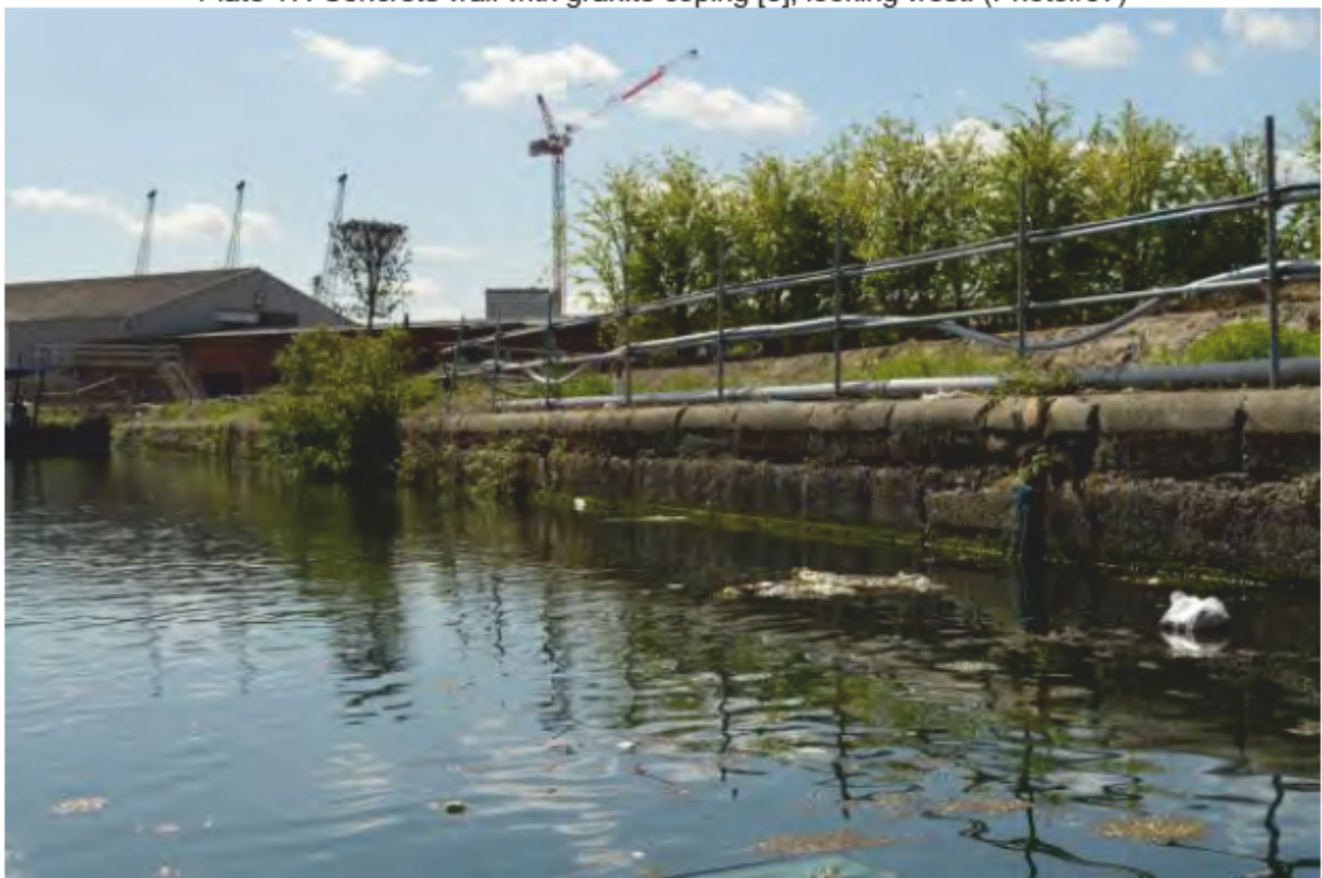
Plate 18: Concrete wall with granite coping [8], looking east. Note the ladder recess to the right of the photo. (Photo#106)
