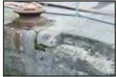
7525-0150 7525_West India Dock_South Dock_North Wall_Exposed Granite Coping in North East Corner of the South Dock. Facing north
