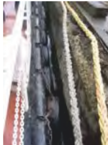
4. Detail Survey 15, Chainage 15 Wood Wharf 2 – WWS2 (3) Defect in Wall
