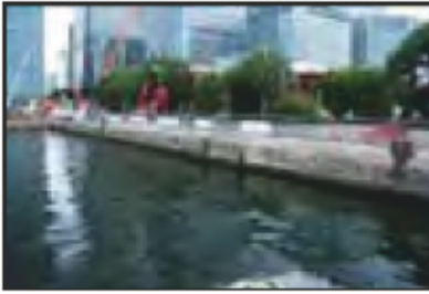
7525-0148 7525_West India Dock_South Dock_North Wall_Note Concrete Parged Coping atop Large Aggregate Concrete Wall Material. Facing north-west
