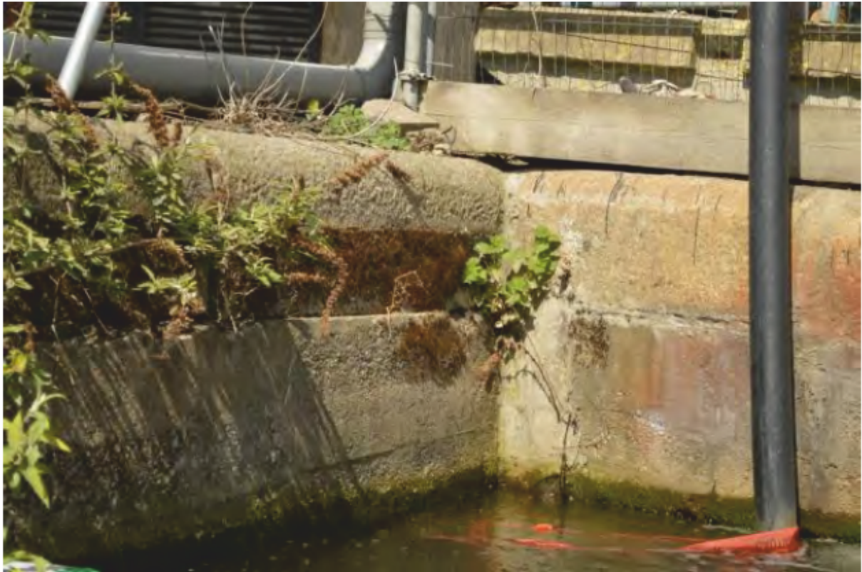
Plate 19: Interface of the 1927-29 concrete wall [8] with the likely original brick quay wall at the west end of the Blackwall Basin, looking west. (Photo#104)
