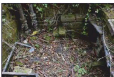
7494-0073 Combers Glasshouses - Building 1 - Pipes in east end of south lean-to. Facing south
