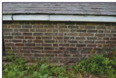
7494-0041 Combers Glasshouses - Building 4 - Joint in north elevation between east and west structures. Facing south
