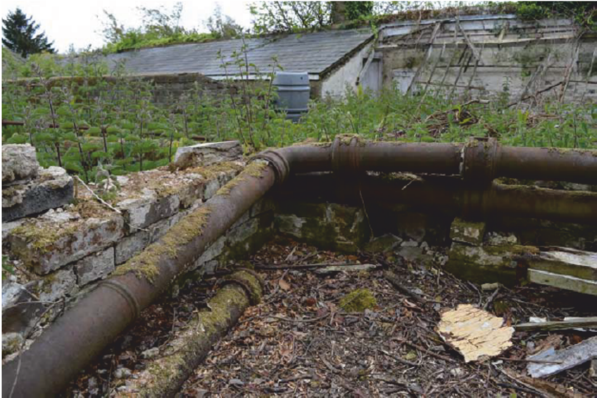
Plate 29: Building 2, heating pipes in Bay 1, looking south-east (Photo #13)
