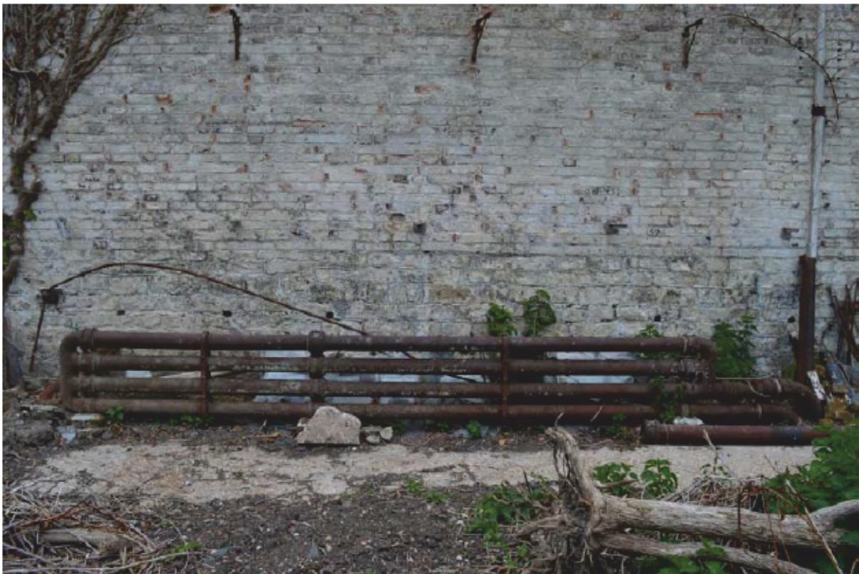
Plate 30: Building 2, four-tier pipe stack in Bay 2, looking north (Photo #19)
