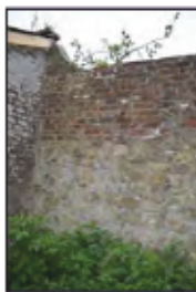
7494-0082 Combers Glasshouses - Building 5 - straight joint against kitchen garden wall, note extended wall above. Facing north- east
