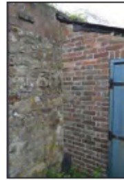
7494-0035 Combers Glasshouses - Building 4 - straight joint intersection of building and wall. Facing south-west
