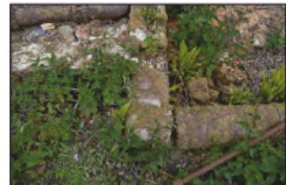
7494-0027 Combers Glasshouses - Building 2 - straight joint intersection of bed and building. Facing north
