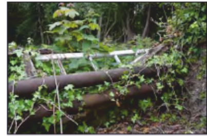
7494-0078 Combers Glasshouses - Building 1 - top- heating pipes and in-situ window in south lean-to. Facing south
