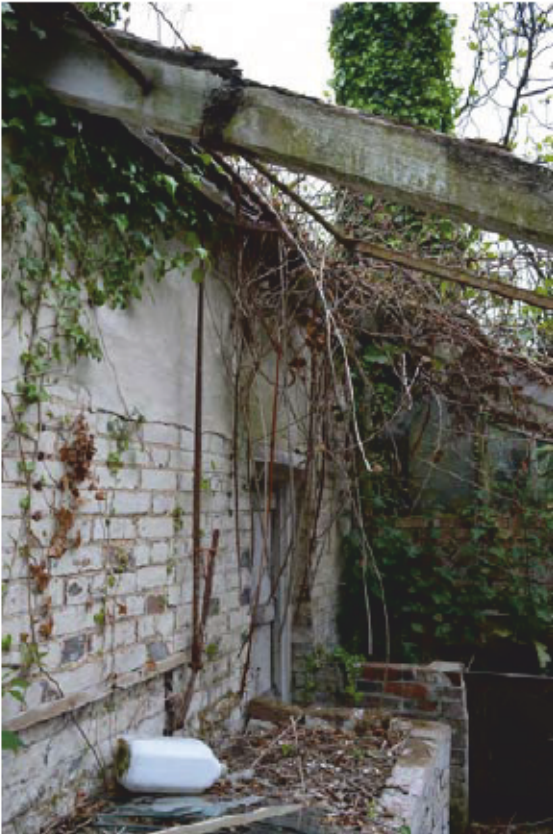
Plate 9: Southern lean-to, Building 1, lever tackle and roof construction. Note void mortise for timber purlin. Looking east (Photo #72)
