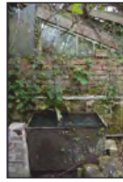
7494-0077 Combers Glasshouses - Building 1 - water vatt in east of south lean-to. Facing east
