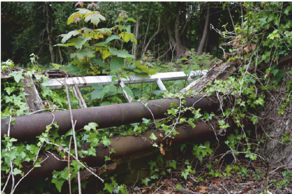
Plate 8: Southern lean-to, Building 1, extant window framing on south wall. Note the top-heating pipes. Looking south (Photo #78)
