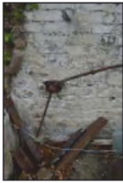
7494-0016 Combers Glasshouses - Building 2 - Bay 2, screw operated window opening. Facing north
