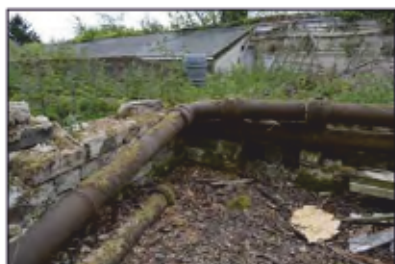
7494-0013 Combers Glasshouses - Building 2 - Bay 1, heating pipes. Facing south-east
