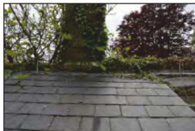
7494-0044 Combers Glasshouses - Building 4 - Slate roof, kitchen garden wall coping, and chimney stack. Facing south
