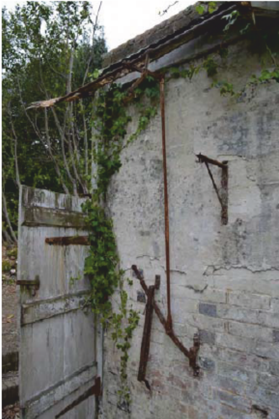
Plate 5: Southern lean-to, Building 1, door to west and lever tackle, looking west (Photo #66)
