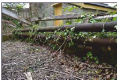
7494-0070 Combers Glasshouses - Building 1 - Top- heating pipes in east of south lean-to. Facing south-east
