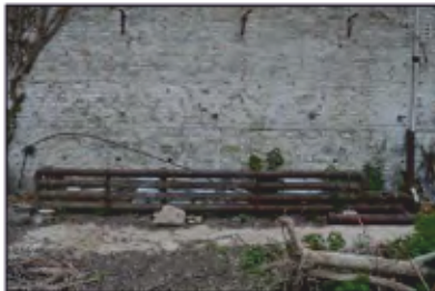
7494-0019 Combers Glasshouses - Building 2 - Bay 2 pipework. Facing north
