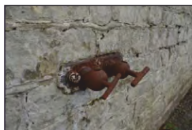
7494-0012 Combers Glasshouses - Building 2 - Bay 1, screw operated window opening. Facing east
