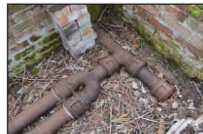
7494-0069 Combers Glasshouses - Building 1 - pipework in south lean-to. Facing south
