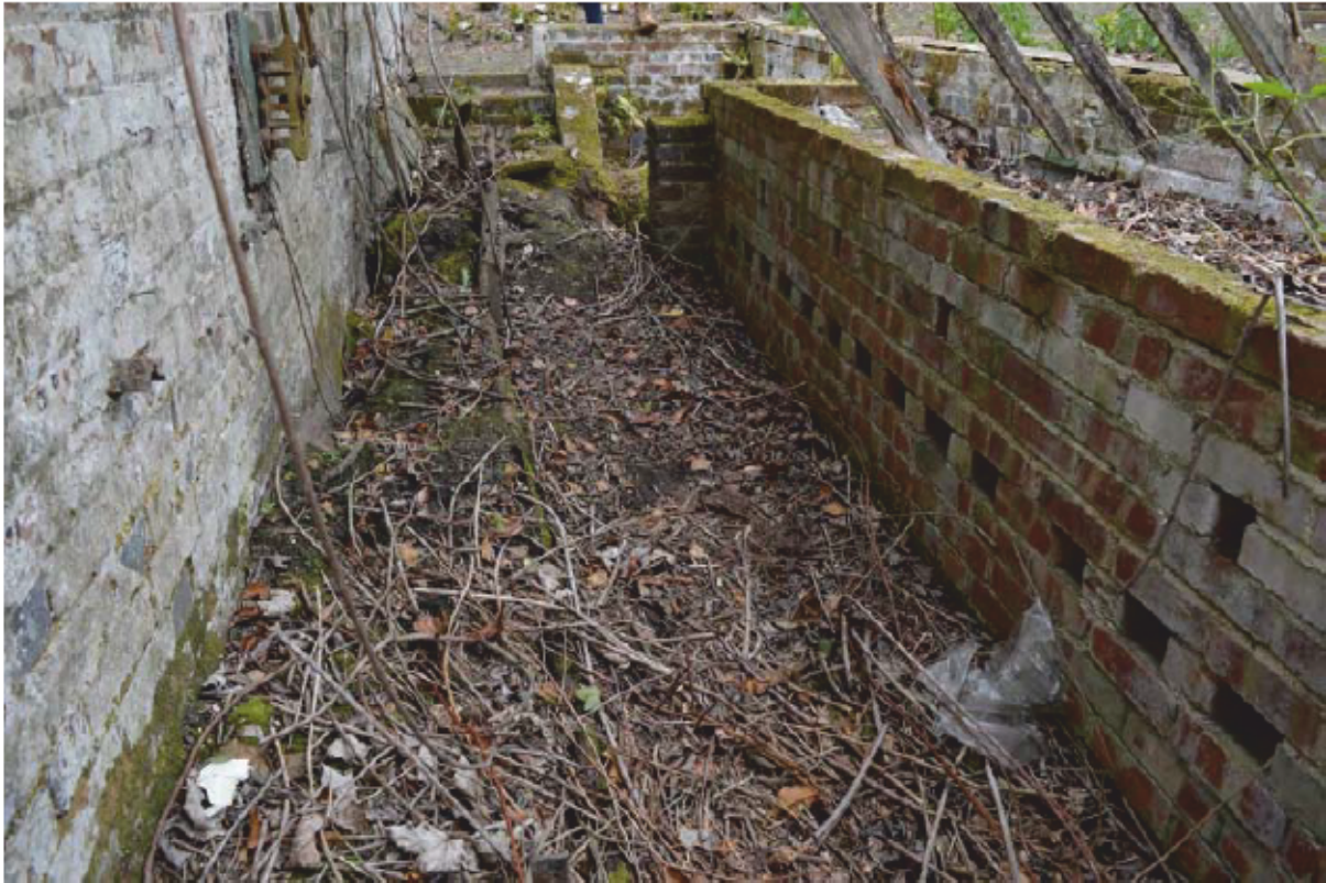
Plate 15: Northern lean-to, Building 1, interior overview. Note metal bed to south and possible brackets above. Also note ventilation and drainage holes in the northern bed. Looking west (Photo #57)
