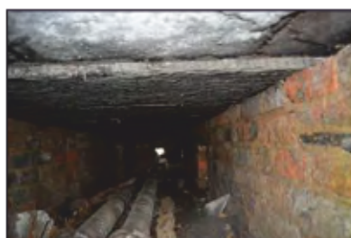
7494-0074 Combers Glasshouses - Building 1 - Pipework beneath forcing bed in south lean-to. Facing west
